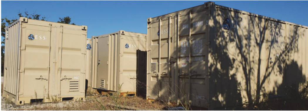
Figure 20. Flow battery system at CBITEC.
