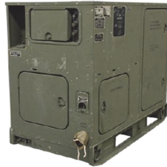
Figure 18. 60 kW AMMPS generator.
