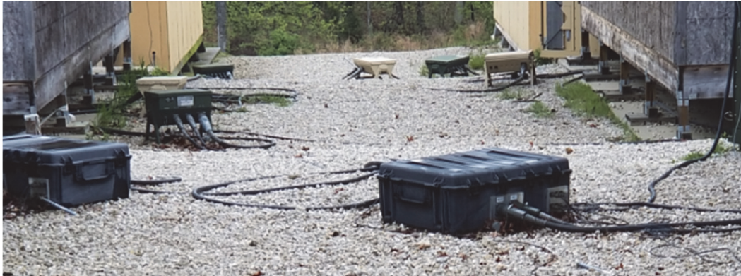
Figure 22. PDISE equipment at CBITEC.
