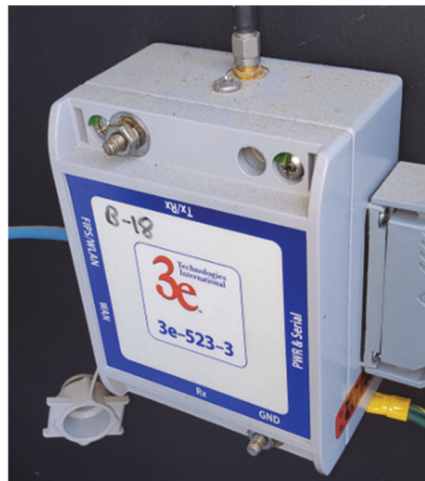
Figure 107. DMMA wireless access point.
