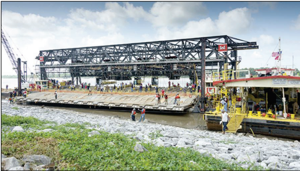
Figure 8. View of the current MSU from landside prior to anchoring of mats for placement.
