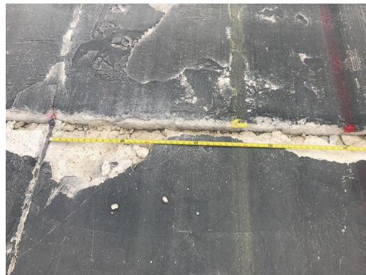
(f) Spalling in Quadrant #3 at 896 passes
