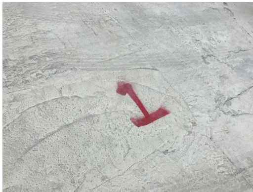
(a) Shrinkage cracks at 0 passes
