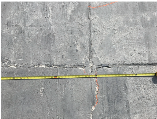
(c) Small corner break in center of repair at 112 passes
