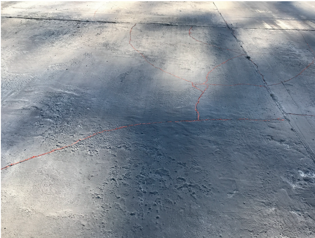
Figure 54. Low-severity shattered slab at 448 passes.
