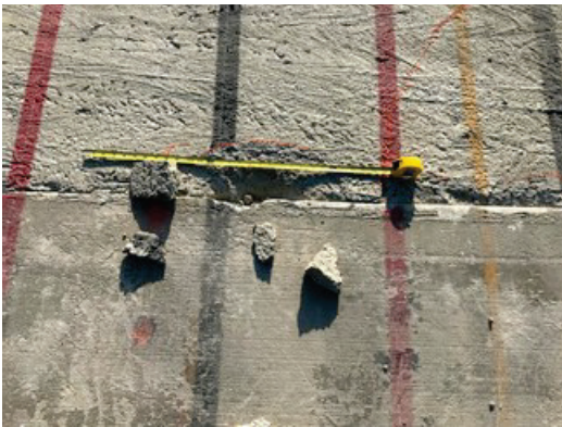
(c) FOD and spall on the western edge at 112 passes
