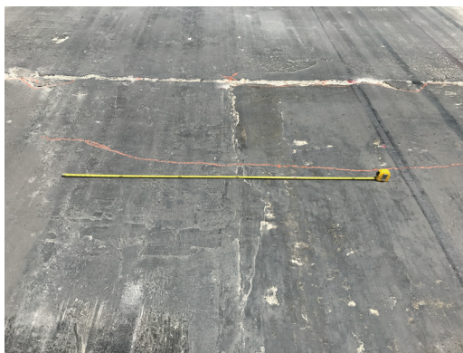
(e) Crack from Quadrant #1 to #3 at 768 passes
