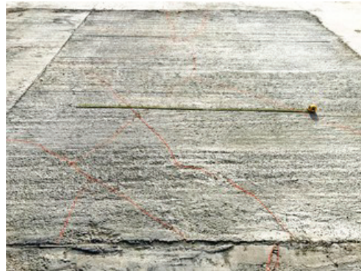
(b) Low severity shattered slab at 112 passes
