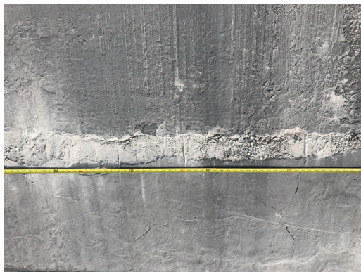
(e) Spalling in Quadrant #3 at 784 passes
