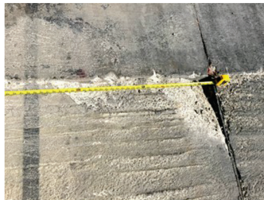
(f) Spall on the eastern edge causing failure at 224 passes.
