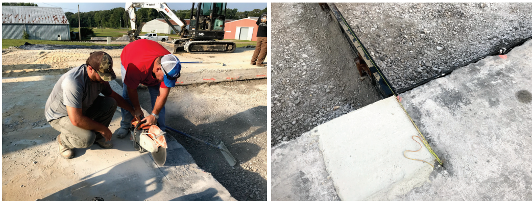
Figure 34. Patching high-severity joint spalls on the parent slabs adjacent to the repair area.
