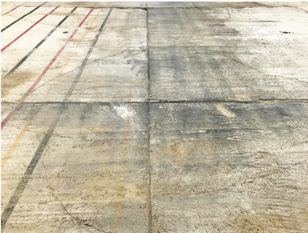
Figure 42. Cracking in the center of Repair 2 at 224 passes.
