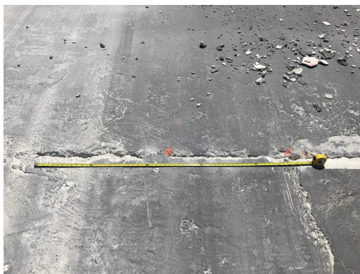
(c) Spalling at joint on Quadrant #1 at 224 passes
