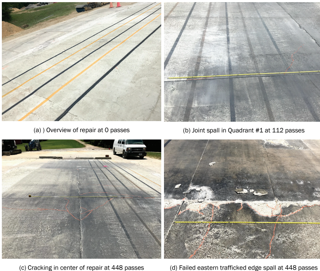
Figure 43. Repair 3 progression of distresses.
