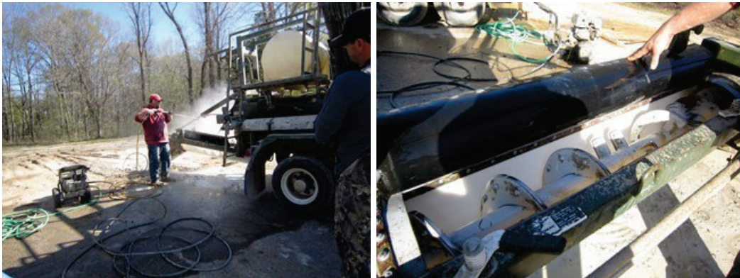
Figure 33. Washout of volumetric mixer using a pressure washer (left) and the resulting clean auger (right).
