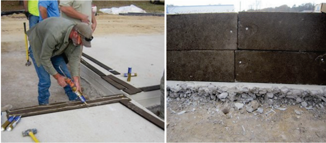
Figure 21. Installation of expansion board that included a combination of applying Liquid Nails and masonry nails in the curing rapid-setting concrete (Repair 1).
