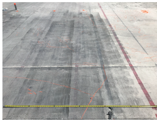
(b) Cracking in the paste at 112 passes
