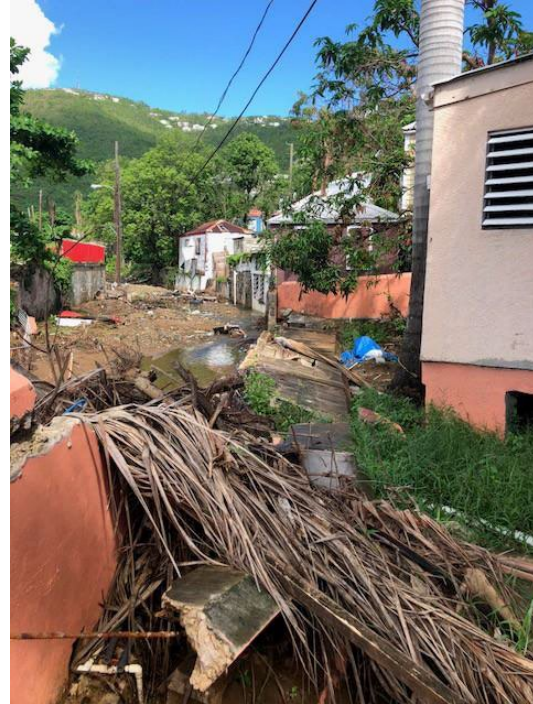
Figure 10. Collapsed channel wall. (SOURCE: Corps staff, October 2017)
