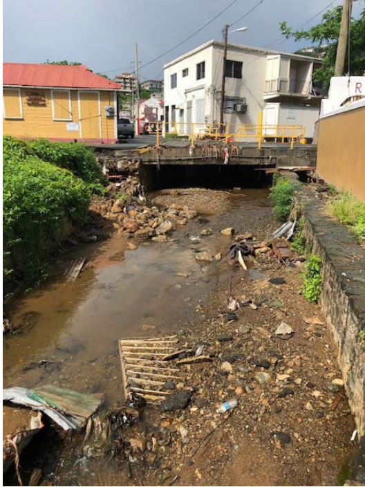
Figure 7. Sediment build up in the channel. (SOURCE: Corps staff, October 2017)
