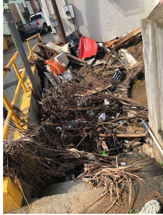
Figure 9. Debris accumulation in the channel. (SOURCE: Corps staff, October 2017)
