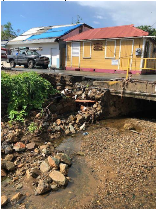
Figure 8. Channel wall damage and erosion. (SOURCE: Corps staff, October 2017)
