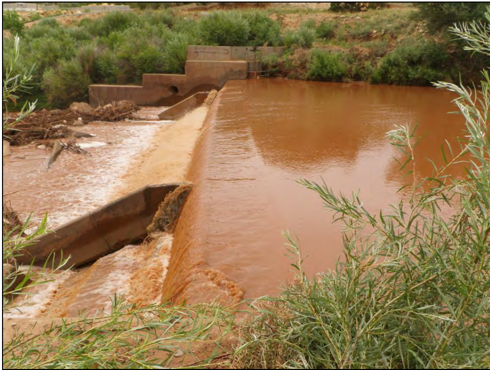
Photograph No. 59: View to the south of the leaning Villanueva Diversion Structure. July 15, 2014.
