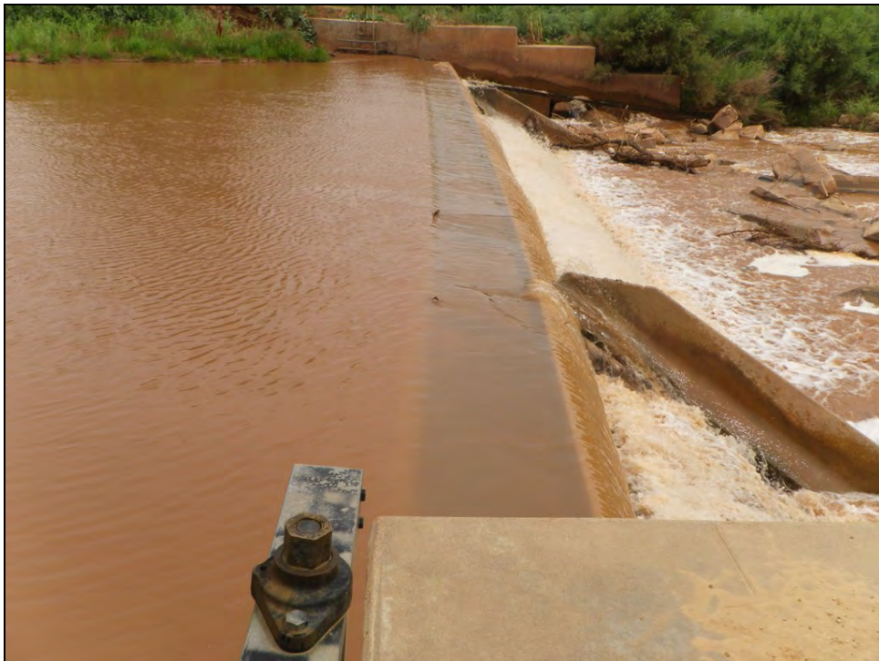
Photograph No. 23: View to the north of the leaning Villanueva Diversion Structure. July 15, 2014.
