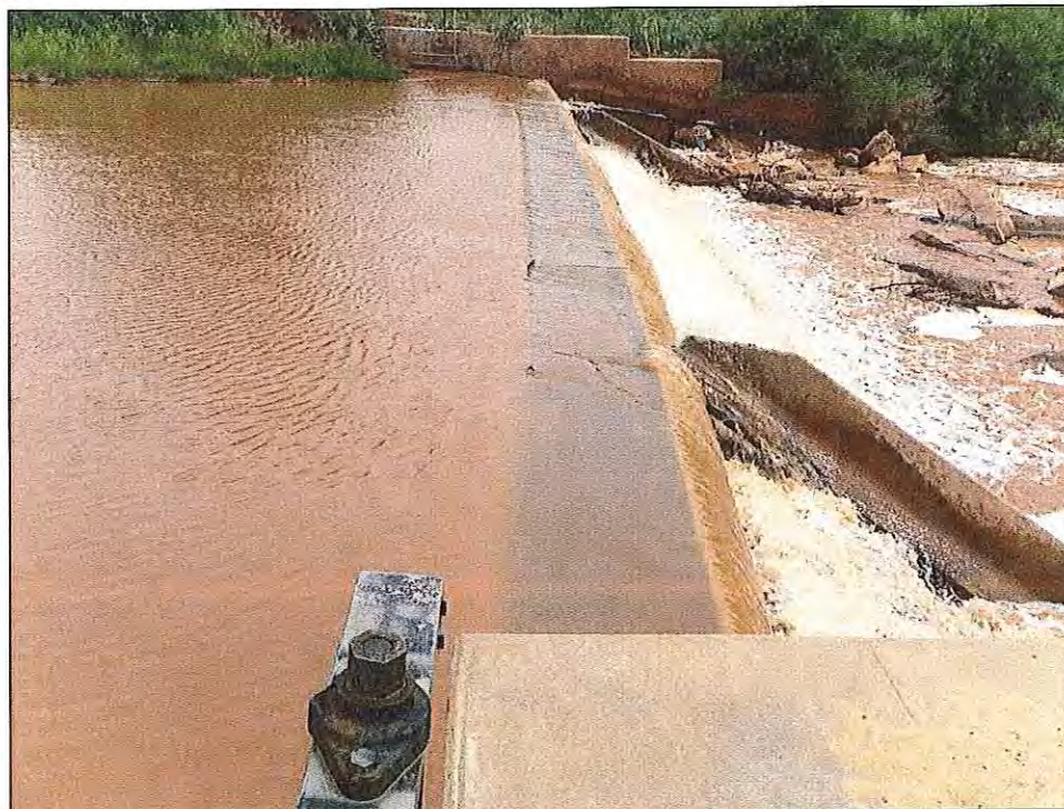
Photograph No. 23: View to the north of the leaning Villanueva Diversion Structure. July 15, 2014.
