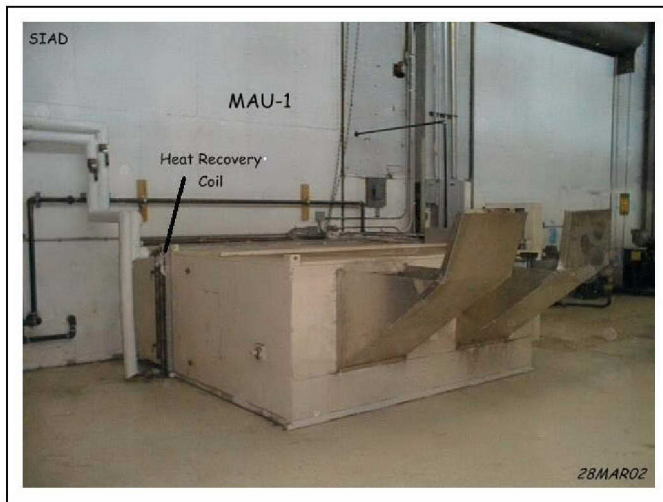
Figure 18. MAU-1 heat recovery coil.
