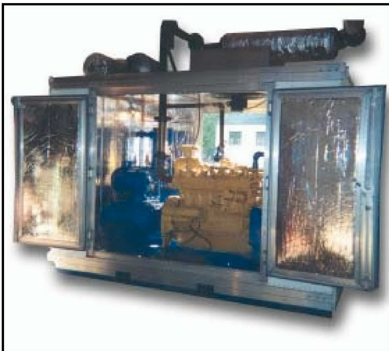
Figure 1. Dearing Ultra Air Model GSR-125LA NGEDAC installed at Picatinny Arsenal
