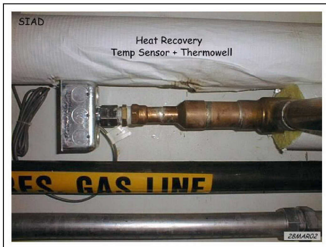
Figure 19. Heat recovery temperature sensor/thermowell.
