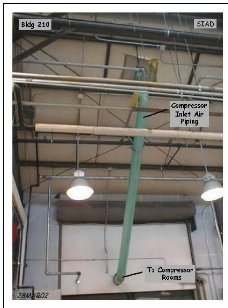
Figure 14. Compressor intake air duct—inside Bldg 210.
