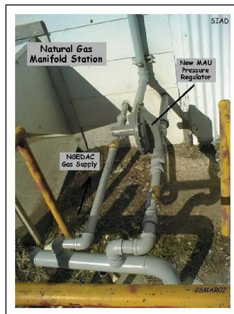
Figure 11. Natural gas manifold station.
