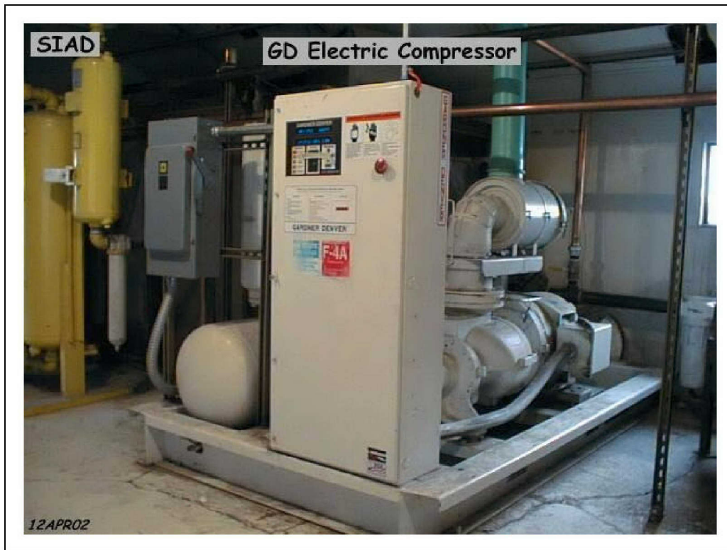
Figure 25. Backup electric compressor.
