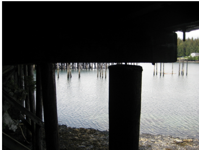
Figure D-2. Gap between pile and dock
