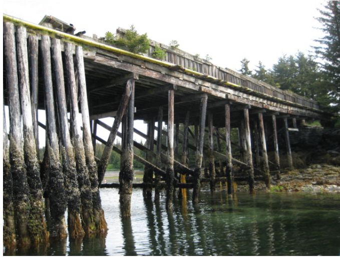
Figure D-7. View showing misaligned pile under causeway
