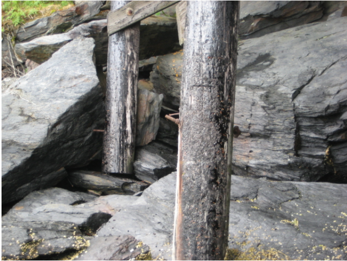
Figure D-4. Unbraced piles on bedrock with bolts indicating missing bracing
