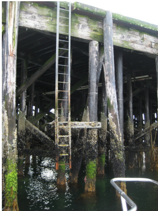
Figure D-6. Dangling ladder missing supports due to decay of bracing
