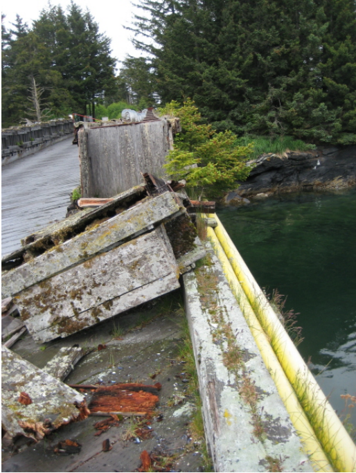
Figure D-12. Decaying live crab pots, fuel lines, and vegetative growth including trees
