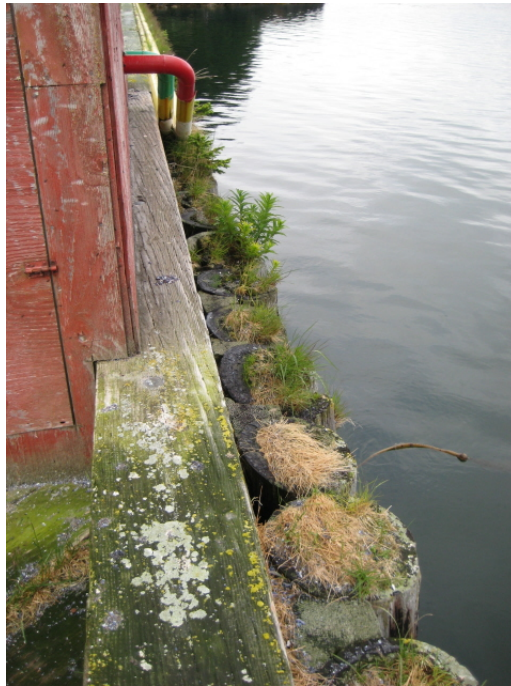
Figure D-1. Vegetation growing atop pile ends
