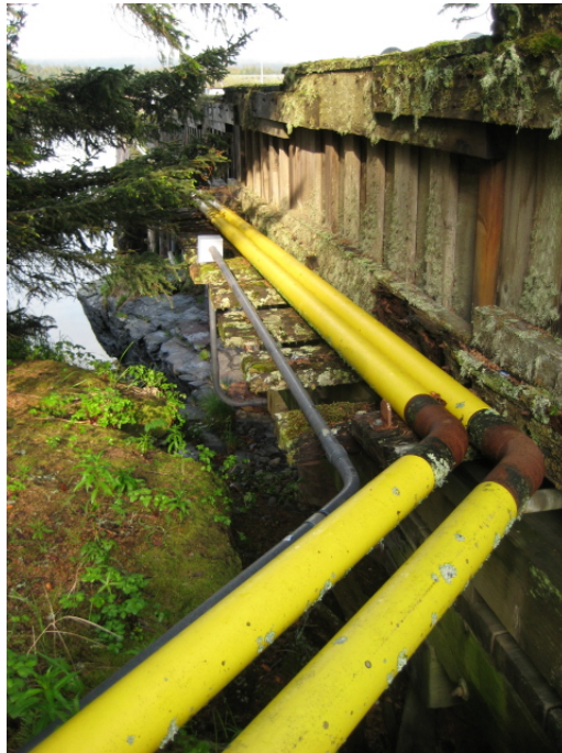
Figure D-10. Fuel lines on edge of dock
