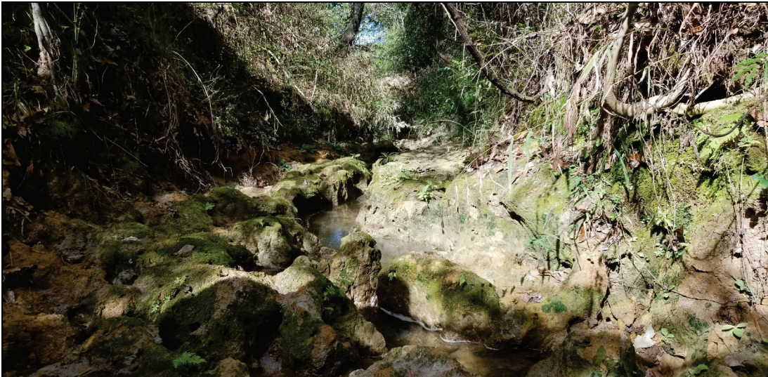
Figure 10. Campbell Creek Tributary nick zone downstream of James H. Bidy Road culverts.
