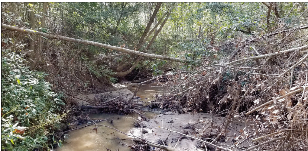
Figure 8. Campbell Creek field identified bed degradation with sloughing bank and vegetation.
