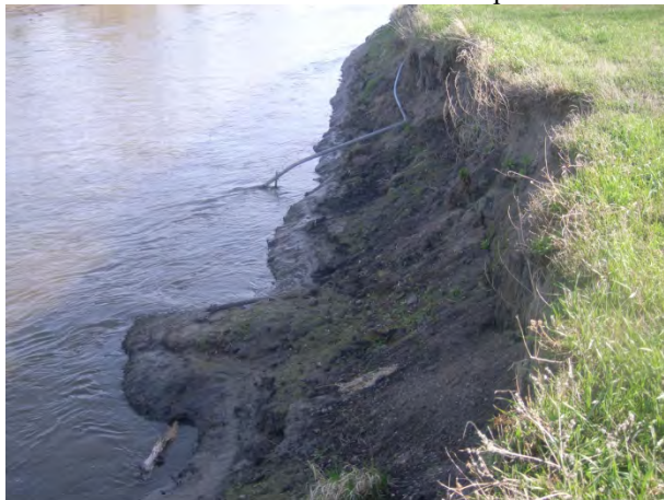
Figure 4. Chippewa River Diversion approach channel east bank – middle reach with pipeline connecting to the USGS gage station (4 April 2012).
