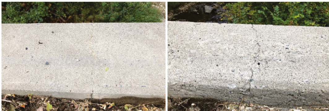
Figure 2. Representative photos showing the conditions of the CWAS (left) and conventional (right) bridge curb repairs detailed in Fig. 1, circa September 2018. The repair performed using CWAS exhibits superior surface quality as well as less extensive cracking after 16 years of exposure to winter freeze-thaw cycling and road-deicing salts.
