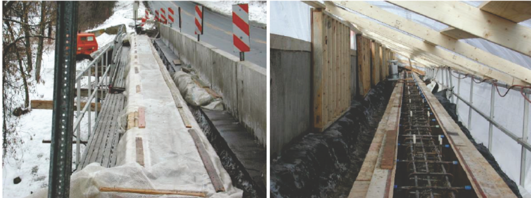
Figure 1. Bridge curb repairs performed in the winter of 2002, on the west and east sides of the Trues Brook Bridge in Lebanon, NH. The west side (left) of the bridge was repaired using CWAS concrete, while the east side (right) was repaired using conventional concrete in a heated enclosure.
