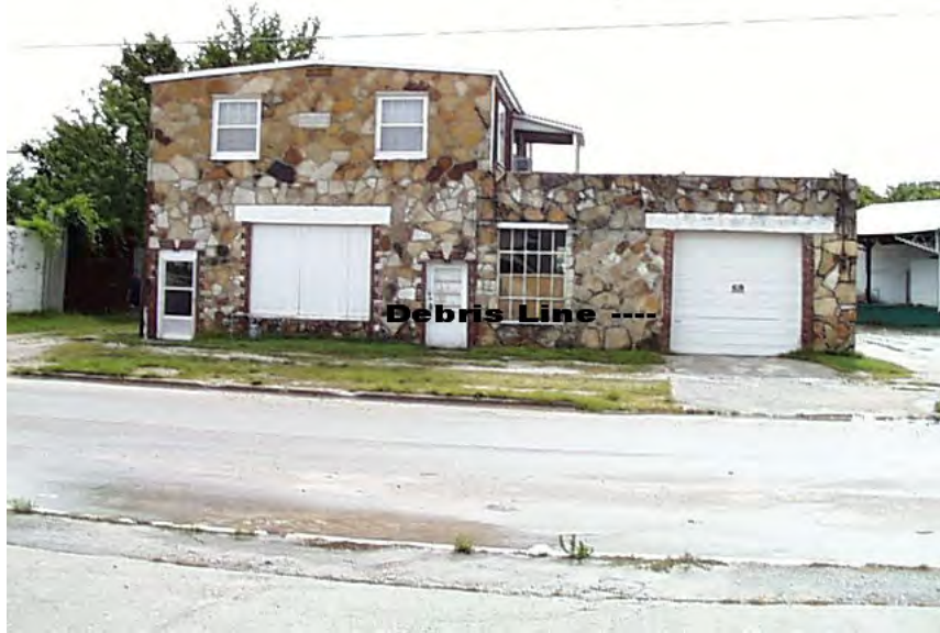
Lower Branch of Jordan Creek. 210 N Nettleton Avenue (Lower Branch RS 9211). The debris line on the garage door measures 34-inches from the floor. The FFE of the building is 1248.14, giving a WSE of 1250.97. This photo was taken after flood waters receded on July 12, 2000. See Appendix F for WSE comparison.
