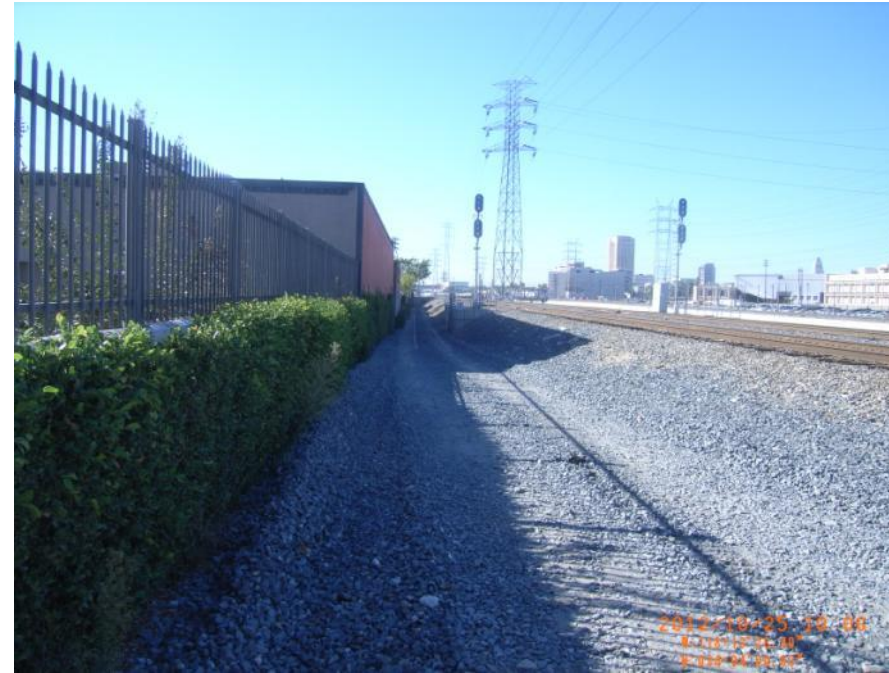
Photo 3: View looking downstream at N. Main Street. LAR 5 on right side. Not a levee condition. Ground in immediate foreground at approximately the same elevation of the wall depicted in Photo 2.
