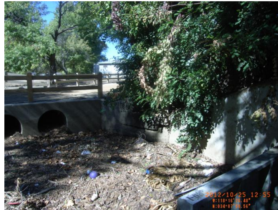
Photo 9: Landside of tunnel looking upstream. Wall in foreground is the wall depicted in Photo 8. The building in background is at approximately same grade as top of tunnel.
