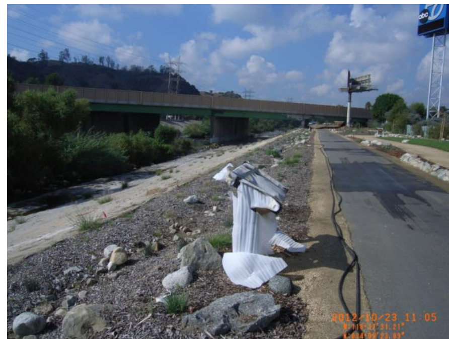
Photo 16: Looking upstream on LAR 7. Levee condition and irrigation lines at riverside crest and across entire landside slope. I-5 in background.
