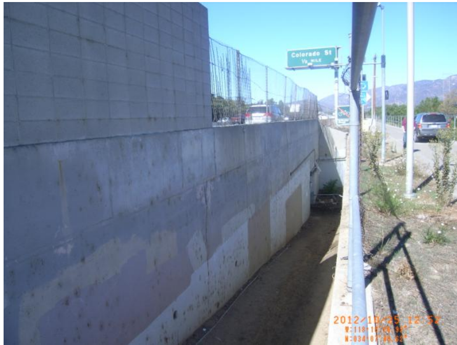
Photo 7: Equestrian ramp and tunnel entrance. Note crest on right, highway on left. Tunnel and culvert at base of down-ramp in center.
