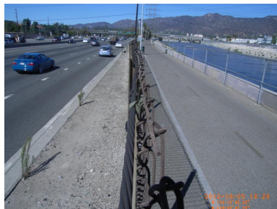
Photo 10: Looking upstream on LAR 3 near Gene Autry Museum. Levee condition of approximately 2 to 4-feet exists and flow would be directed on I-5 and along levee. Southbound lanes are higher than northbound lanes.
