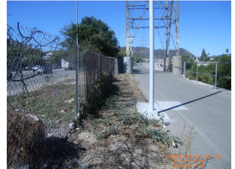
Photo 5: On crest of LAR 3 looking upstream. Not a levee condition. Although landside is slightly lower than crest. Flow would be directed along I-5 (on left) and the crest of the highway is above the crest of LAR 3.
