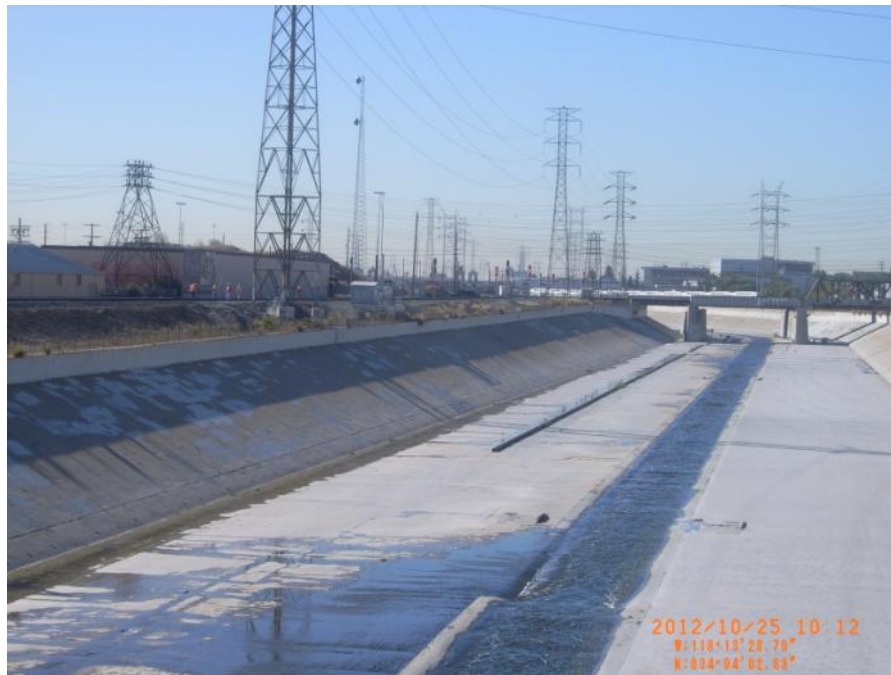
Photo 2: View looking downstream at N. Main Street. LAR 5 on left side. Not a levee condition. Railroad embankment with ascending slope above top of wall. Photo 3 depicts landside condition further.
