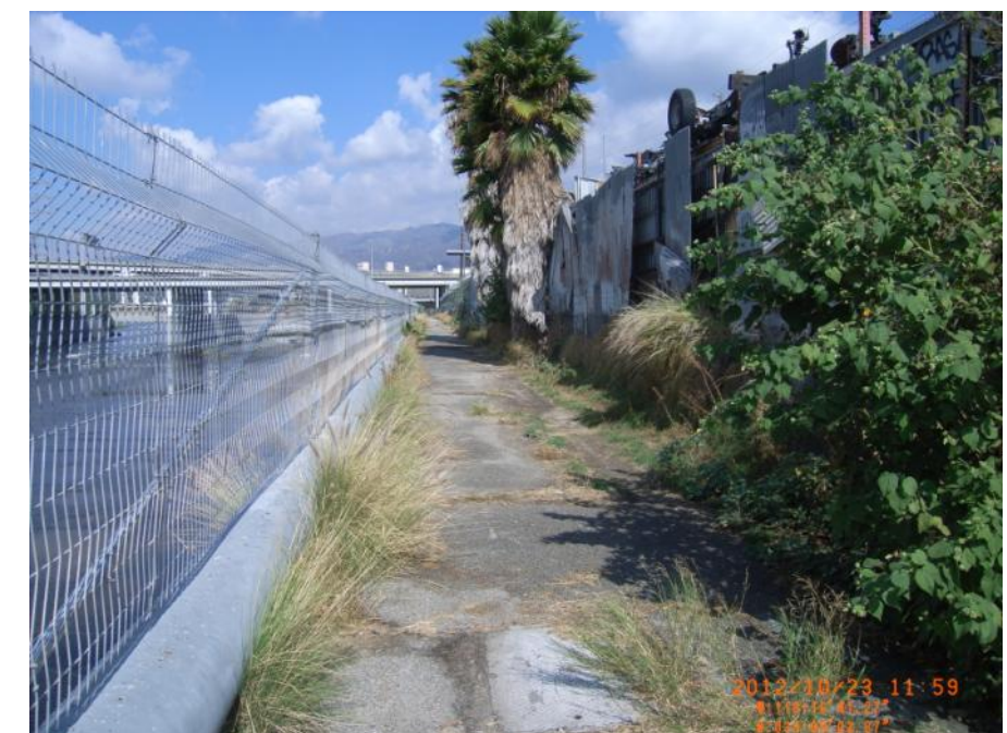
Photo 18: Looking upstream on LAR 6. Vegetation on levee and cannot inspect toe with fence.
