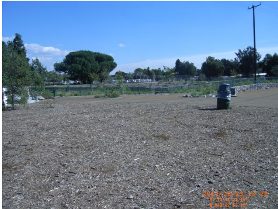
Photo 19: Atwater Park. Not a levee condition on LAR 6 but needed as levee conditions exist upstream and downstream.
