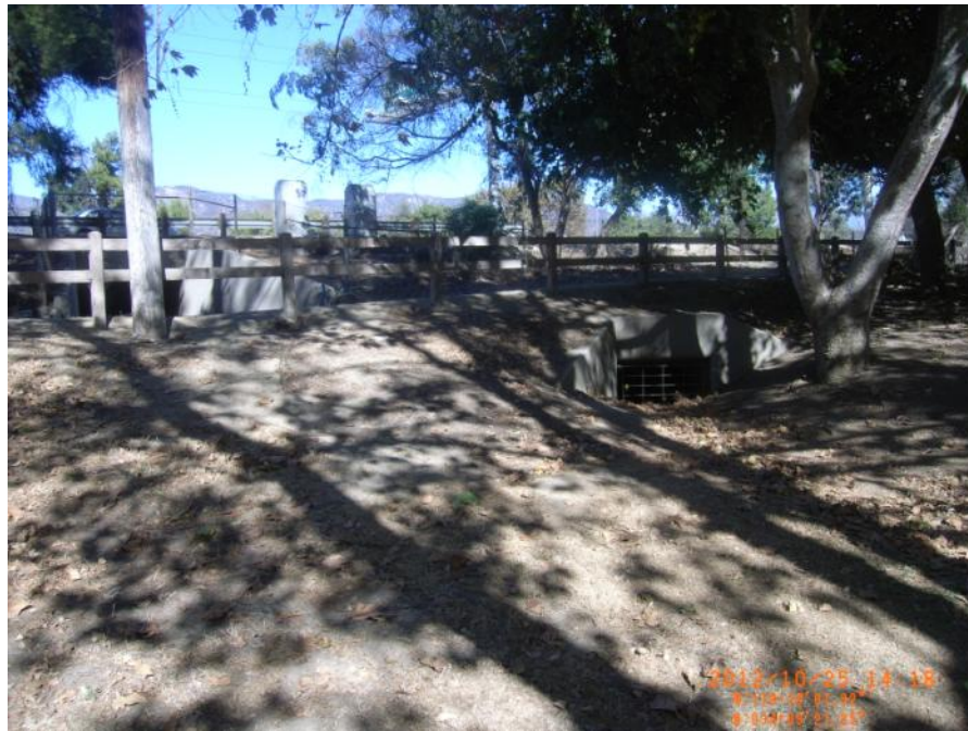
Photo 13: Landside of undercrossing on left side. Inlet of drain on right side.
