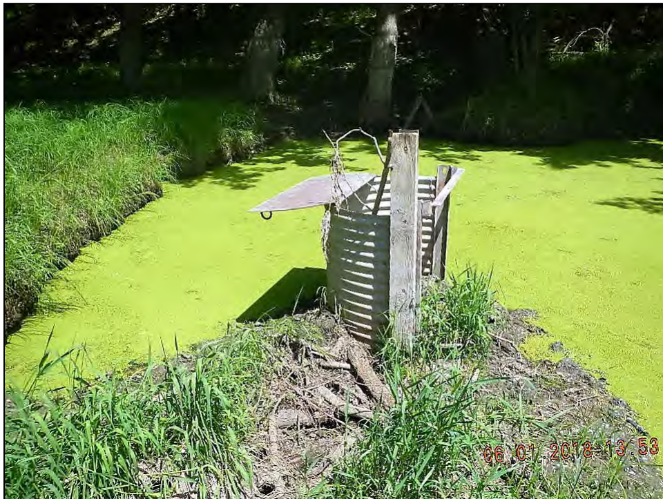
Figure 6. General view of silted stoplog structure
