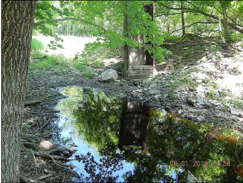
Figure 7. Abandoned and unmaintained stoplog structure
