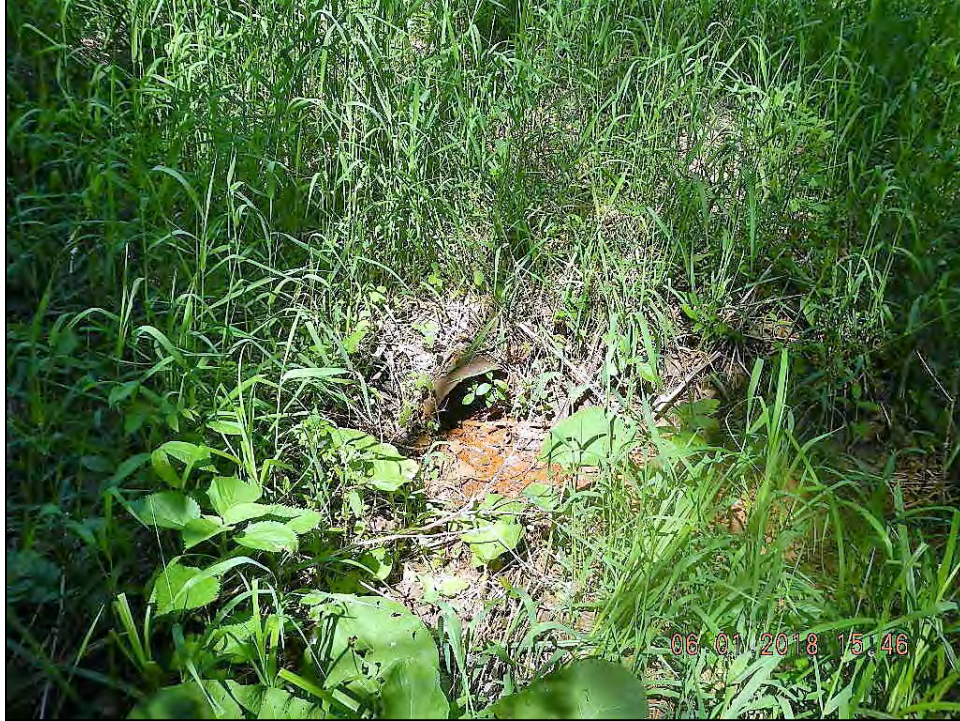
Figure 31. Obscured inlet of iron pipe
