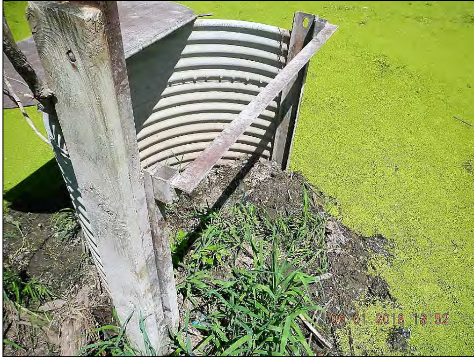
Figure 5. Silted in stoplog structure
