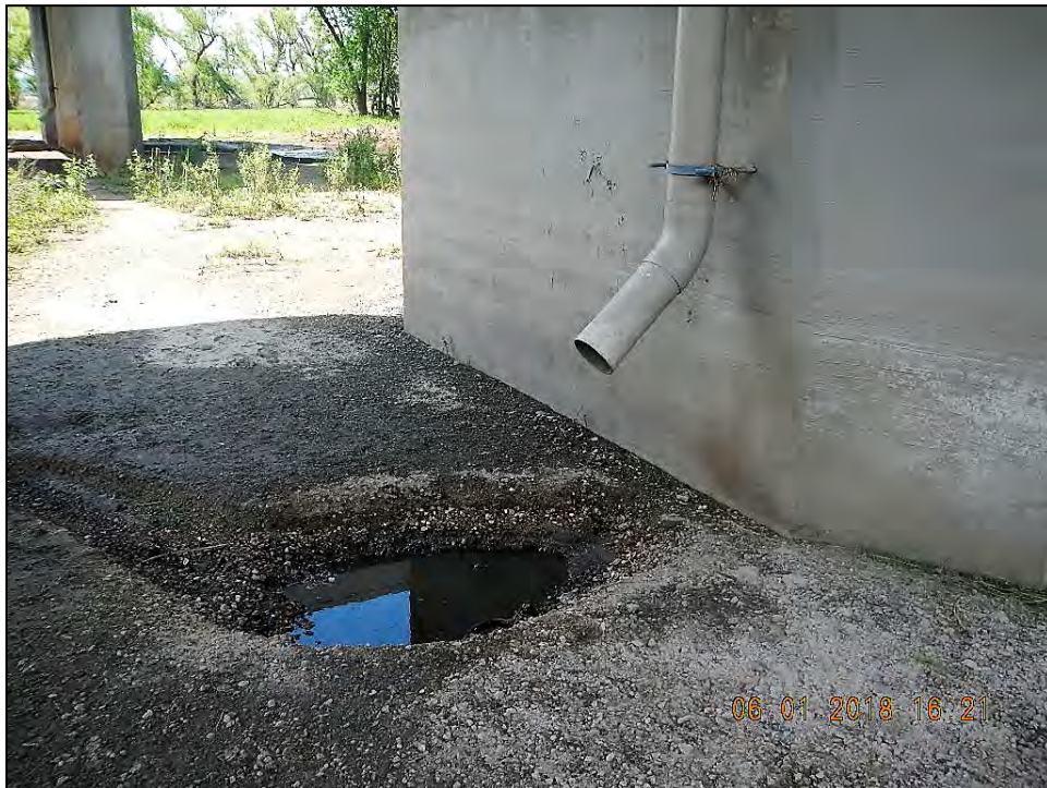
Figure 44. US Highway 169 roadway drainage discharge pipe scour
