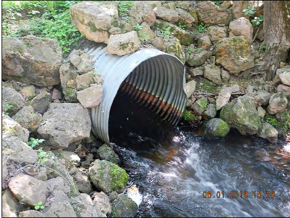
Figure 23. Discharge end of 72-inch corrugated metal pipe
