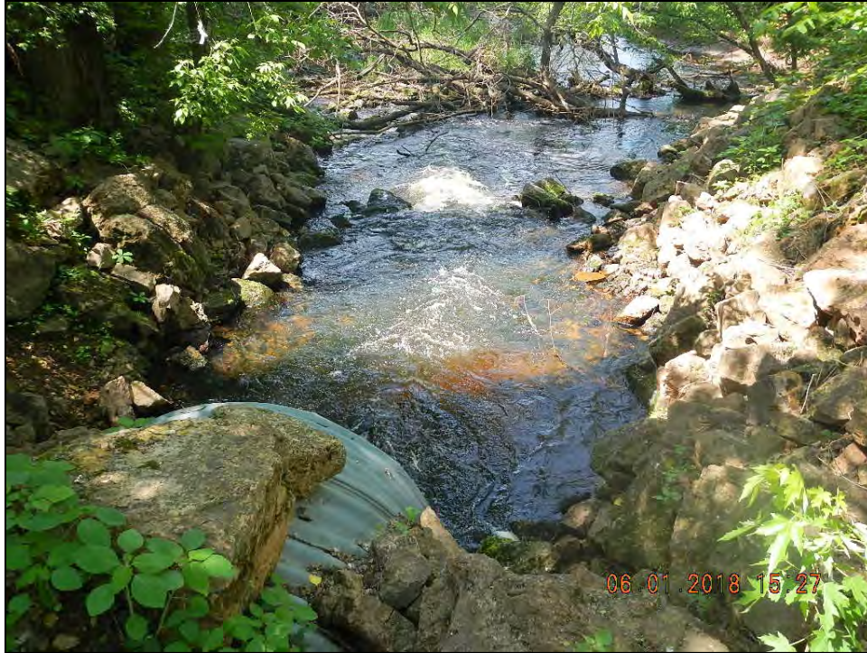
Figure 21. Corrugated metal pipe conveying primary Blue Lake Watershed channel
