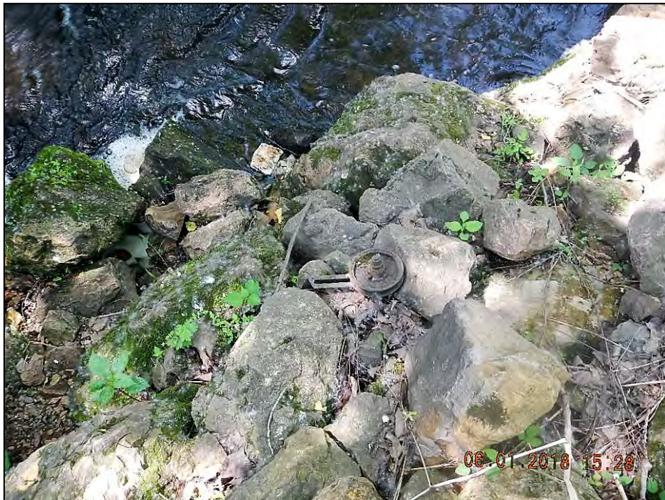
Figure 22. Miscellaneous metal scrap on culvert discharge riprap
