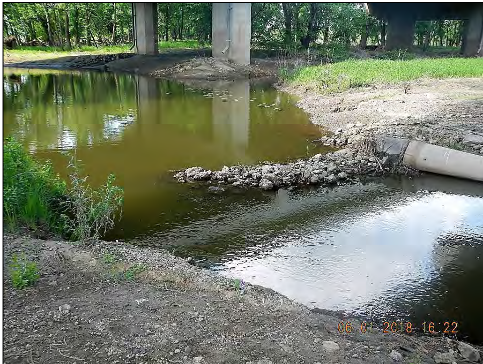
Figure 46. Upstream end of scour around reinforced concrete pipe culvert
