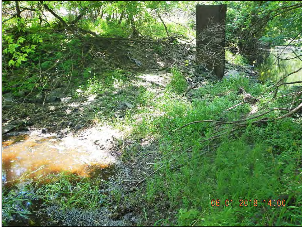
Figure 11. Outlet/discharge area of abandoned stoplog structure
