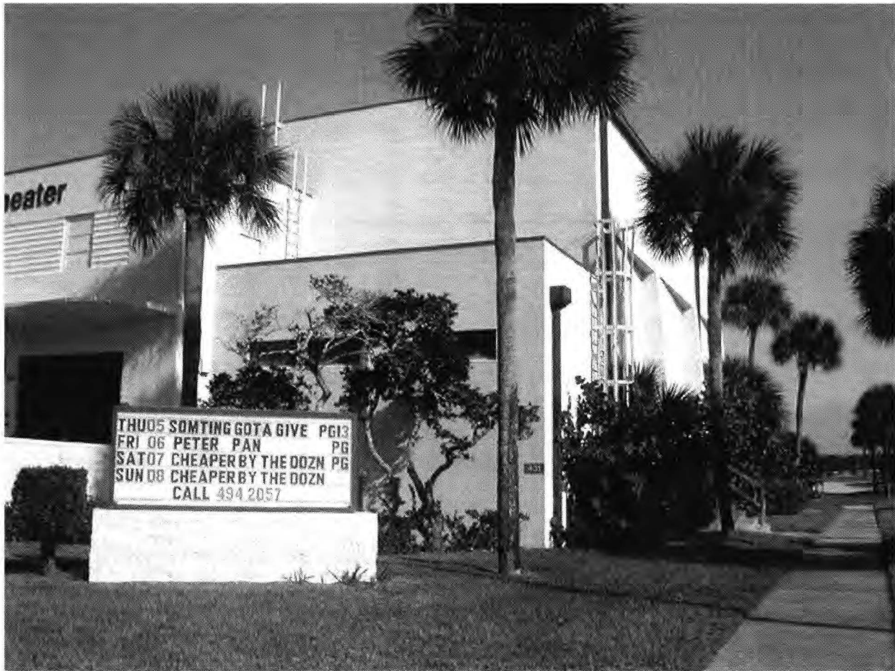
Figure 7. Multiple Ladders to Rooftops.
