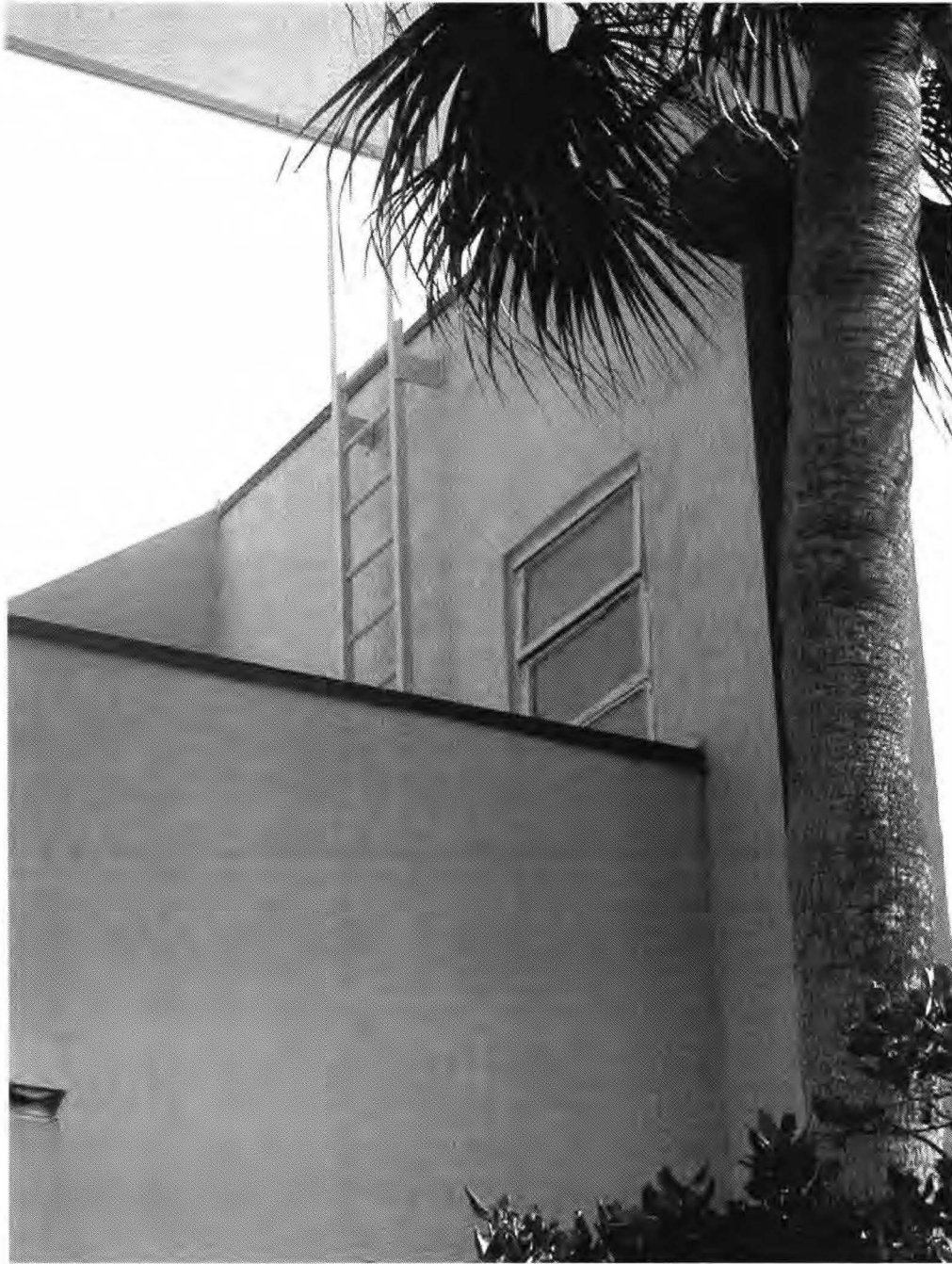
Figure 12. Original Projection Room Awning Window.
