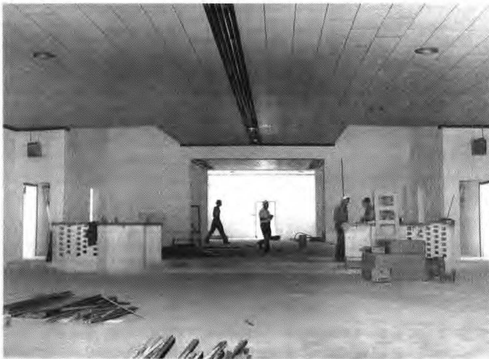
Figure 4. Progress Shots of Chapel at NAS Banana River, Florida, Interior Looking Toward the Front of Chapel, 20 August 1945. (NARA, RG 80-G Box 1281 339538).
