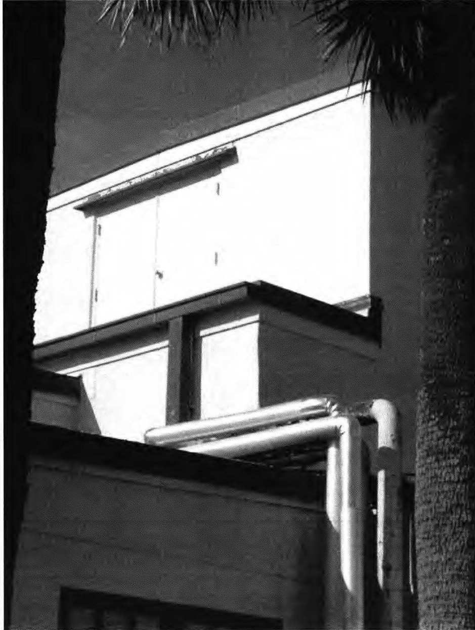
Figure 21. Hot Water Heating Pipes, Duct Enclosures, and Mechanical Penthouse.
