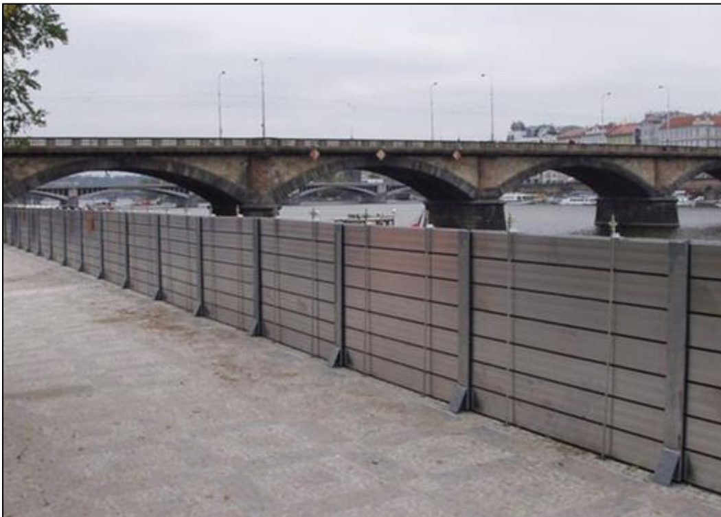
Figure 9. Demountable floodwall system.
