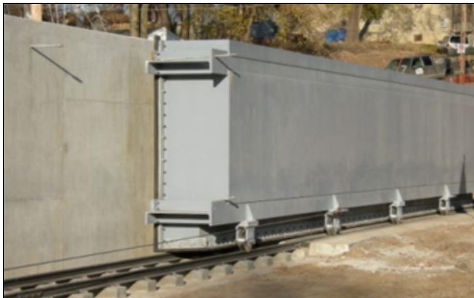
Figure 12. Rolling gate (photo: MVR).
