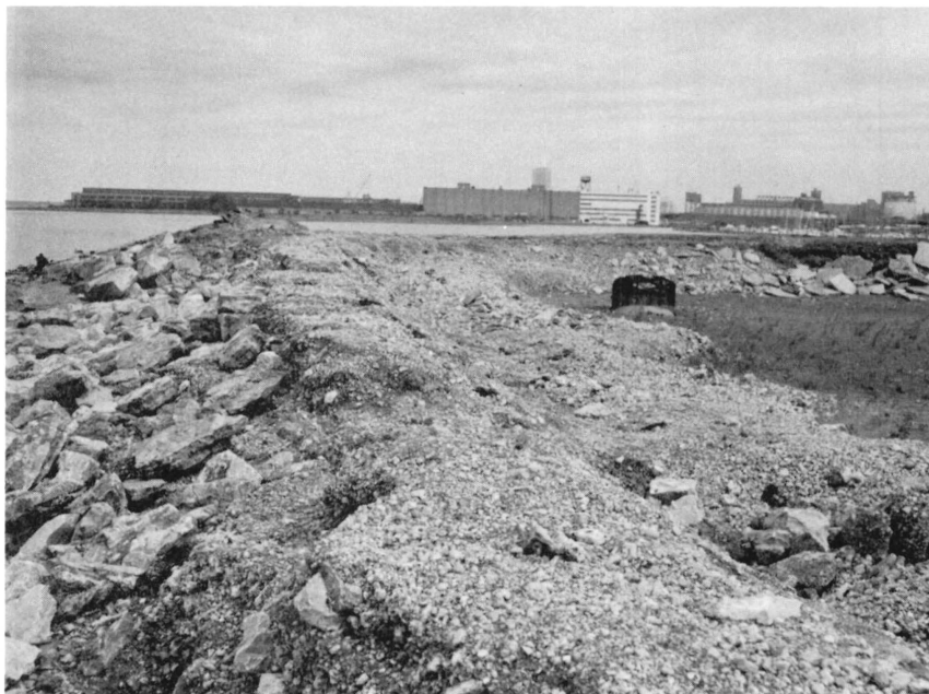
Fig. 44. Storm damage--displacement and loss of stone protection on retaining dike, Buffalo Harbor facility No. 1 (Buffalo District)
