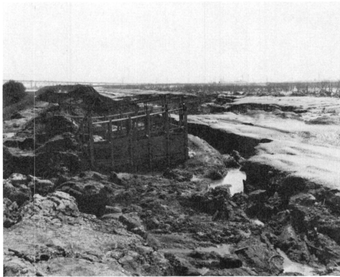
b. Sluice structure which settled 9 ft and moved horizontally outward a distance of 6 ft
