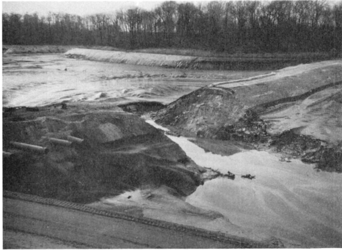
a. A 60-ft-wide break in the 30-ft-high cross dike
