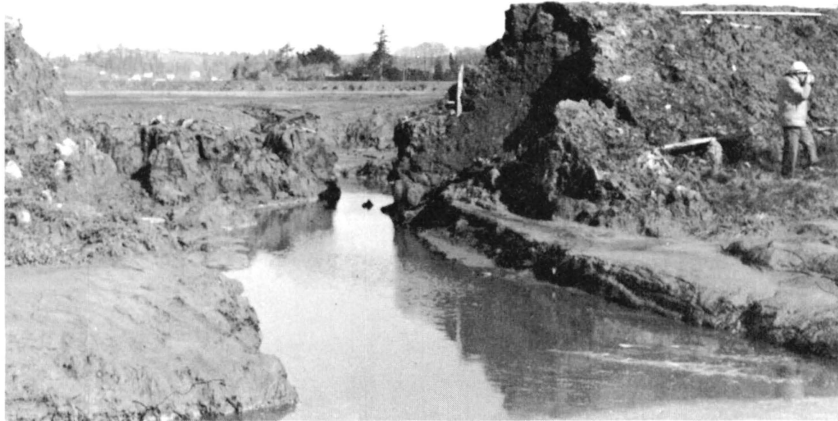
a. Washout at sluice structure
