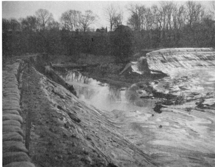
b. A 50-ft-wide break in the 21-ft-high dike surrounding the adjacent lower area
