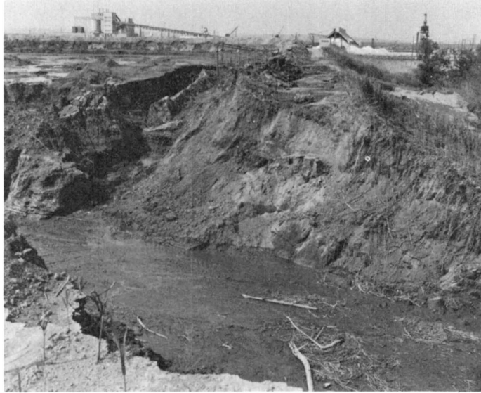
a. A 50-ft-wide break in the 25-ft-high dike section
