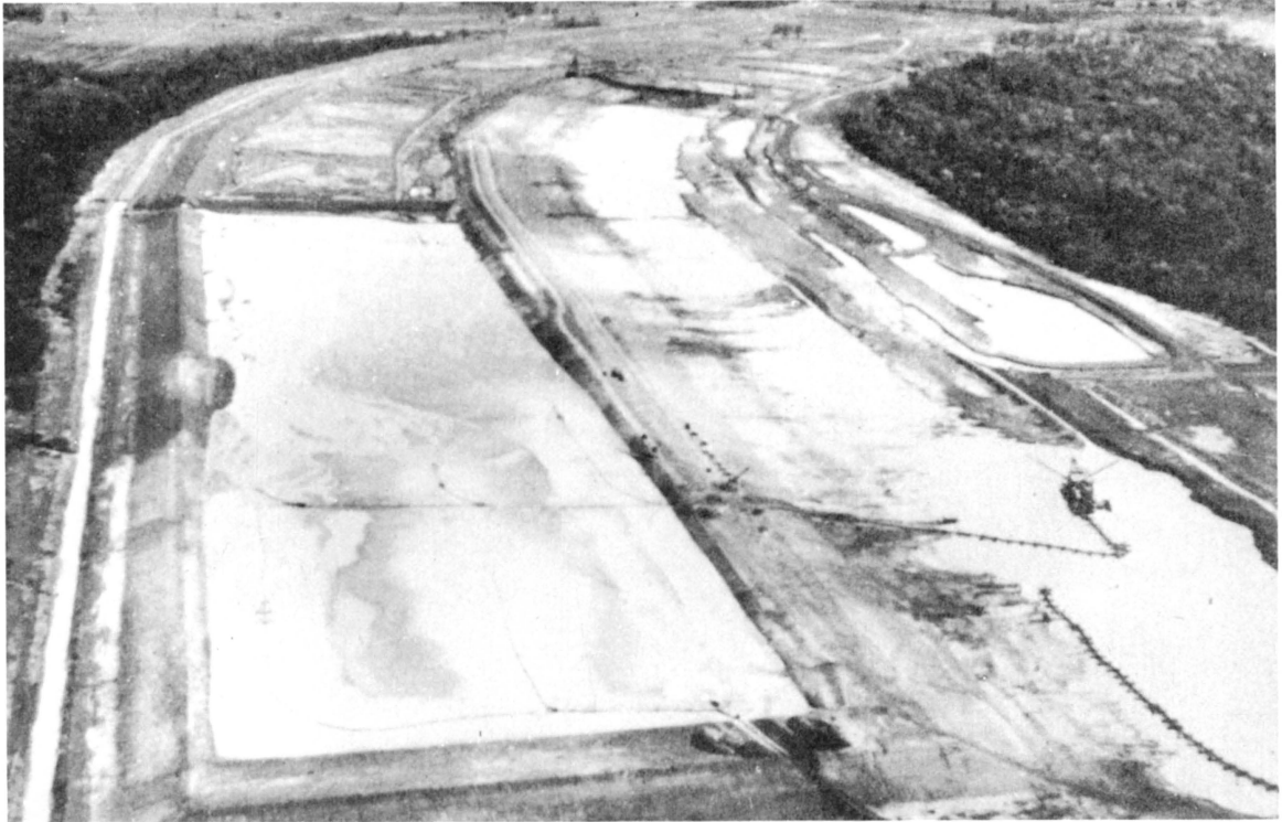
Fig. 6. View of Vicksburg Harbor industrial fill under construction. Hydraulic filling in progress (Vicksburg District)
