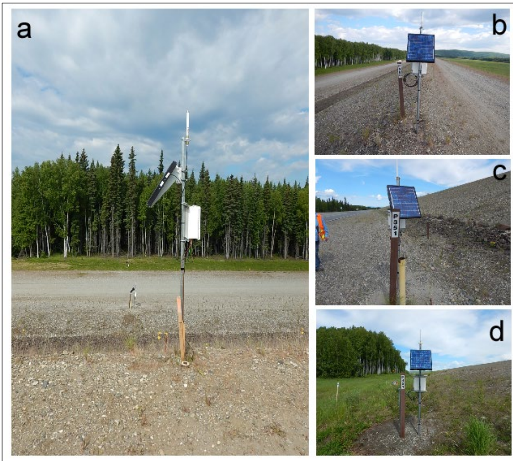
Figure 17. View of a cross-section with three piezometers (a), with a station at the crest of the embankment (b), the toe of the embankment (c), and at the toe of the stability berm (d).
