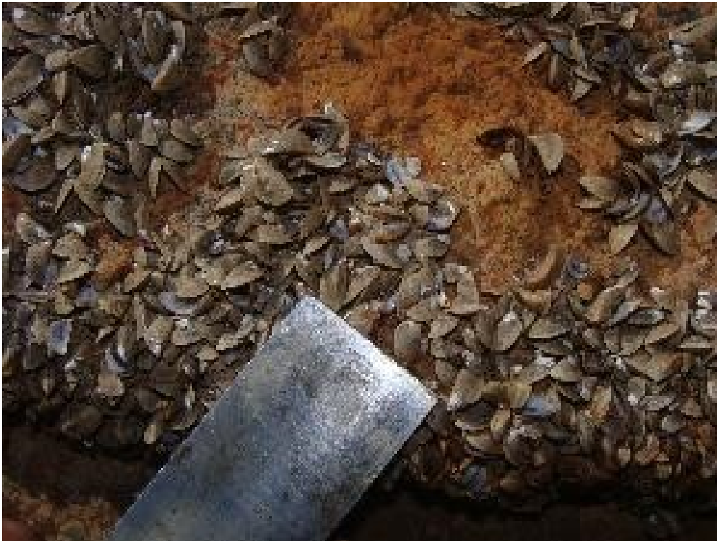
Figure 2. Zebra Mussels on emergency bulkheads at Emsworth Lock & Dam, Pittsburgh District 2016.
