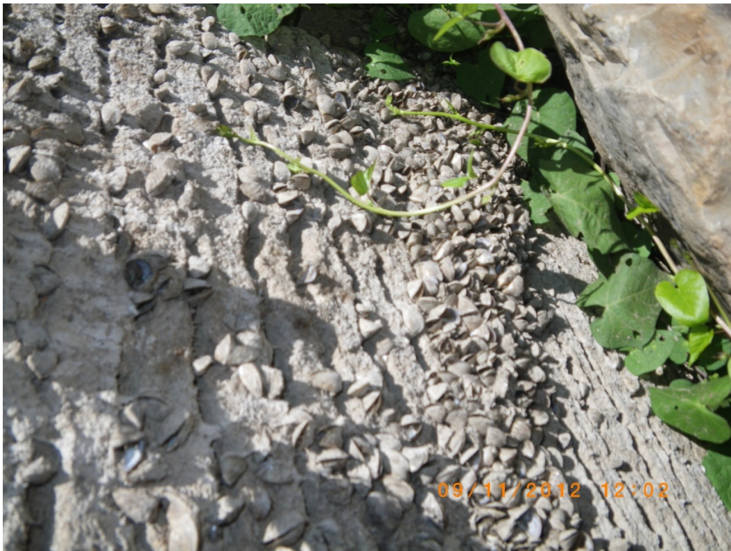
Figure B-3. ZM attached to ACM (articulated concrete mat), September 2012, Memphis District.
