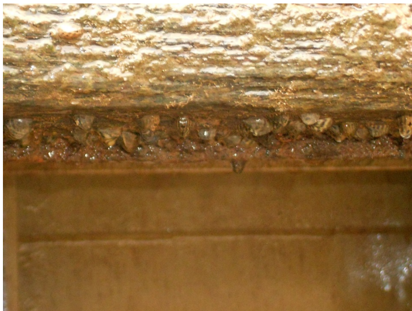
Figure B-2. ZM on concrete wall in lock chamber of #3 Lock & Dam on Red River, April 2017, Vicksburg District.
