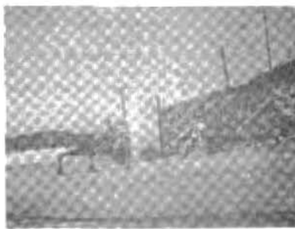
Eroded terrain behind sea wall at Station 12, May 2, 1942.
