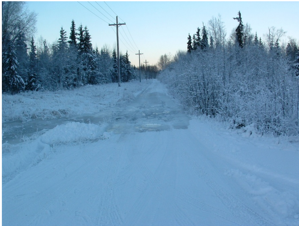
Figure 6. Flooding across the Fort Richardson Fish Hatchery Access Road. (Image by Andrea Tesch.)
