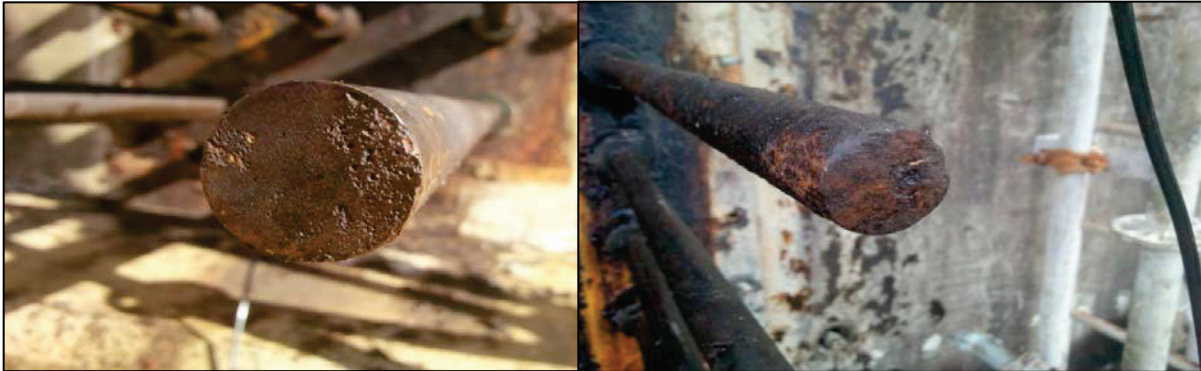
Figure 4. Pitted rod and surface corrosion on rod.
