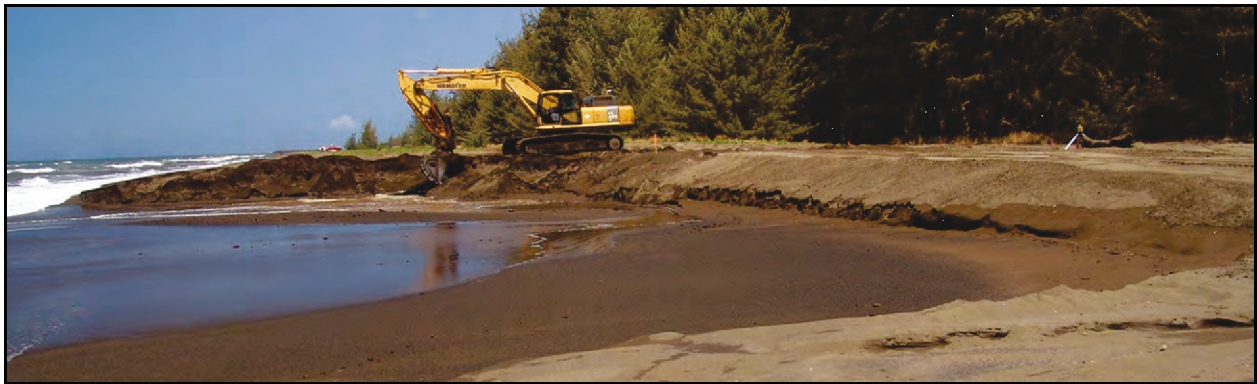
Figure 5. Excavation of the subaerial beach profile at Waimea Cottages during the first increment of the 2014 sand bypass operation. (Location number 2 in Figure 4.)
