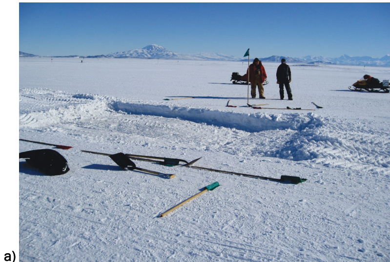
Figure 2. Patching of damaged area of compacted snow runway near McMurdo Station, Antarctica: a) excavated damaged area, b) fresh, tumbled snow being introduced to cavity, c) initial compaction of lower 8-inch layer, d) continued compaction of lower layer, and e) final compaction of upper 8-in. layer (which was placed and compacted in the same fashion as the lower layer).
