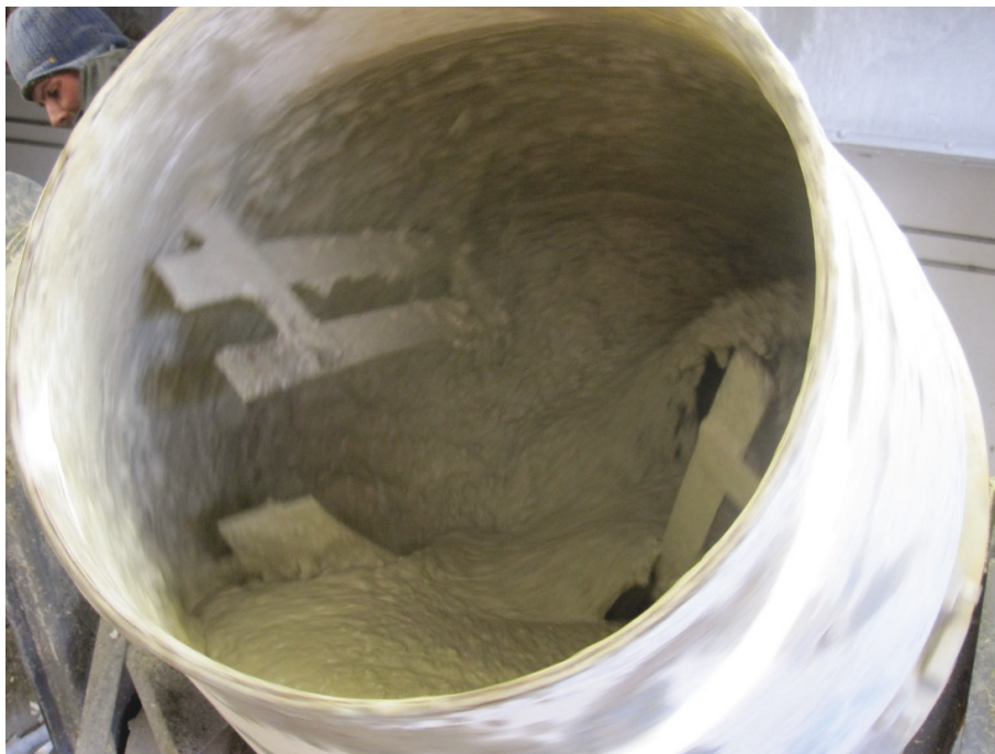
Figure 42. Load of Rapid Set concrete in mixer at 17 °F just prior pouring.
