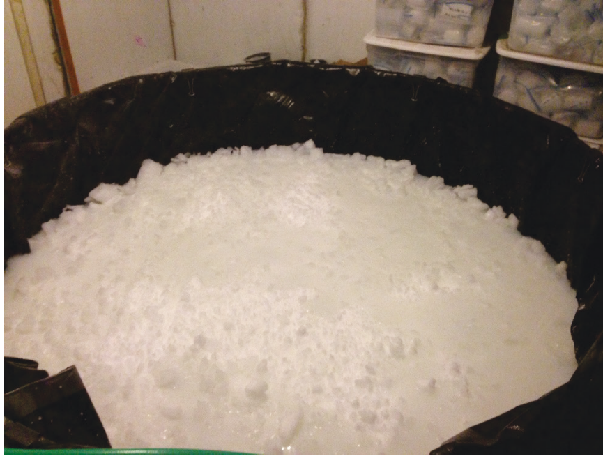
Figure 52. Crater repair with frozen slush at -40\text{ }^{\circ}\text{F} : a) saturated snow surface; b) surface of frozen slush repair. Note: The smooth frozen slush surface in b) is obscured by snow deposition on the top caused by ambient moisture.
