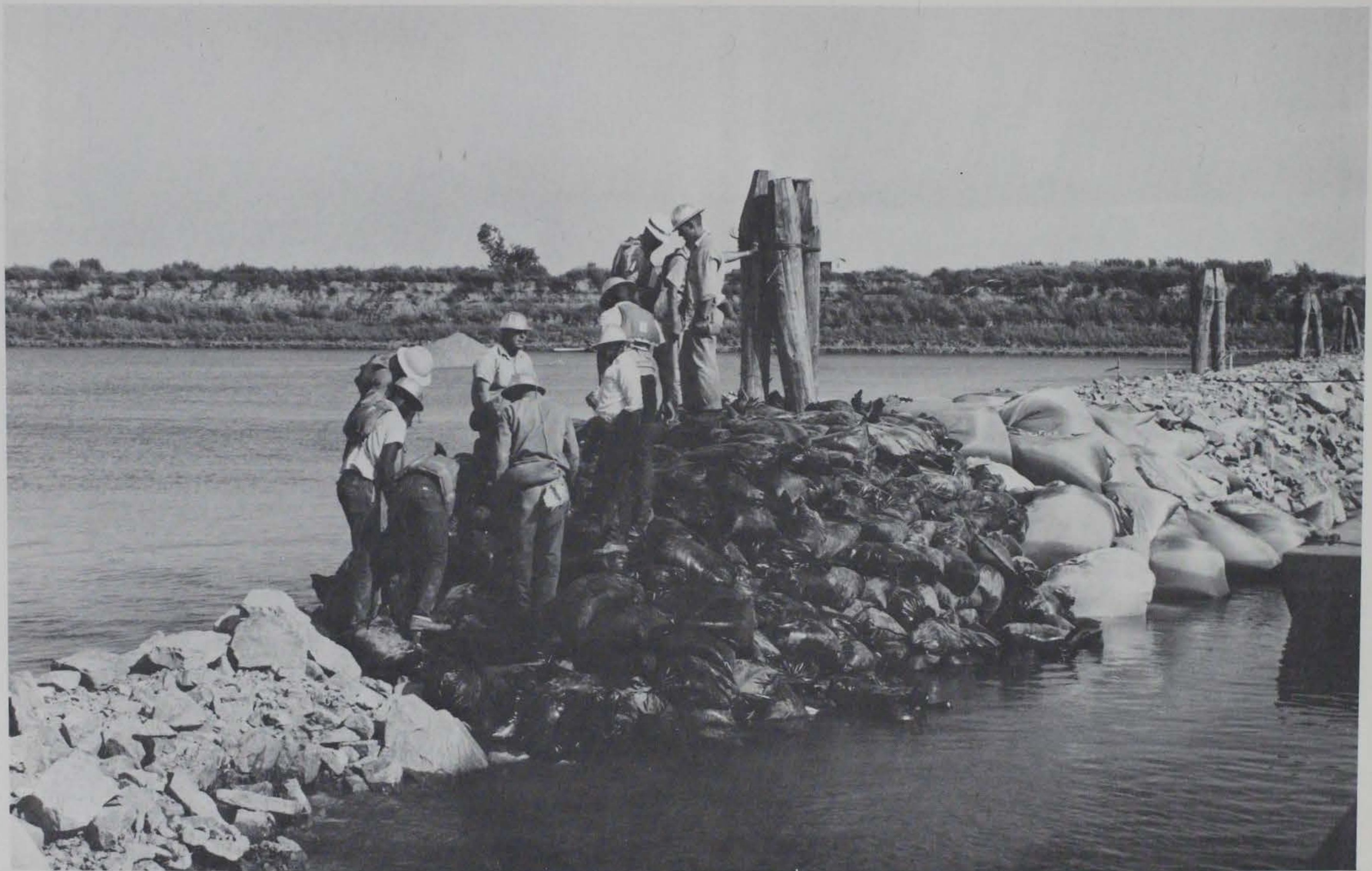
Photograph 20. View looking landward from below dike line. Workmen are hand-placing plastic bags
