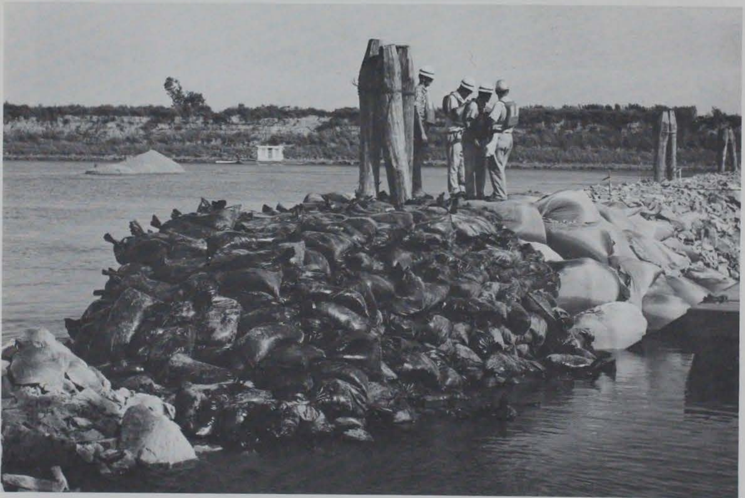
Photograph 22. Looking landward from below dike line. Test section complete except for coating of nylon bags
