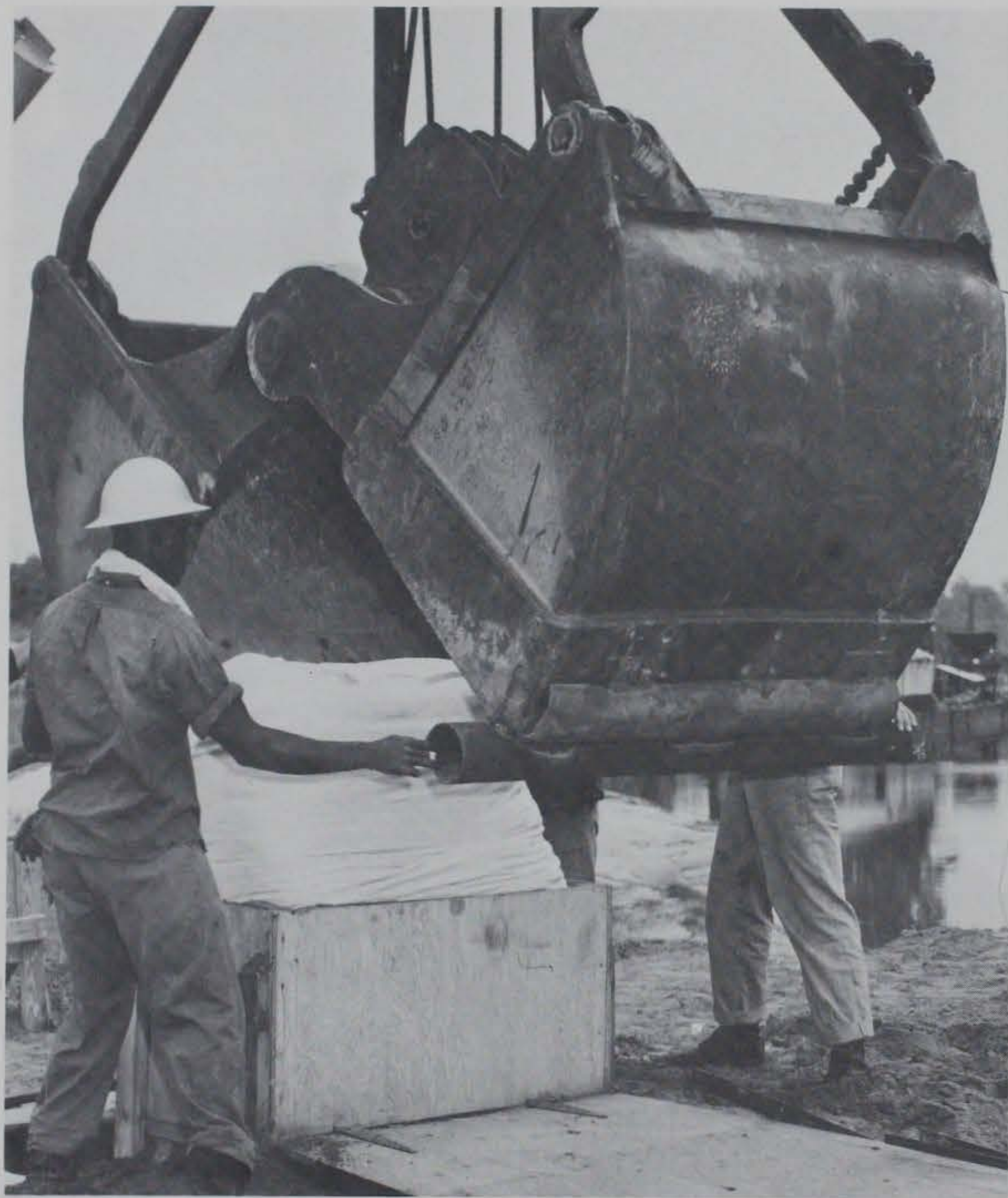
Photograph 6. Clamshell used in handling nylon bags. Note 6-in. pipe welded to jaws of bucket to protect nylon bag from damage
