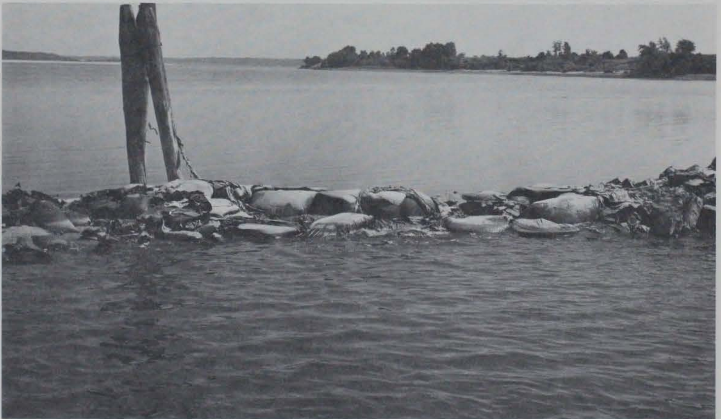
Photograph 29. Upstream profile of damaged nylon bags
