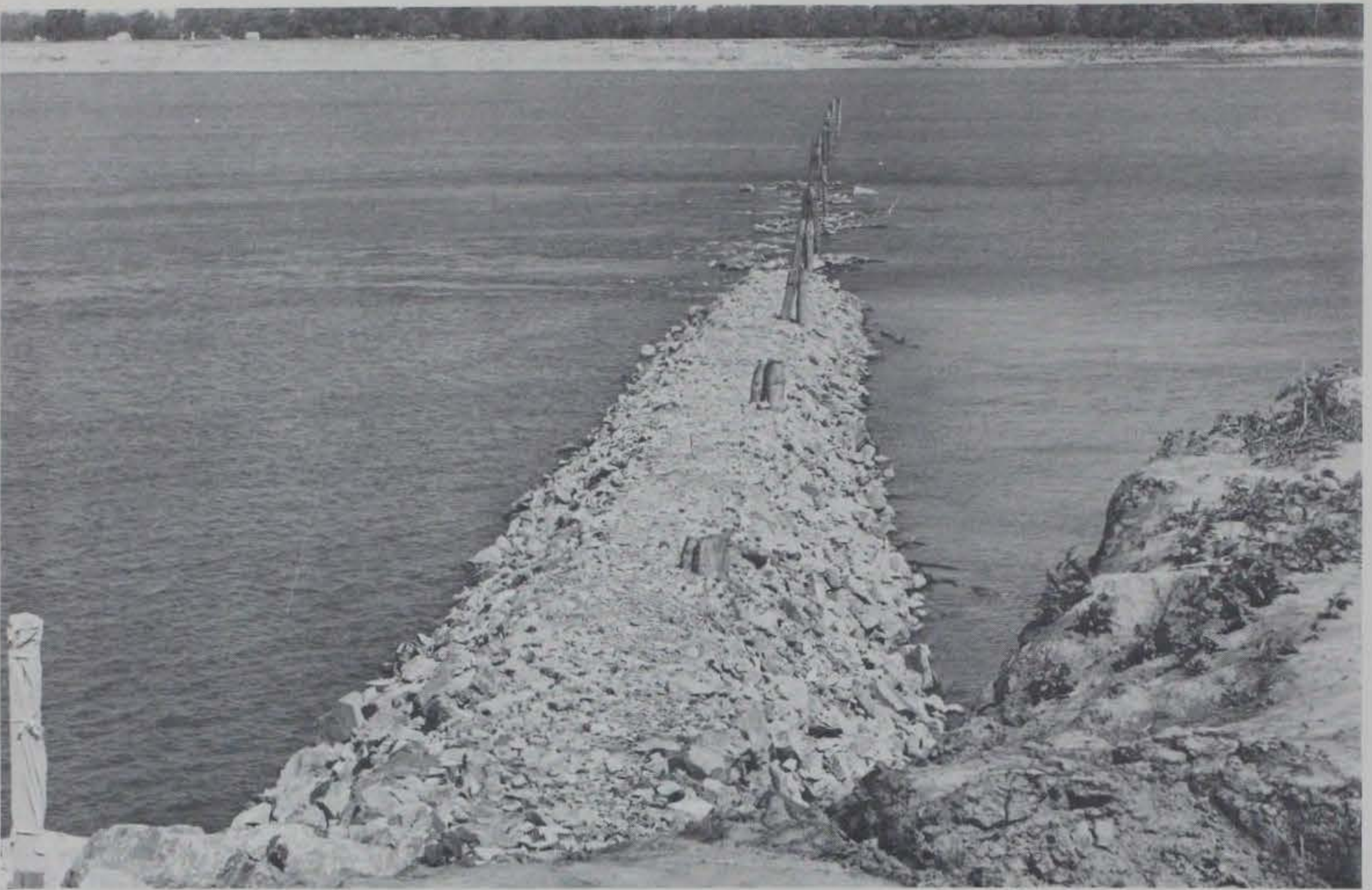
Photograph 12. Dike No. 1 looking riverward along dike line to section where nylon and plastic bags are to be placed. Note stone base extending 400 ft beyond completed portion of dike to experimental section
