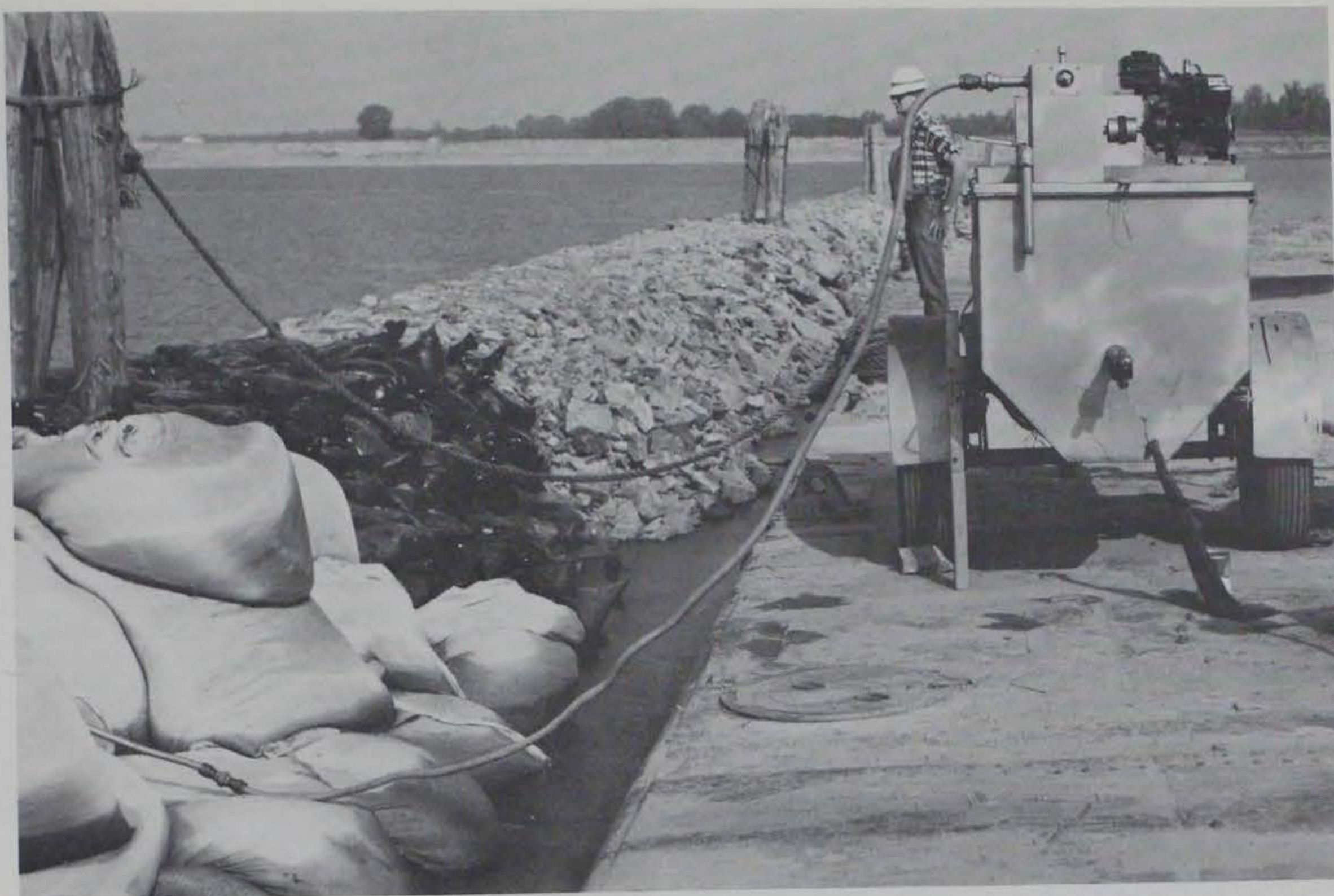
Photograph 23. View showing tank, compressor, and flexible hose to be used for spraying nylon bags
