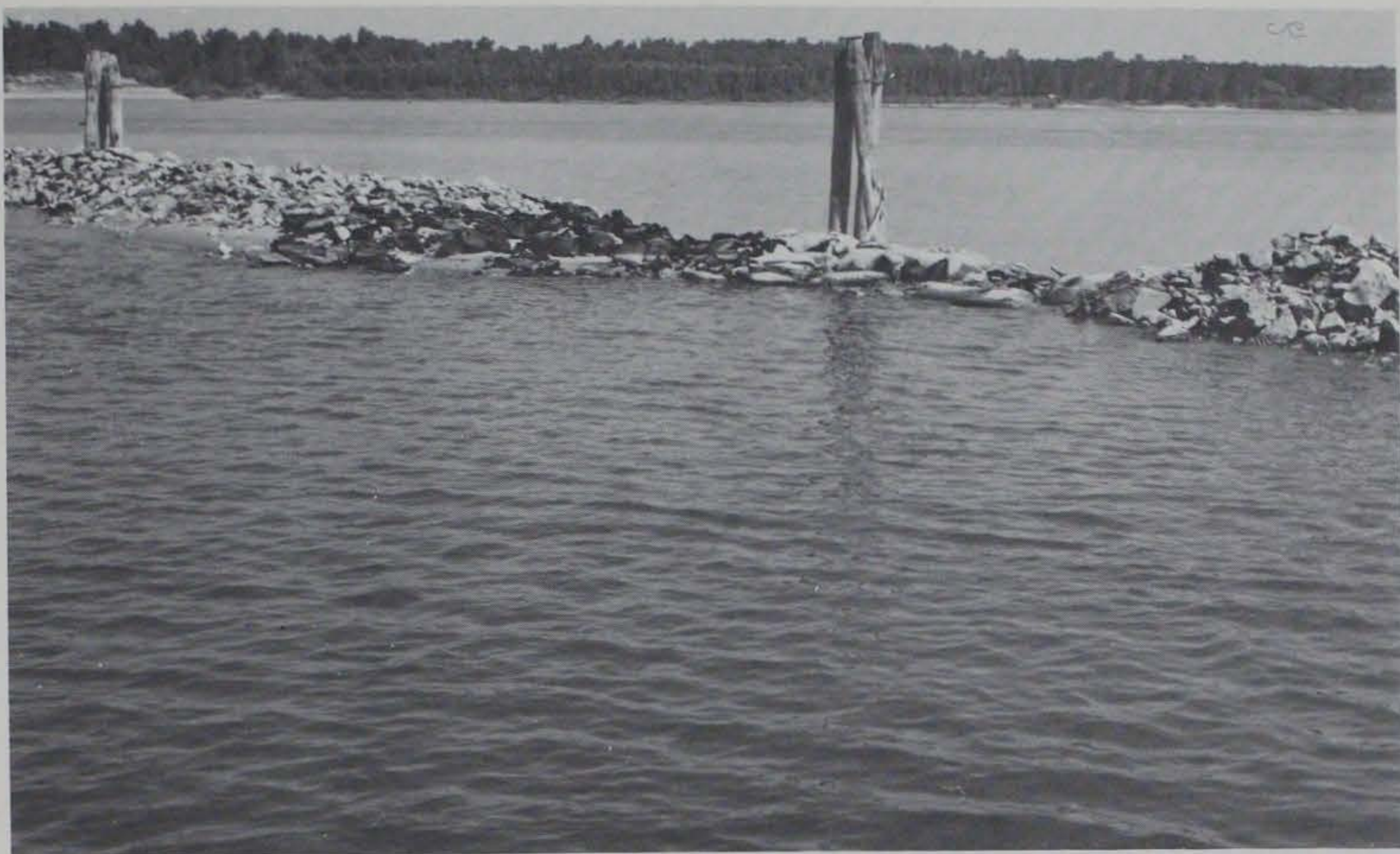
Photograph 26. Looking upstream, showing profile of damaged bag dike
