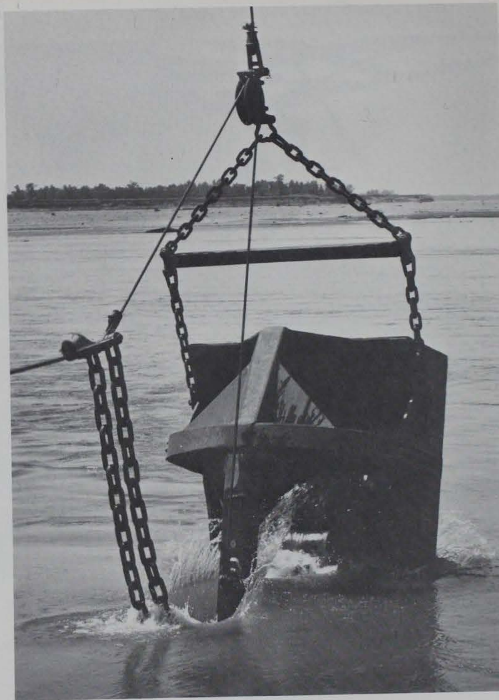
Photograph 18. Load of plastic bags being dumped in base of dike
