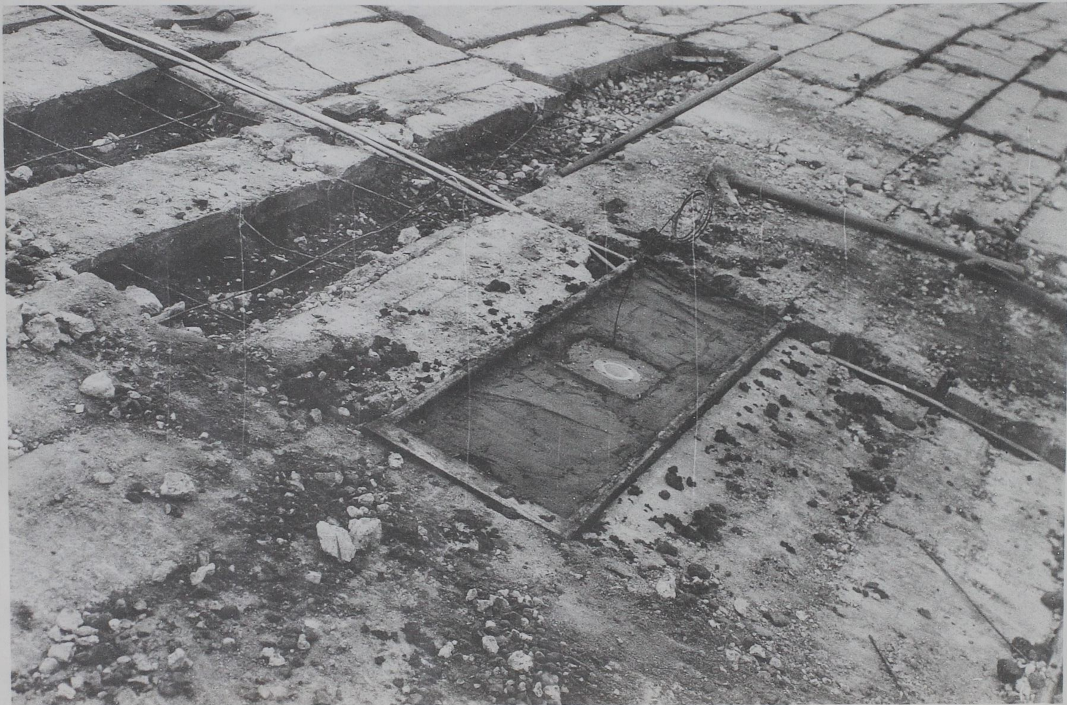
PHOTOGRAPH 6. Differential pressure cell installed in revetment after concrete block is remolded around it
