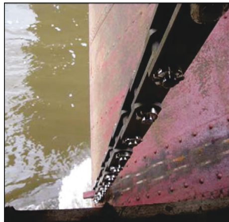
Figure 19. Greaseless roller chain used to raise and lower spillway gate.
