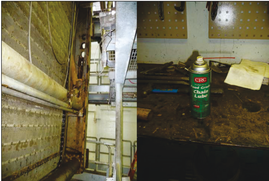
Figure 11. Left- Fish screen undergoing maintenance at John Day Dam, OR. Right- Spray-on chain lubricant.
