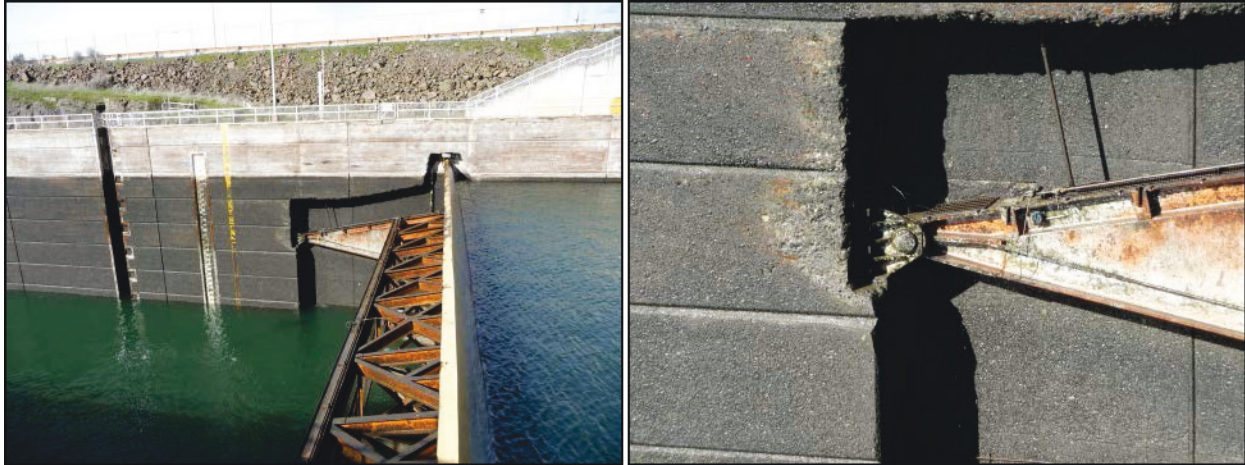
Figure 20. Upper Tainter gate at The Dalles Dam.
