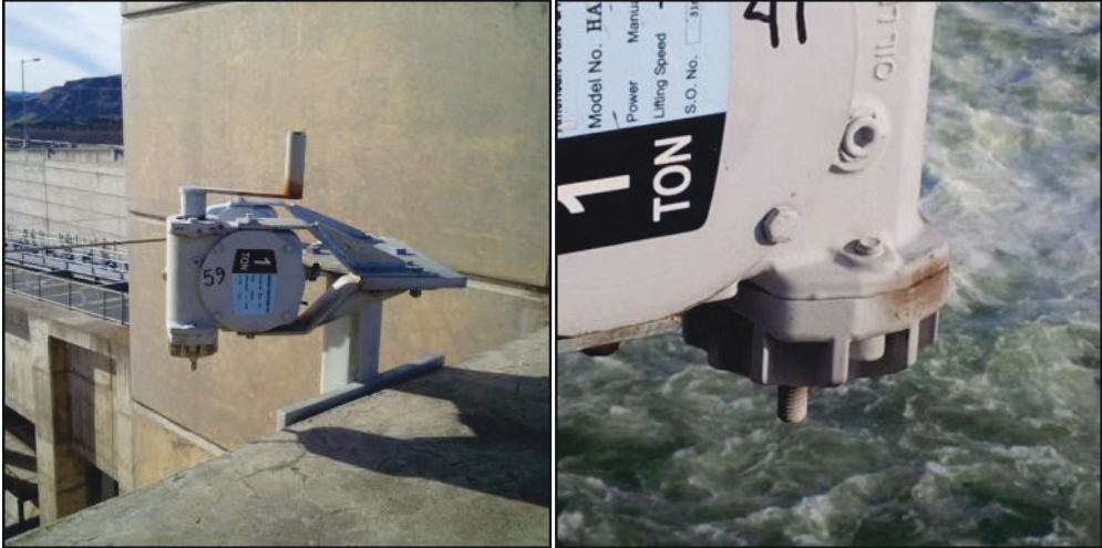
Figure 29. Cable ratchets at John Day Dam.
