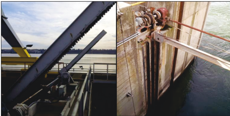
Figure 25. Left - Heavily greased above-water gearing for movement of adjustable fishway weirs at McNary Dam. Right - Greased above water cable system movement of adjustable fishway entrance gates, McNary Dam.
