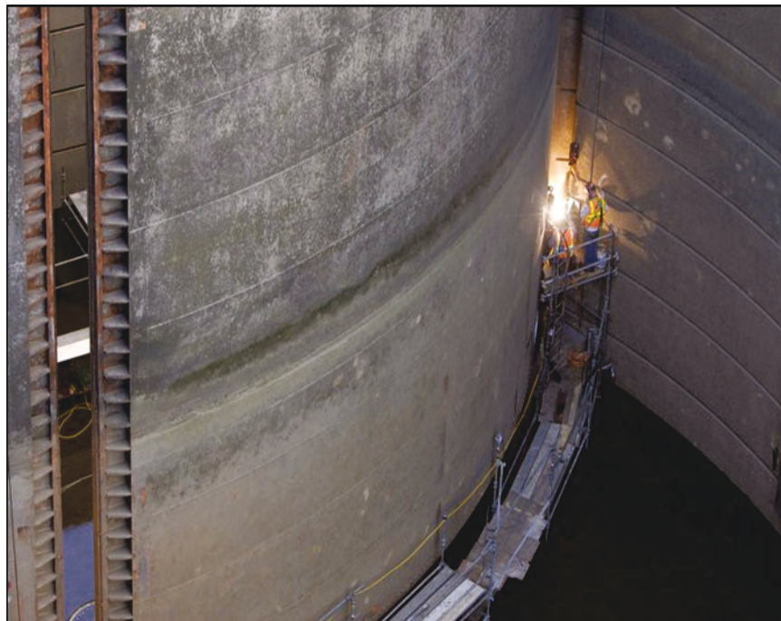
Figure 13. Picture of repairs at The Dalles Dam downstream miter gate in 2010, which also shows the massive size of the structure.
