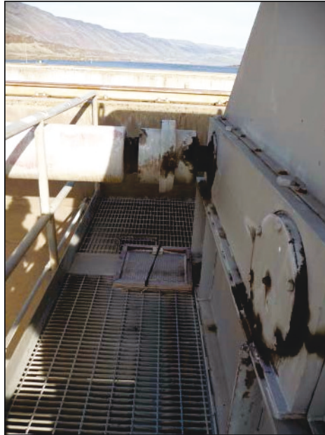
Figure 24. Suspended gate motor showing lubricant leakage at The Dalles. Sorbent pads controlled dripping below.
