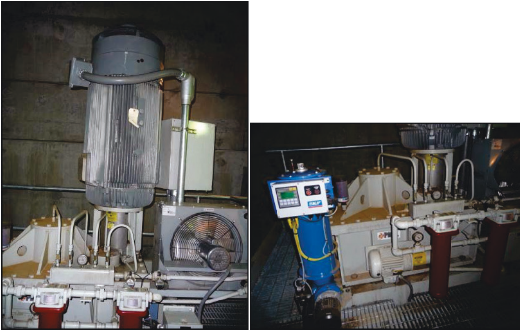
Figure 26. Left- Fish pump at John Day Dam. Right- Grease metering system.
