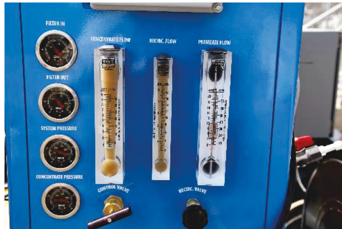
Figure 49. Rotometers to RO system, with the two on the left showing high turbidity in the system, and product flow on the right.
