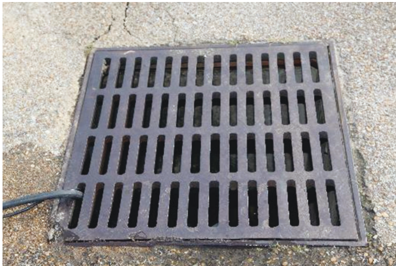
Figure 20. Drain with grate replaced and sump pump hosing/power visible.
