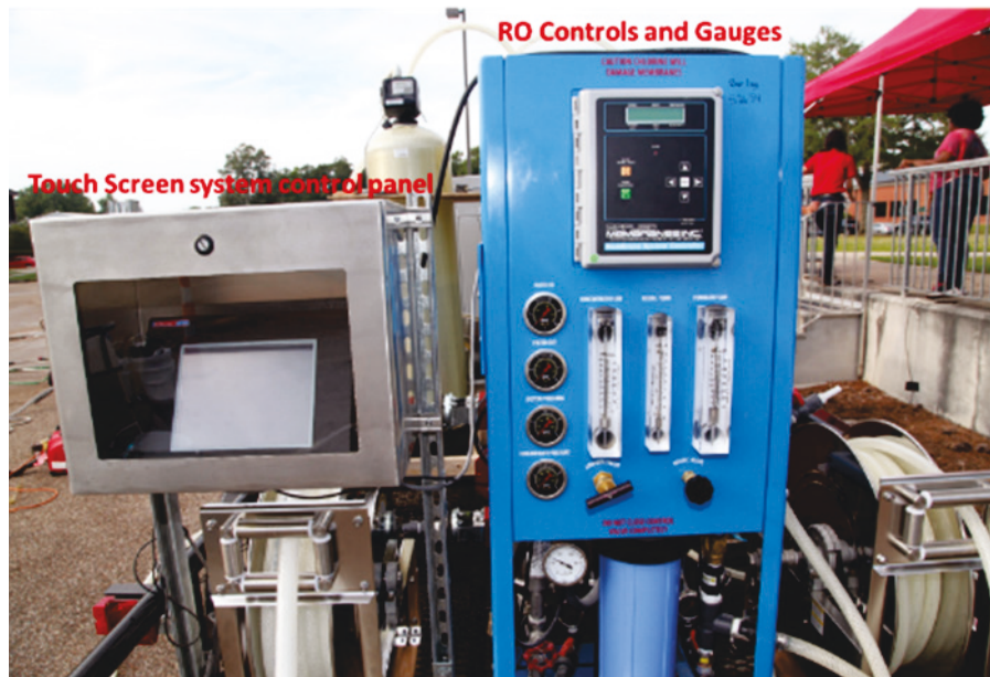
Figure 9. The touch screen control system (left) and the controls and monitoring gauges for the RO system (right).
