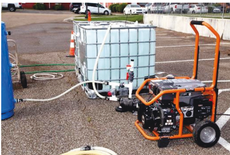
Figure 45. Supplemental generator used in this study to address amperage surge associated with the mechanical phase converter.
