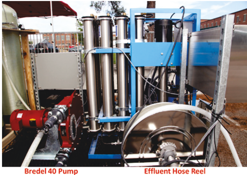
Figure 4. The Bredel 40 pump and hose reel used in the DETS.
