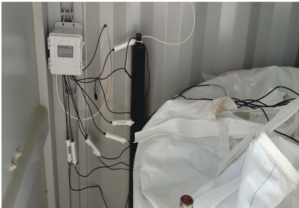
b. Cabling attached to logger device at end of conex.
