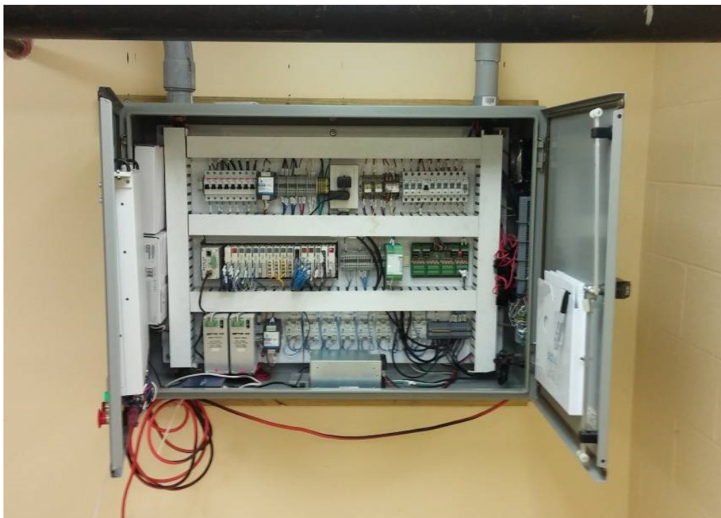
Figure 9. Fully instrumented and wired master control unit.
