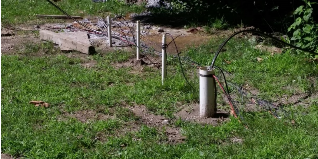
Figure A18. Field installation showing (near to far) Well 1 and PZ-1, PZ-4, and PZ-2.
