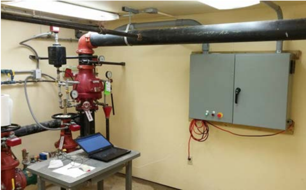
Figure 8. Master control cabinet in basement of building S-3.
