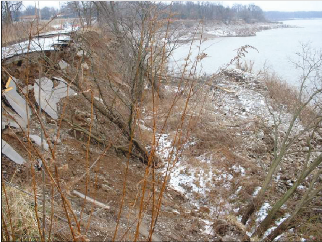
Figure 2. 2004 Bank erosion in problem area.
