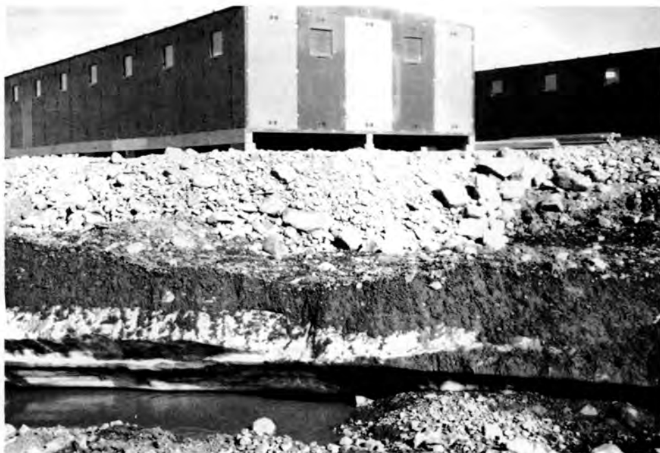
(b) An ice mass in glacial till revealed by excavation. The building above has been erected on a fill of free-draining stony material, which prevents the ground from thawing.
