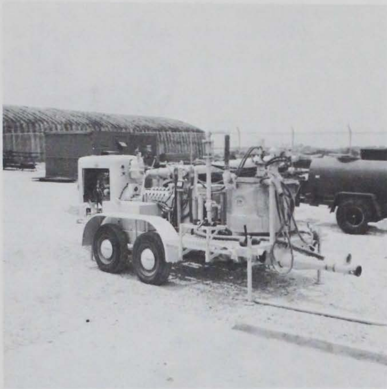
Figure 5.37 Batching and pumping unit 2.
