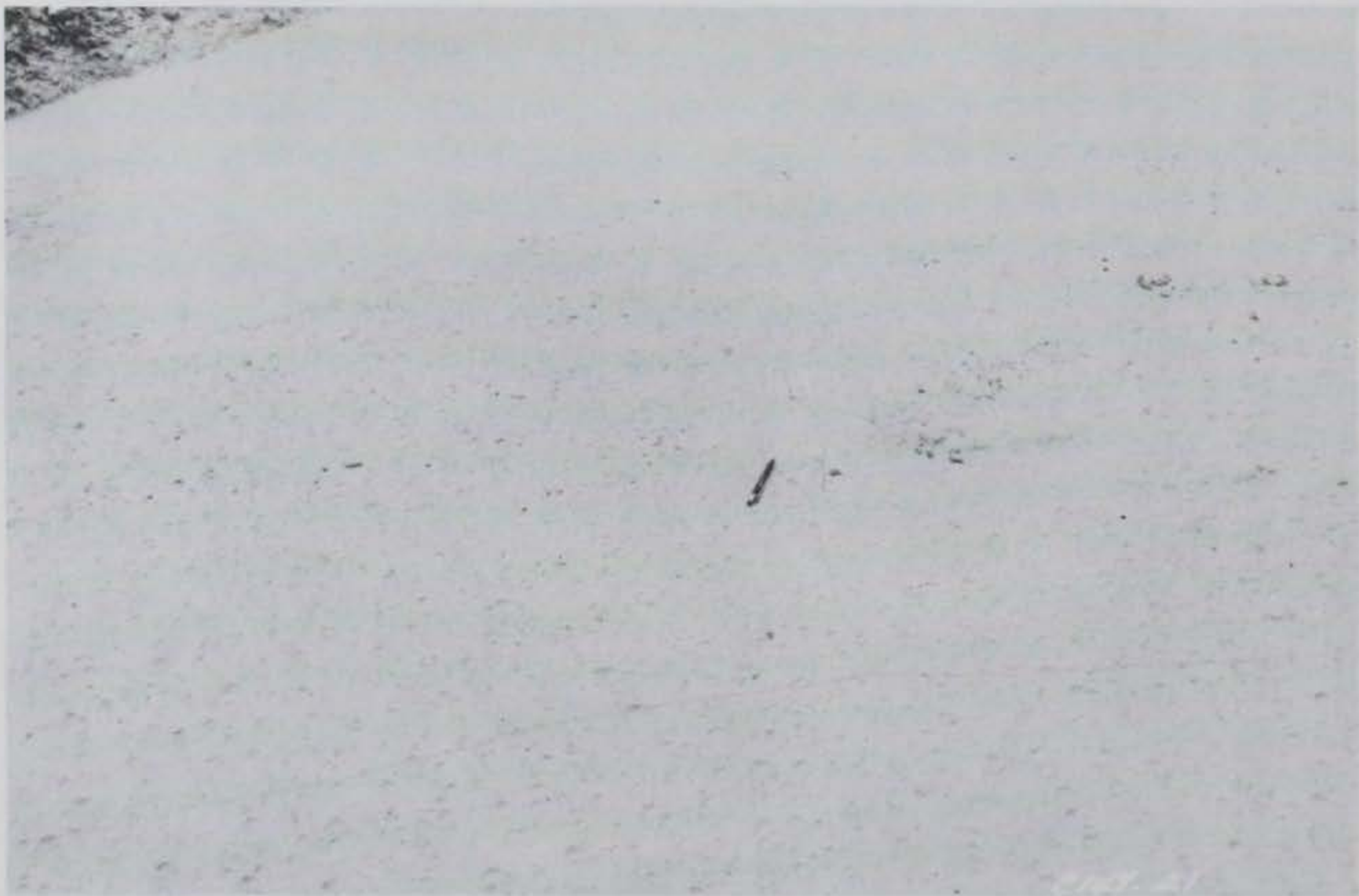
Figure 5.28 Surface of repair showing some drying shrinkage cracking.
