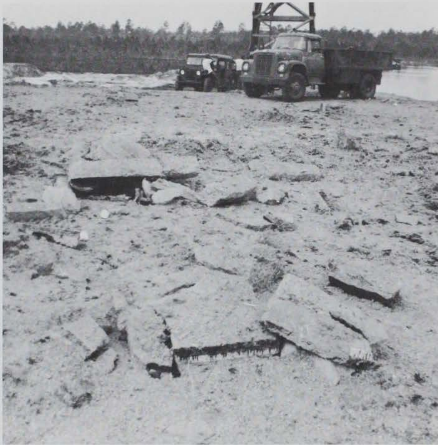
Figure 1.9 Pieces of concrete pavement blown out by the explosion.
