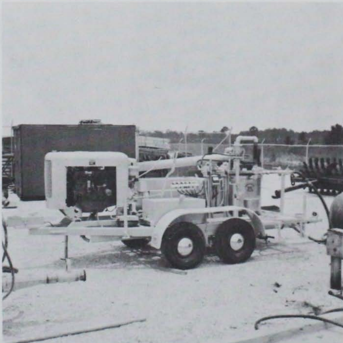
Figure 5.36 Batching and pumping unit 1.
