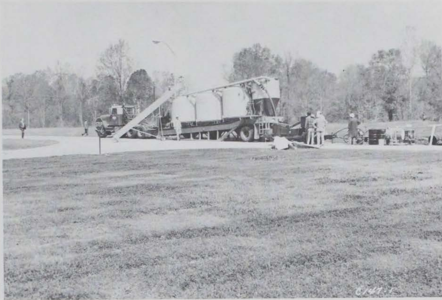
Figure 5.13 Field storage tank cement delivery system.
