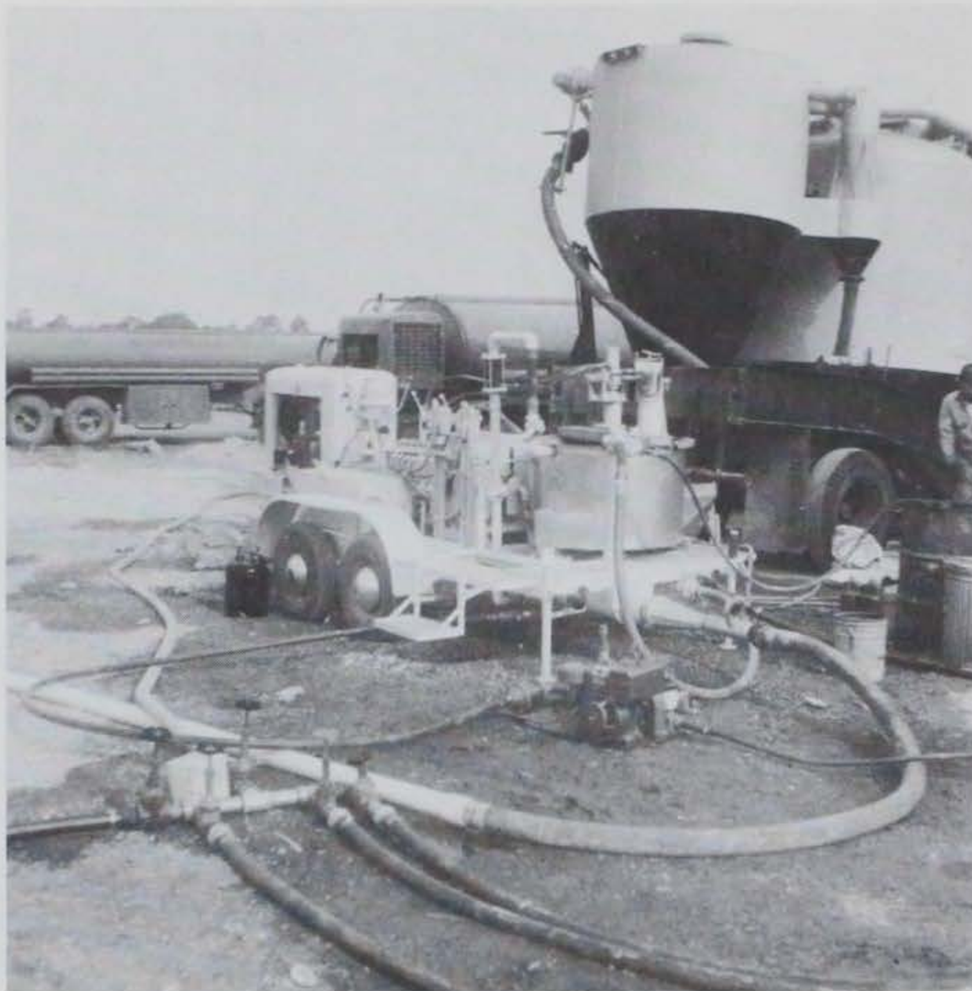
Figure 5.39 Unit 2, foam generator, and cement supply arrangement.
