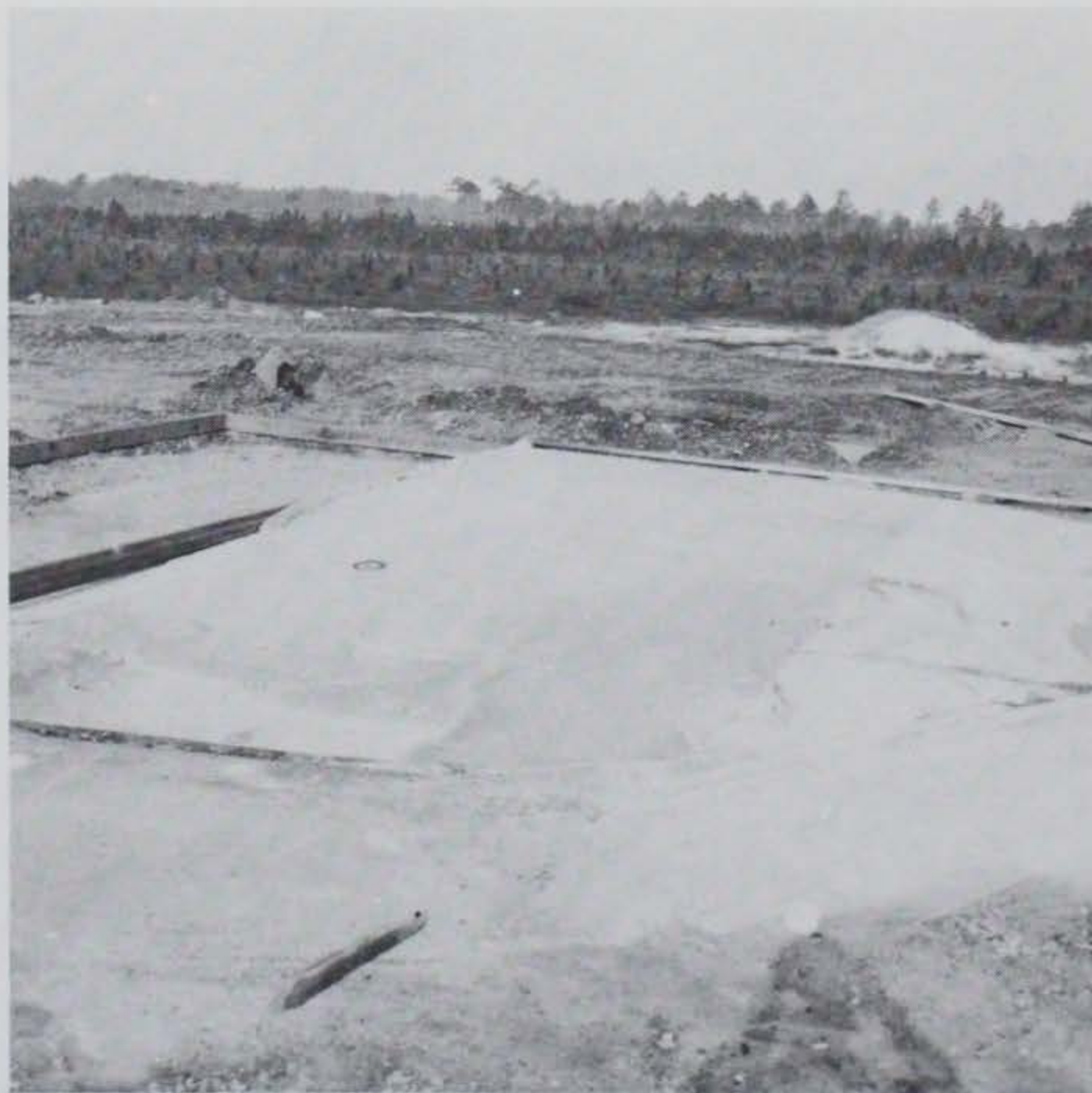
Figure 5.48 Incomplete repair surface.
