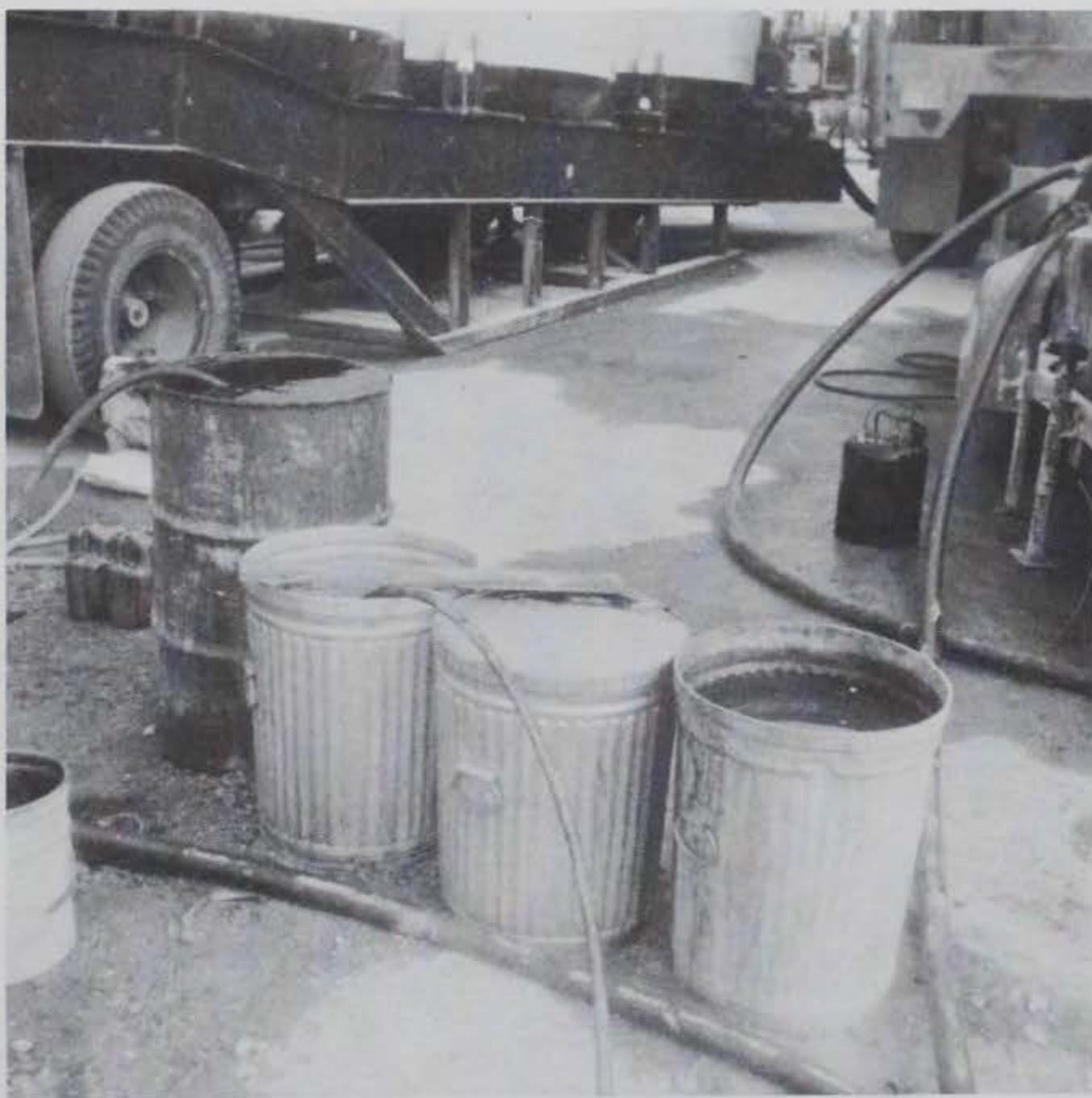
Figure 5.42 Holding tanks for foam solution and retarder concentrate.
