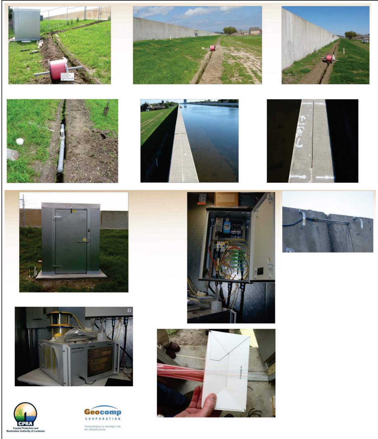
Figure 5-67. View of Site 5 monitoring system consisting of fiber optic sensor system for monitoring strain displacements at the levee toe and I-wall at the 17th Street Canal in New Orleans for the iLevee monitoring demonstration project (Brouillette 2012).
