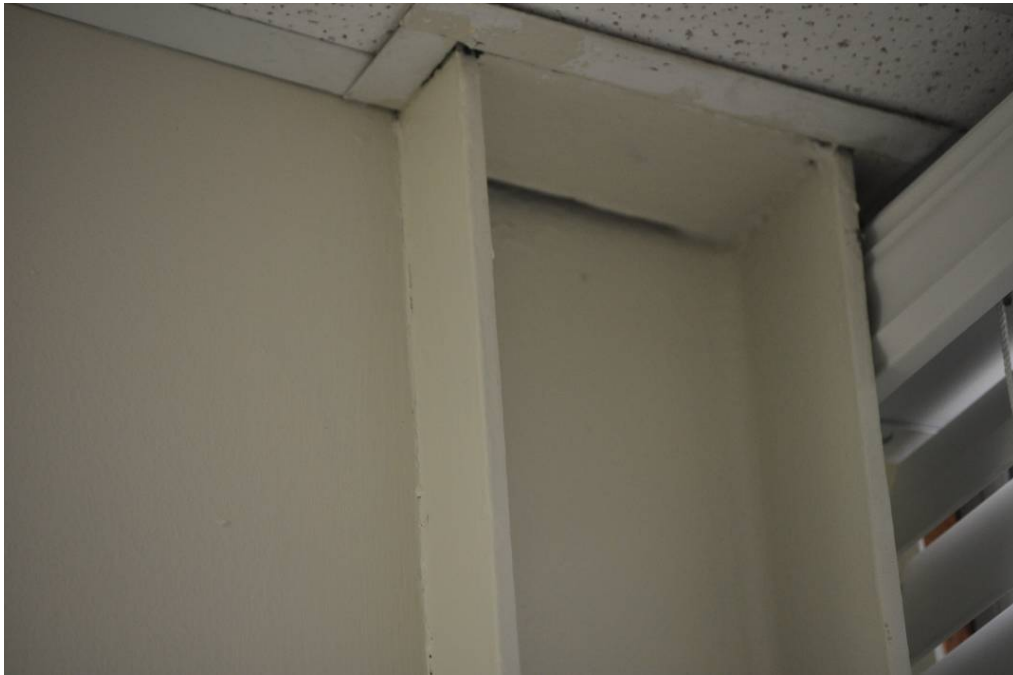
Figure 15. I- beam in Room 11 after 4 months.
