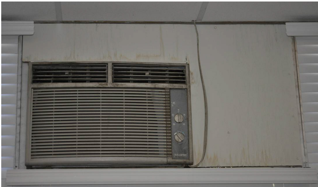
Figure 36. Window air-conditioning unit in Room 11, after 12 months.
