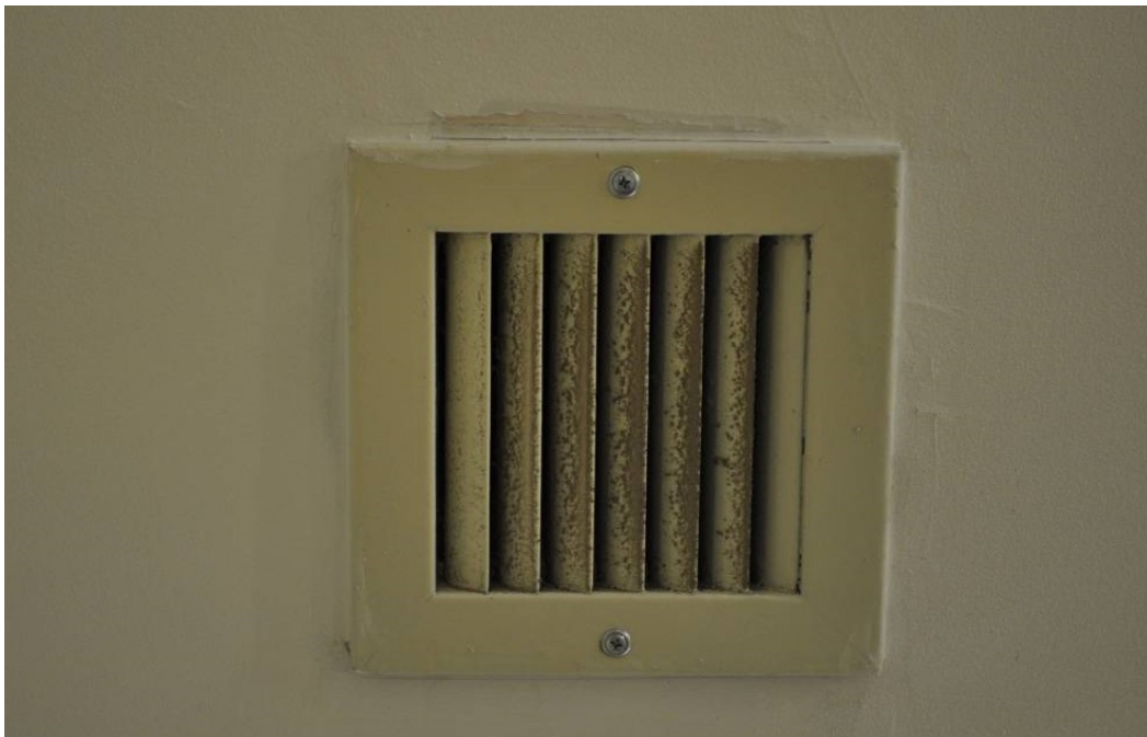
Figure 33. Vent in Room 4 after 12 months; inspector noted that no mold was present.
