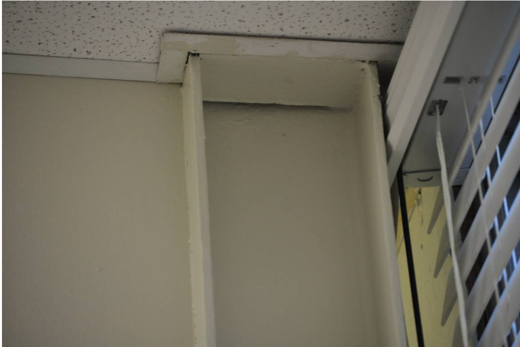
Figure 27. I-beam in Room 11 after 8 months.
