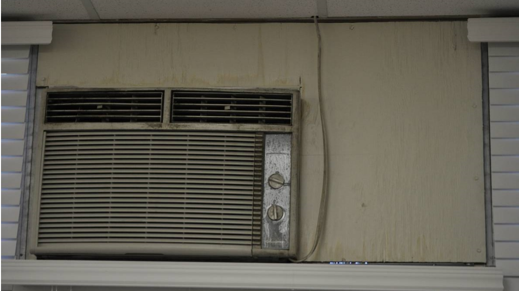
Figure 25. Window air-conditioning unit in Room 11 after 8 months.
