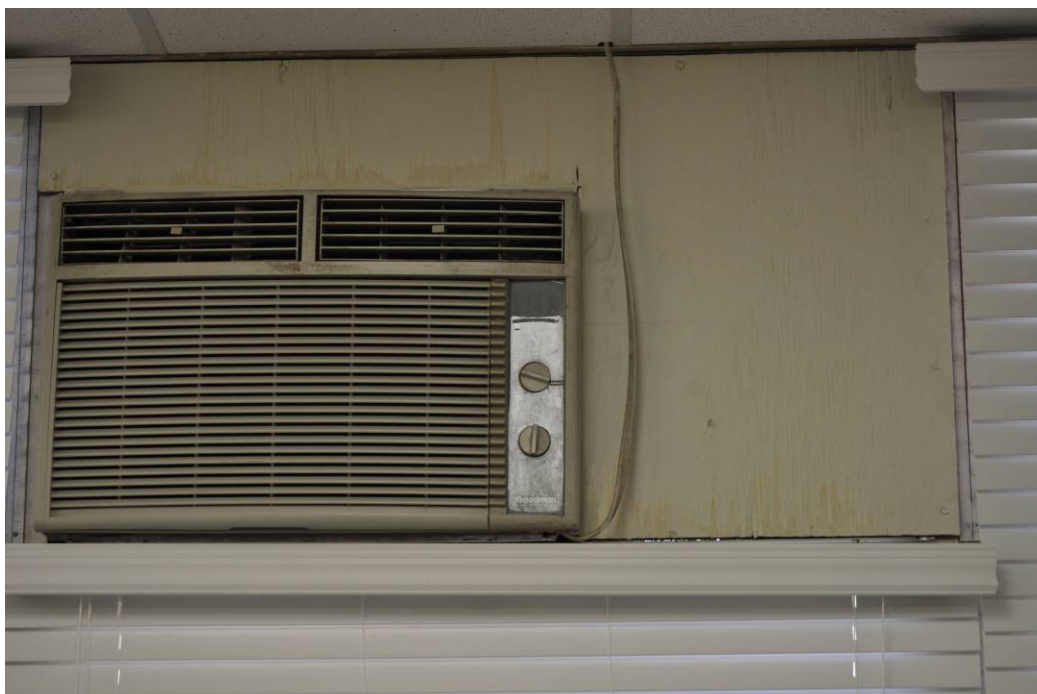
Figure 16. Window air-conditioning unit in Room 11 after 4 months.
