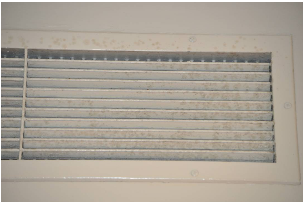
Figure 38. Air vent in Room 11, after 12 months.
