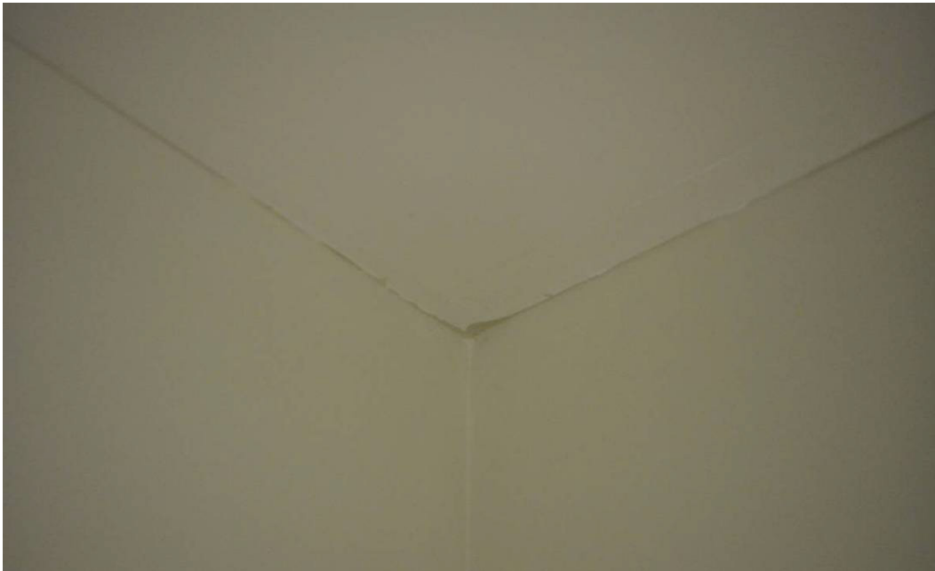
Figure 23. Washroom of Room 9, after 8 months, with an unknown coating on the block walls. Caliwel is still present on the ceiling.
