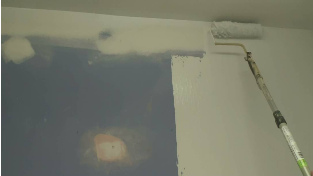
Figure 4. Sherwin Williams ProMar 200 acrylic primer applied to new gypsum board installed in Room 9.
