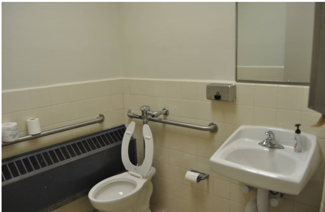
Figure 12. Washroom of Room 9 recoated with an unknown coating after 4 months.
