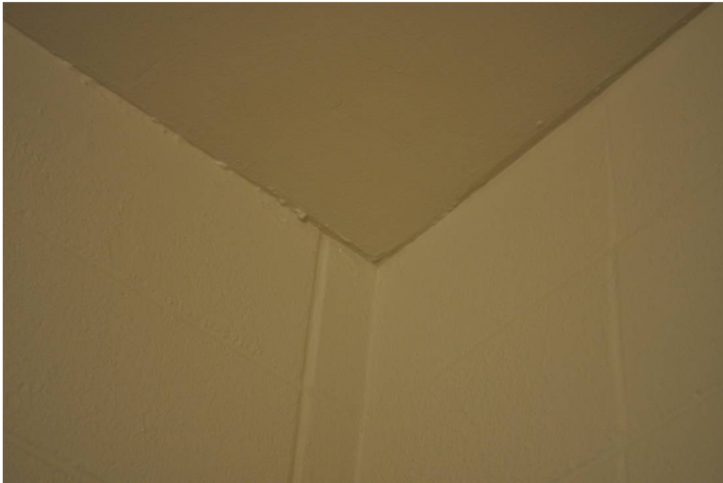
Figure 41. Block walls and gypsum ceiling of washroom next to Room 14 after 12 months.
