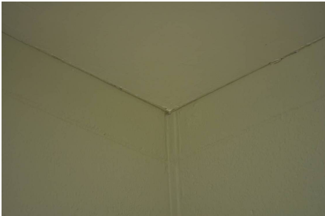
Figure 24. Washroom of Room 9, after 8 months, with unknown coating on the block walls. Caliwel is still present on the ceiling.
