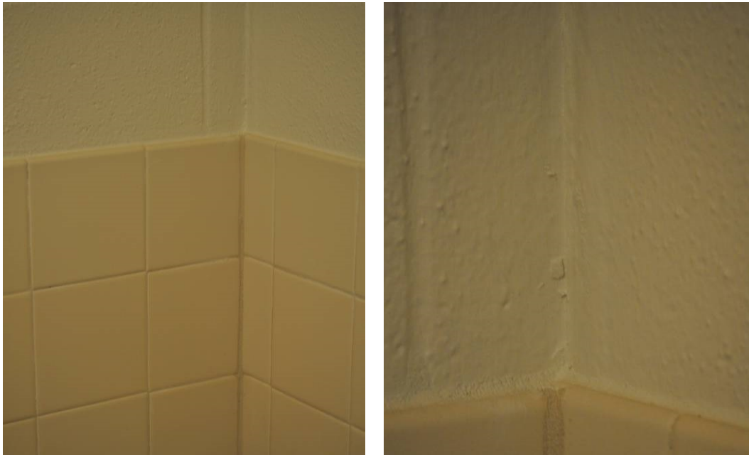
Figure 28. Washroom next to Room 14 after 8 months.
