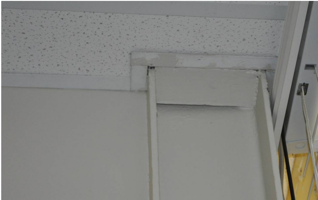
Figure 37. I-beam in Room 11, after 12 months.
