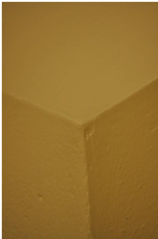
Figure 30. Block walls and gypsum ceiling of the washroom next to Room 14 after 8 months.
