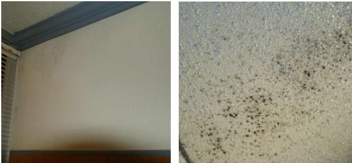
Figure 1. Mold in Fort Polk barracks on concrete block walls and concrete ceiling.
