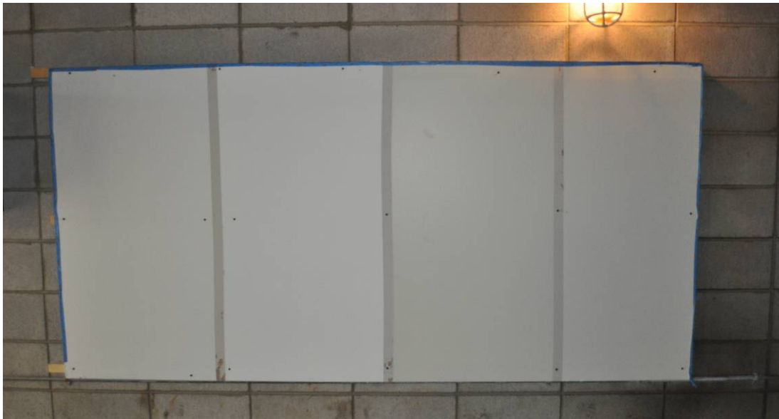
Figure 8. Gypsum board coated with Sherwin Williams ProMar 200, Hirshfield's Platinum Ceramic, Caliwel, and Foster 40-20 (left to right) in 2 x 4 foot sections and hung in the mechanical room of Building 1630.
