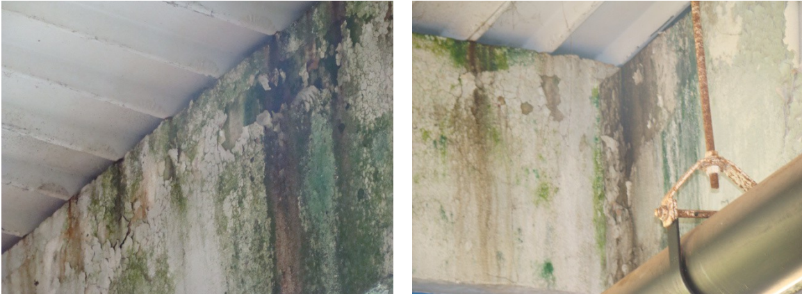
Figure 2. Mold in Fort Polk pumphouse with concrete block walls.
