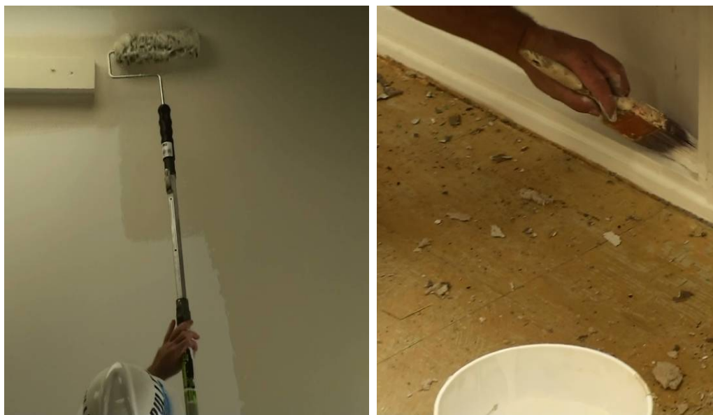
Figure 5. Coating application using 1-inch nap roller (left) and nylon brushes (right) for Sherwin Williams and Hirshfield's coatings.
