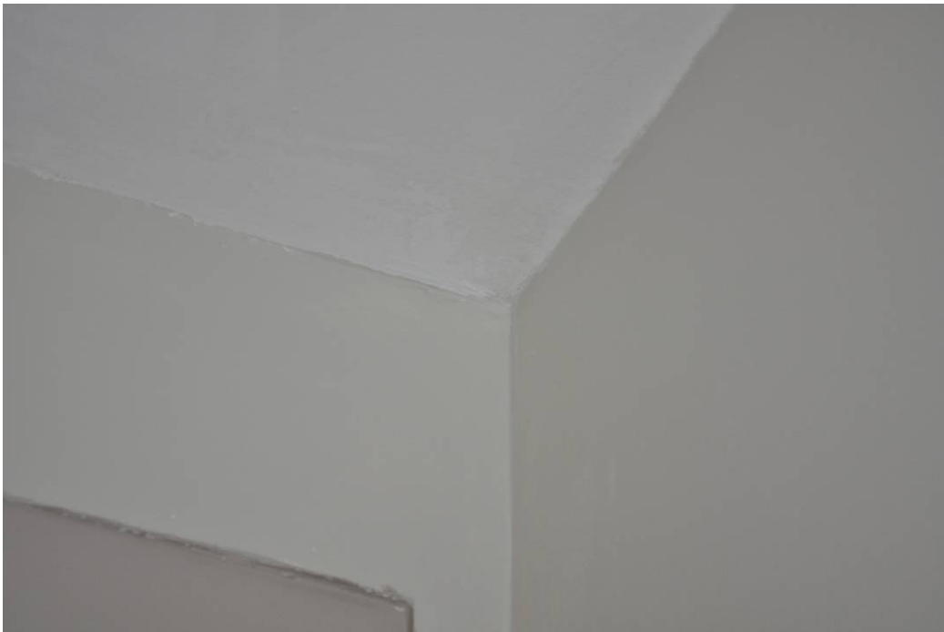
Figure 10. Walls in Room 4 coated with an unknown coating, and ceiling coated with Foster 40-20 after 4 months.
