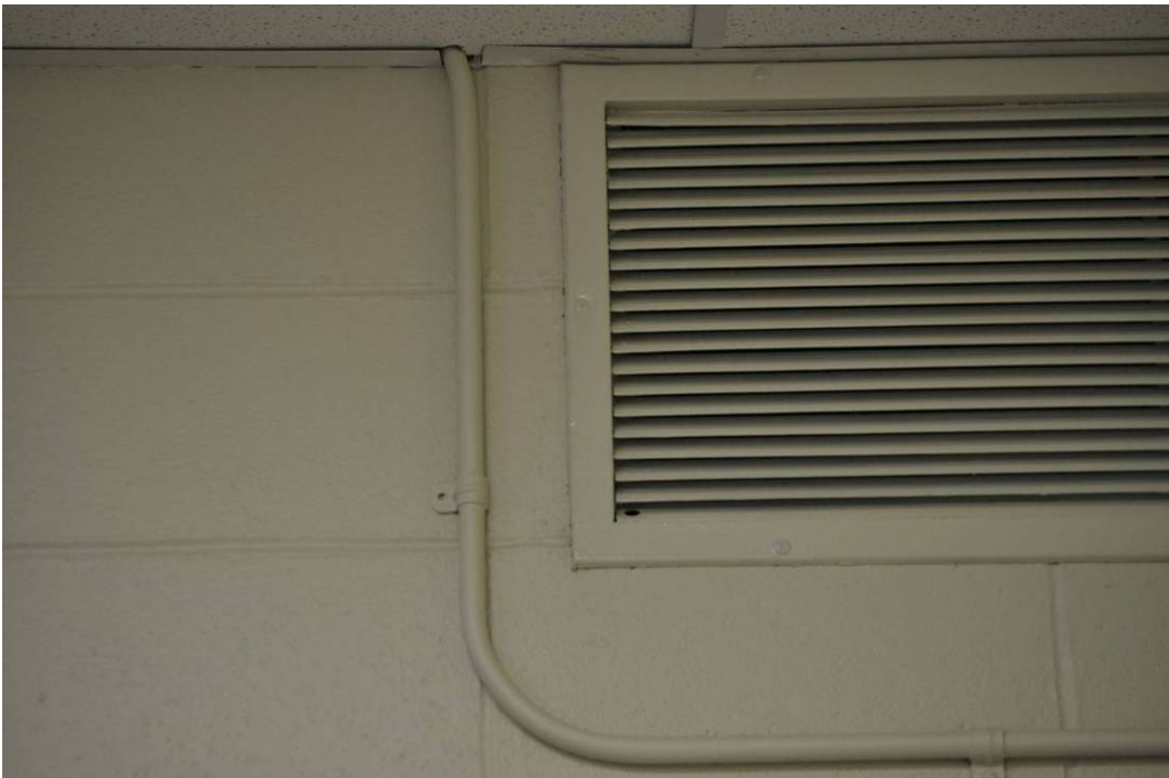
Figure 26. Air vent in Room 11 after 8 months.
