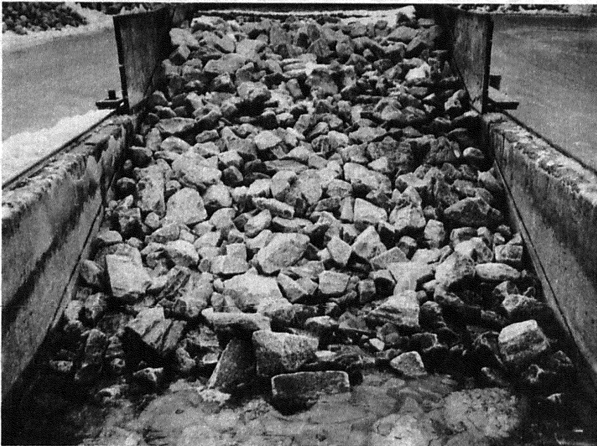
Figure 10. Riprap at a level of damage corresponding to the "greatest tolerable damage."
