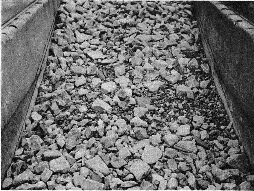
Figure 9. Closeup of failure shown in Figure 8.
