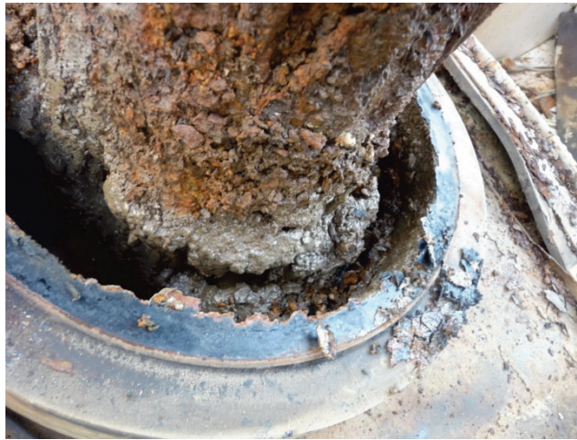
Figure 2.10. Example of accelerated corrosion due to biological agents in existing grease (Ebeling et al. 2013).
