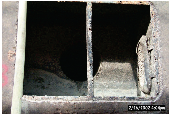
Figure 2.4. Example of anode protecting ship's hull (cathode). This is the U.S. Army Corps of Engineers Dredge Jadwin in dry dock. Note the partially consumed anode (to the right) at the entrance of the engine cooling water intake.
