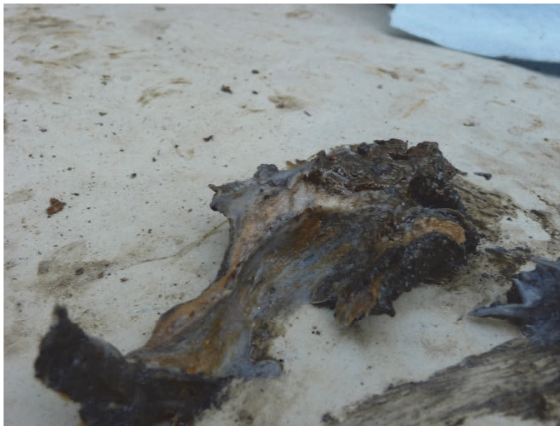
Figure 2.12. Grease with biological growth at John Day lock when anchor head was removed (Ebeling et al. 2013).
