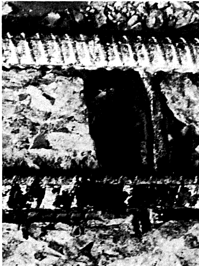
Photo 30. Corrosion on reinforcement adjacent to weld
