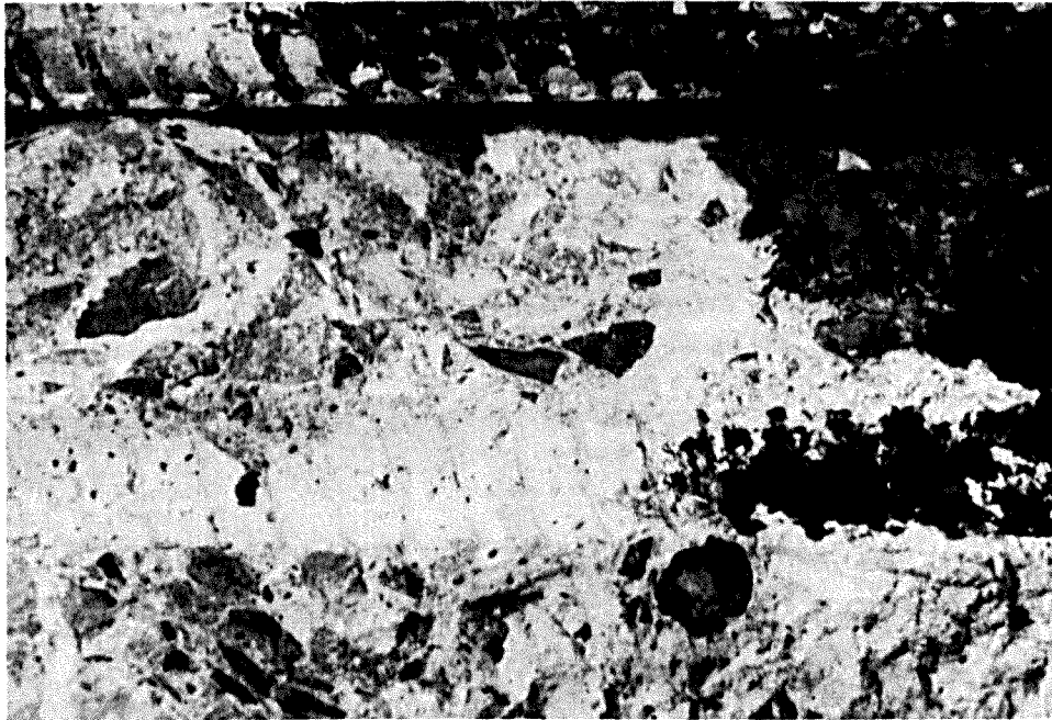
Photo 32. Corrosion on reinforcing bar adjacent to spalled area
