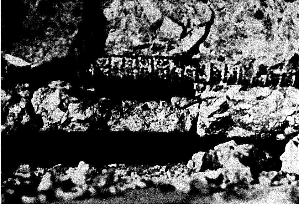
Photo 33. Moderate amounts of corrosion on reinforcement
