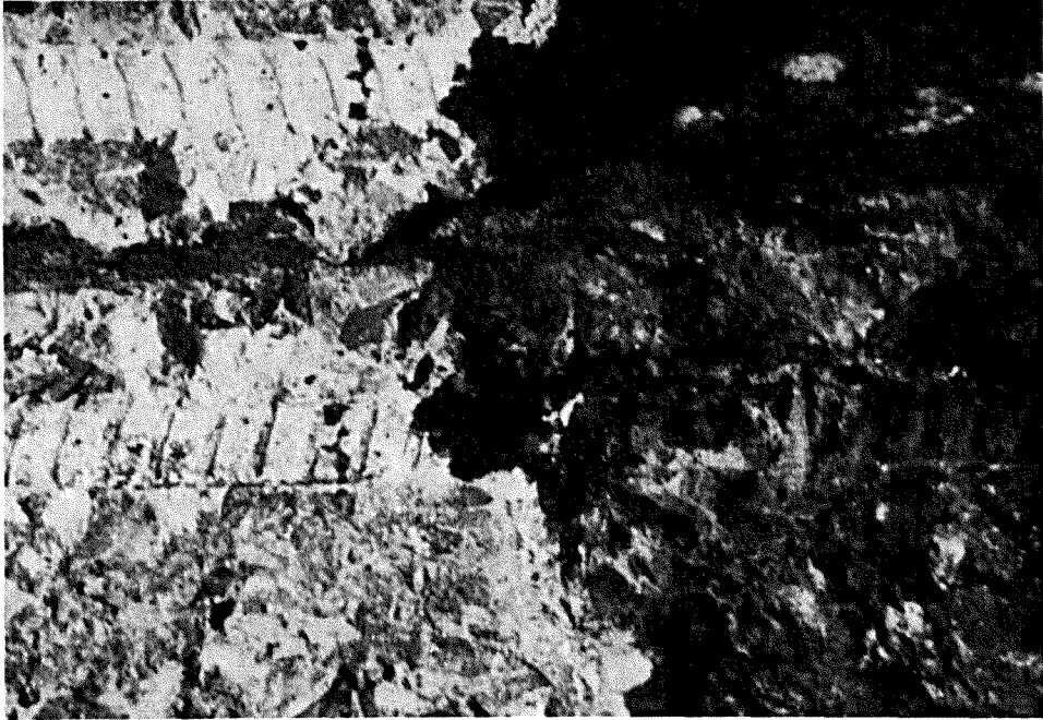
Photo 31. Corrosion on reinforcement at spalled area
