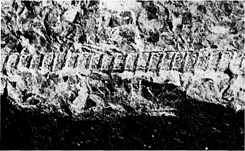
Photo 37. Uncorroded condition of reinforcement bar beneath unspalled concrete
