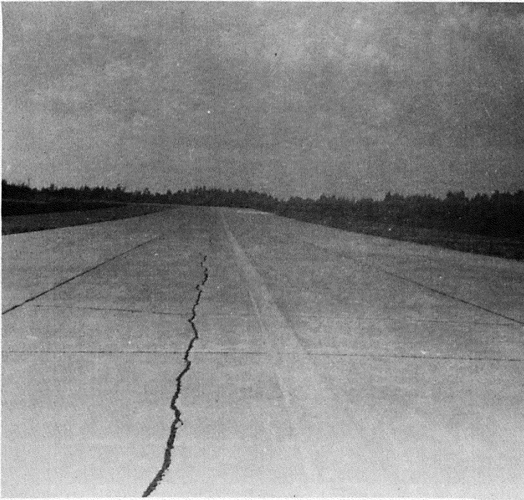
Photo 5. Cracks in taxiway G
