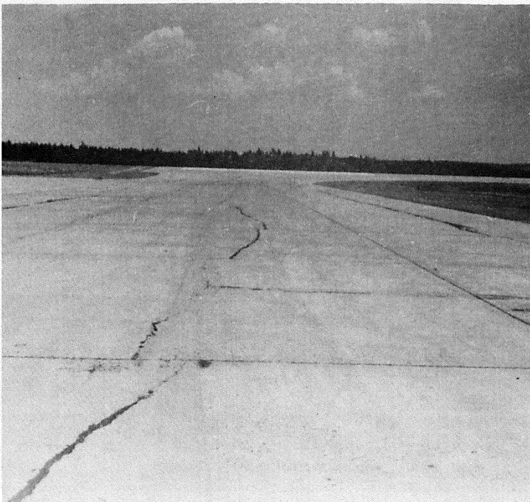
Photo 6. Cracks in north connecting taxiway
