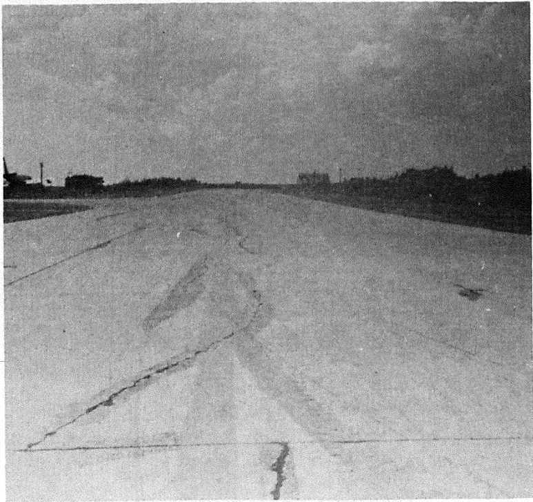
Photo 4. Cracks in taxiway E west of intersection with taxiway G
