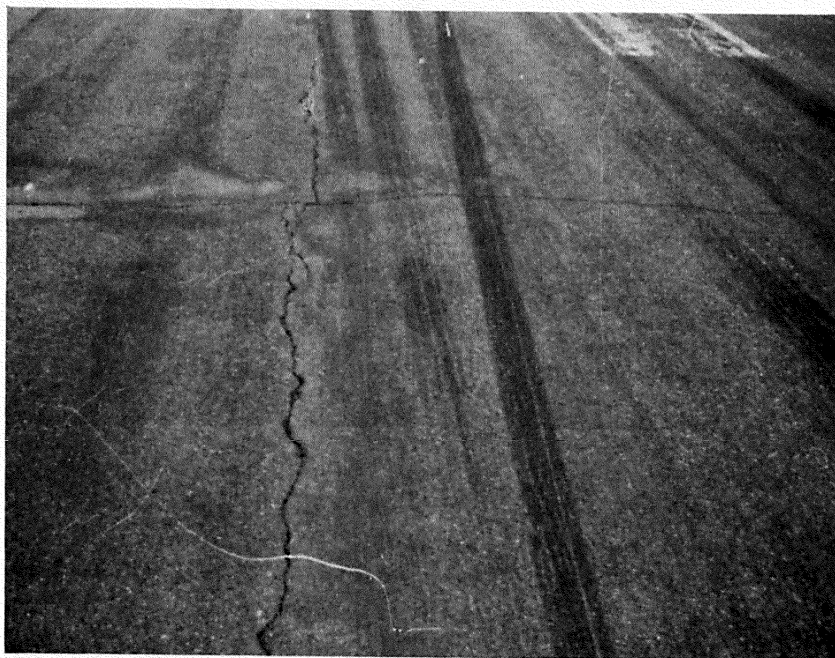
Photo 2. Cracks with slightly raised edges on NW-SE runway
