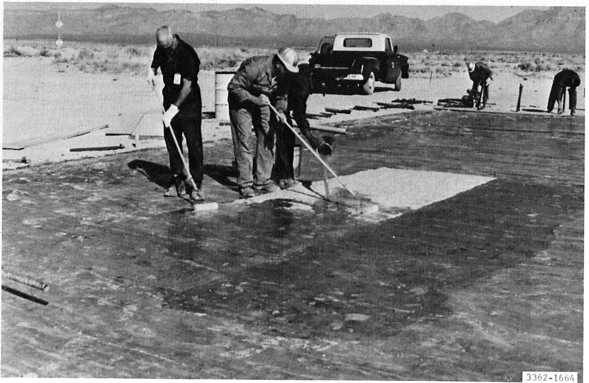
Photograph 28. Buildup in impingement area
