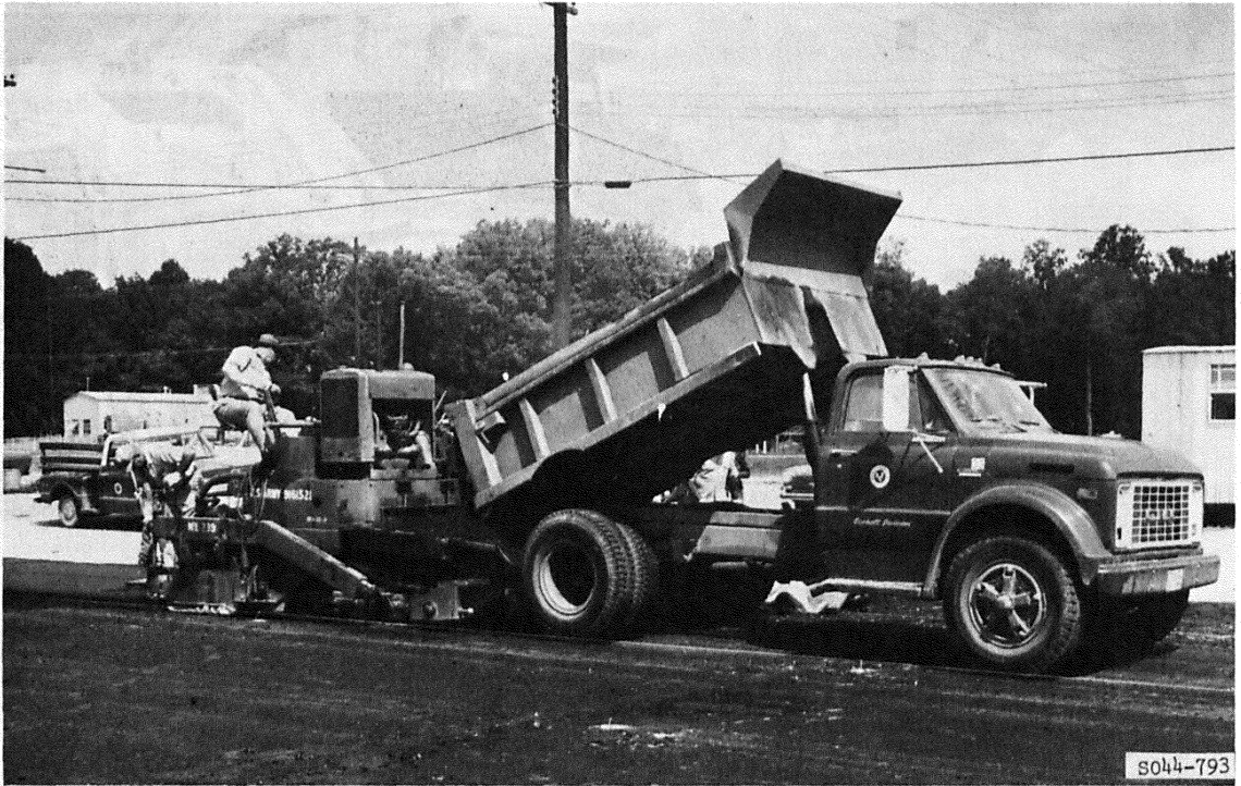
Figure 40. Placement of 3-in.-thick asphaltic concrete surface course on the flexible pavement test section
