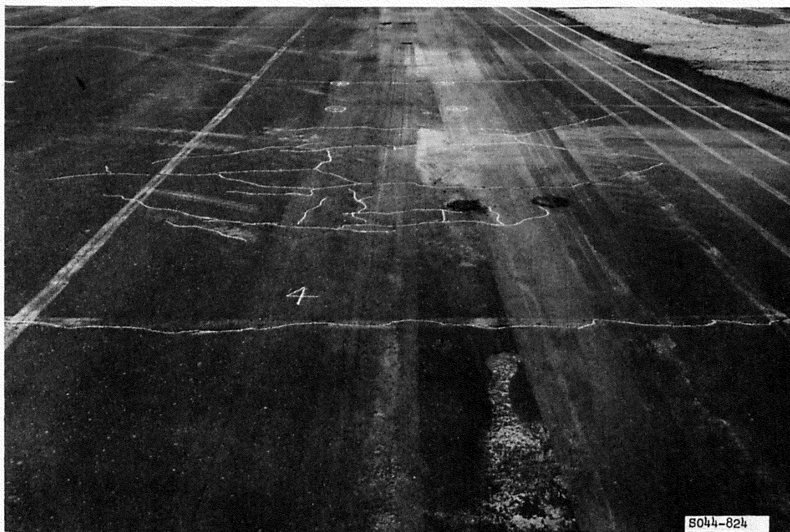
Figure B10. Cracking in item 4, lane 1, flexible pavement test section, after 1200 coverages of 200-kip twin-tandem assembly
