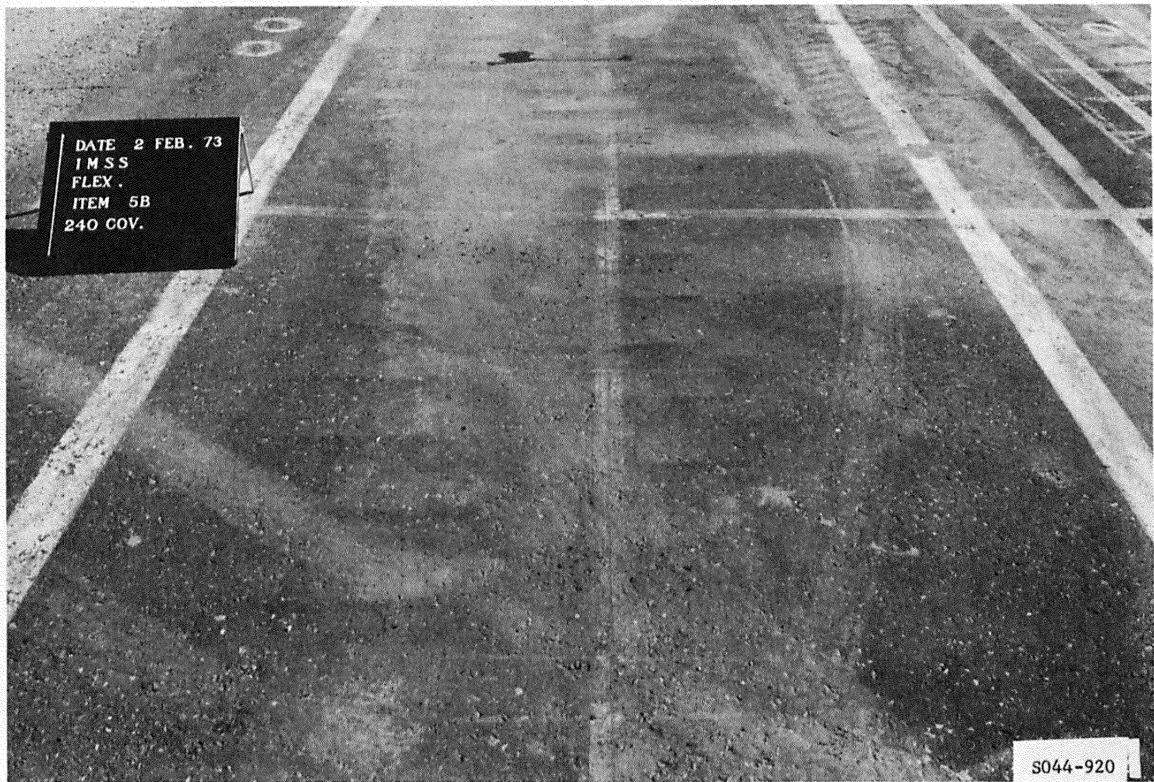
Figure B63. Subitem 5b, lane 3, flexible pavement test section, at failure after 240 coverages of 50-kip single-wheel assembly
