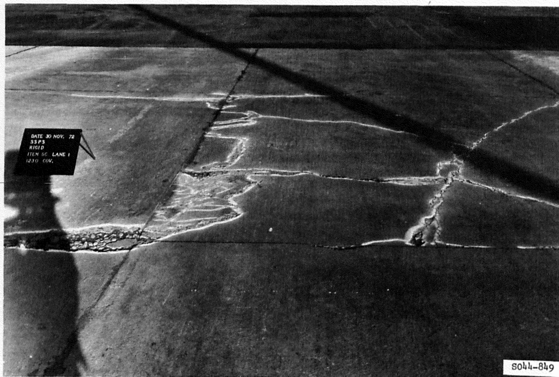
Figure A28. Subitem 5c, lane 1, rigid pavement test section, after 1230 coverages by 200-kip twin-tandem assembly
