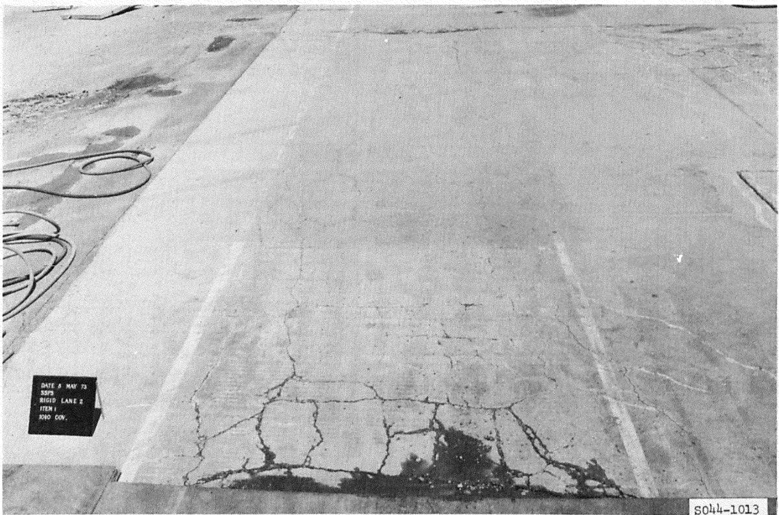
Figure A34. Item 1, lane 2, rigid pavement test section, after 1010 coverages by 240-kip twin-tandem assembly
