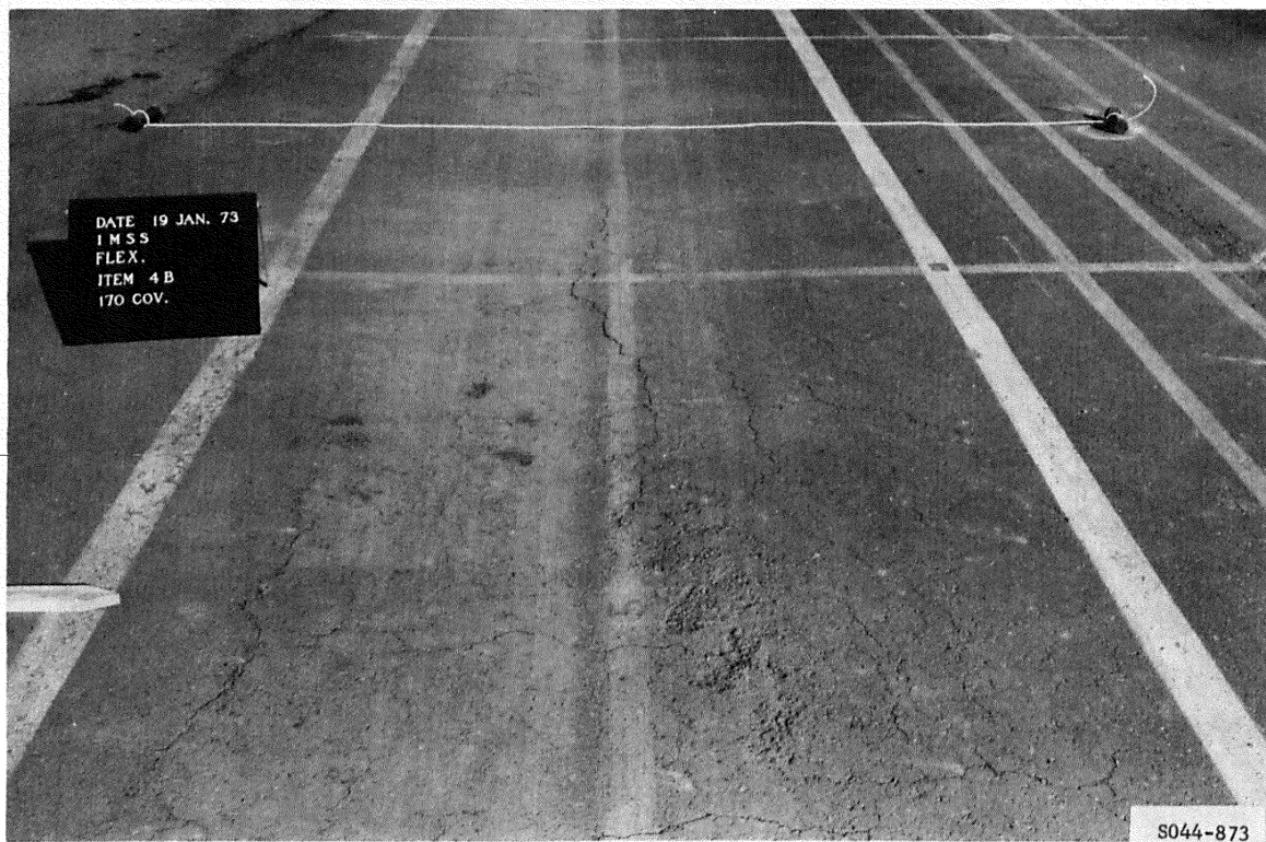
Figure B54. Cracking and deformation in subitem 4b, lane 3, flexible pavement test section, at failure after 170 coverages of 50-kip single-wheel assembly
