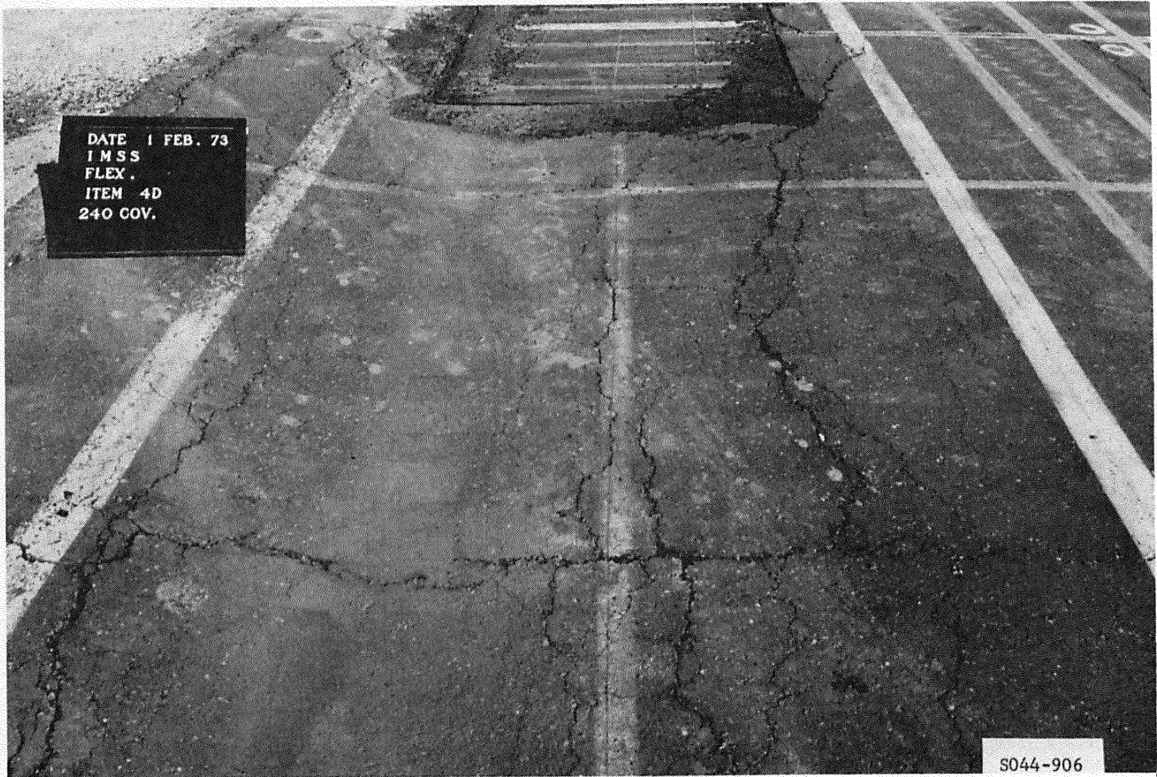
Figure B59. Cracking in subitem 4d, lane 3, flexible pavement test section, at failure after 240 coverages of 50-kip single-wheel assembly
