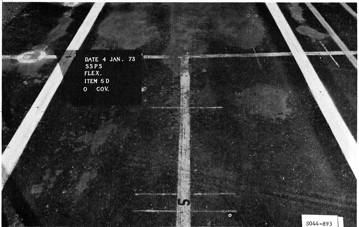
Figure B66. Subitem 5d, lane 3, flexible pavement test section, prior to traffic
