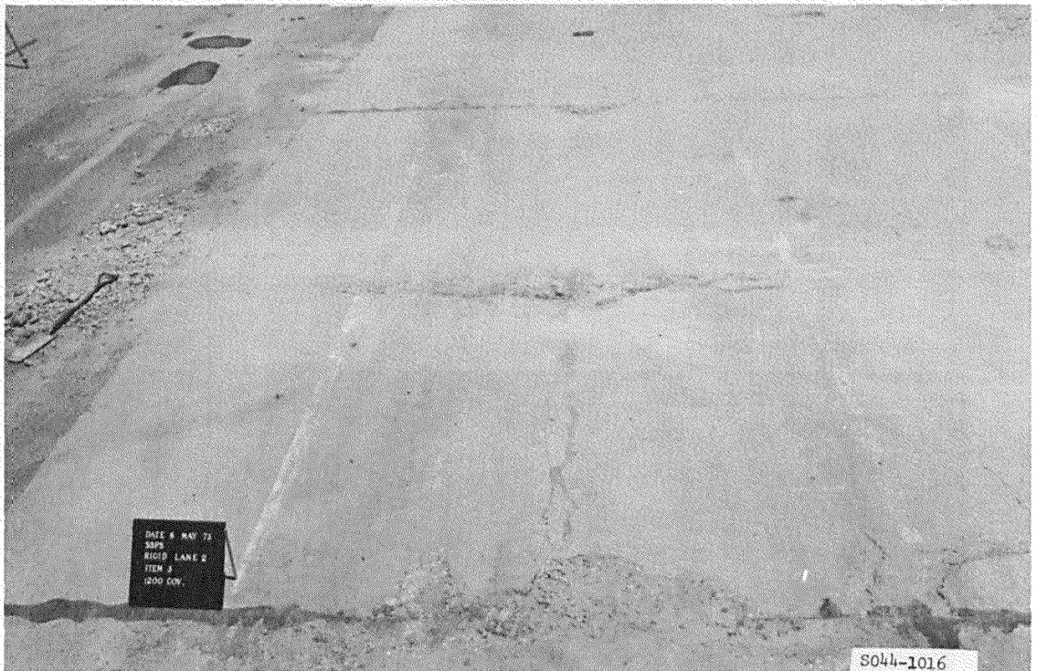
Figure A42. Item 3, lane 2, rigid pavement test section, after 1200 coverages by 240-kip twin-tandem assembly
