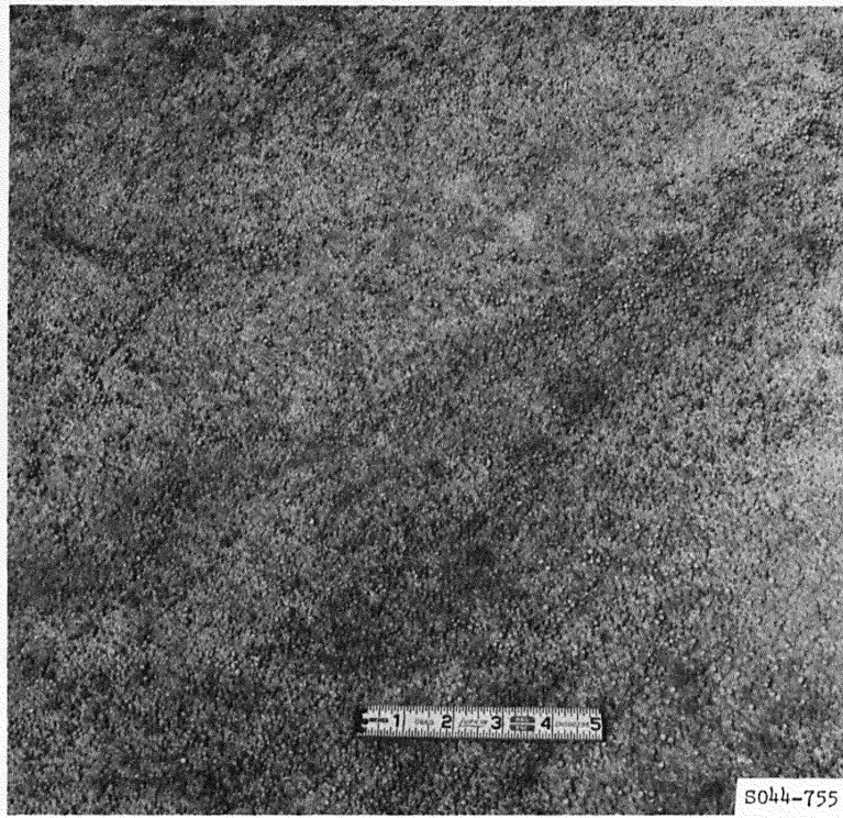
Figure 29. Surface texture of the lightweight concrete insulating layer in subitem 5b of the rigid pavement test section
