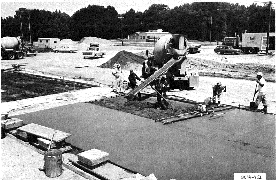
Figure 32. Placement of fibrous-reinforced concrete over insulating materials in item 2 of the rigid pavement test section
