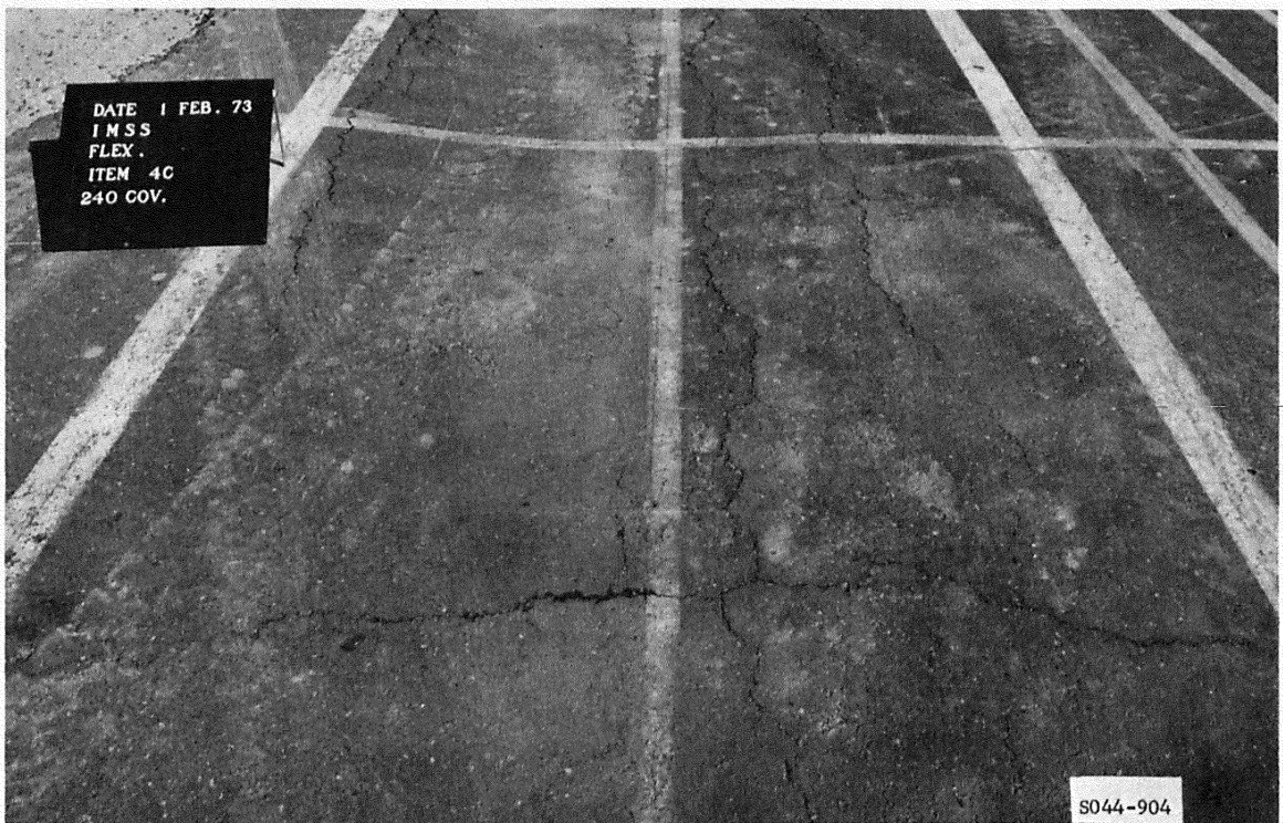
Figure B56. Cracking in subitem 4c, lane 3, flexible pavement test section, at failure after 240 coverages of 50-kip single-wheel assembly
