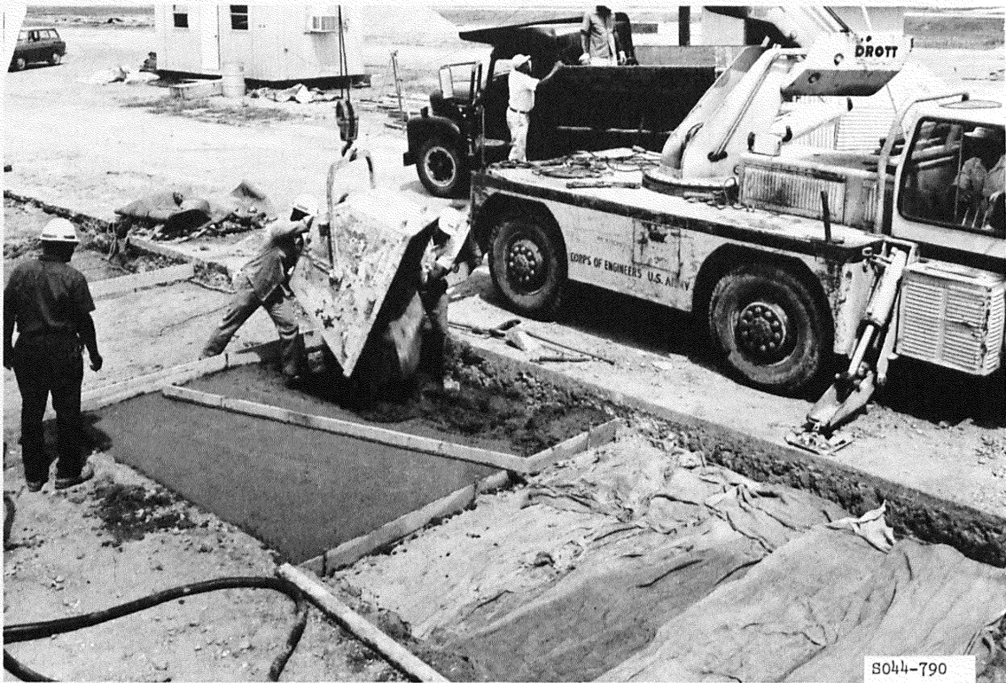
Figure 38. Placement of lightweight concrete insulating materials in item 5 of the flexible pavement test section
