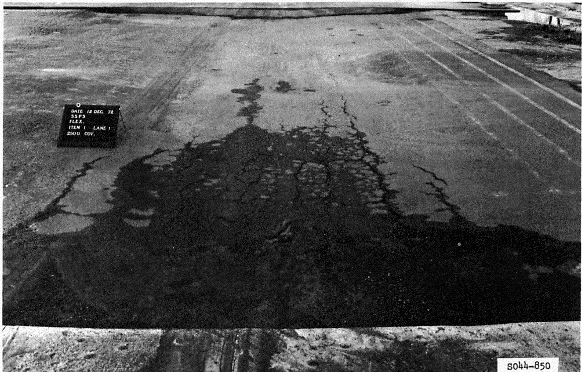
Figure B2. Cracking in western quarter of item 1, lane 1, flexible pavement test section, at 2500 coverages of 200-kip twin-tandem assembly
