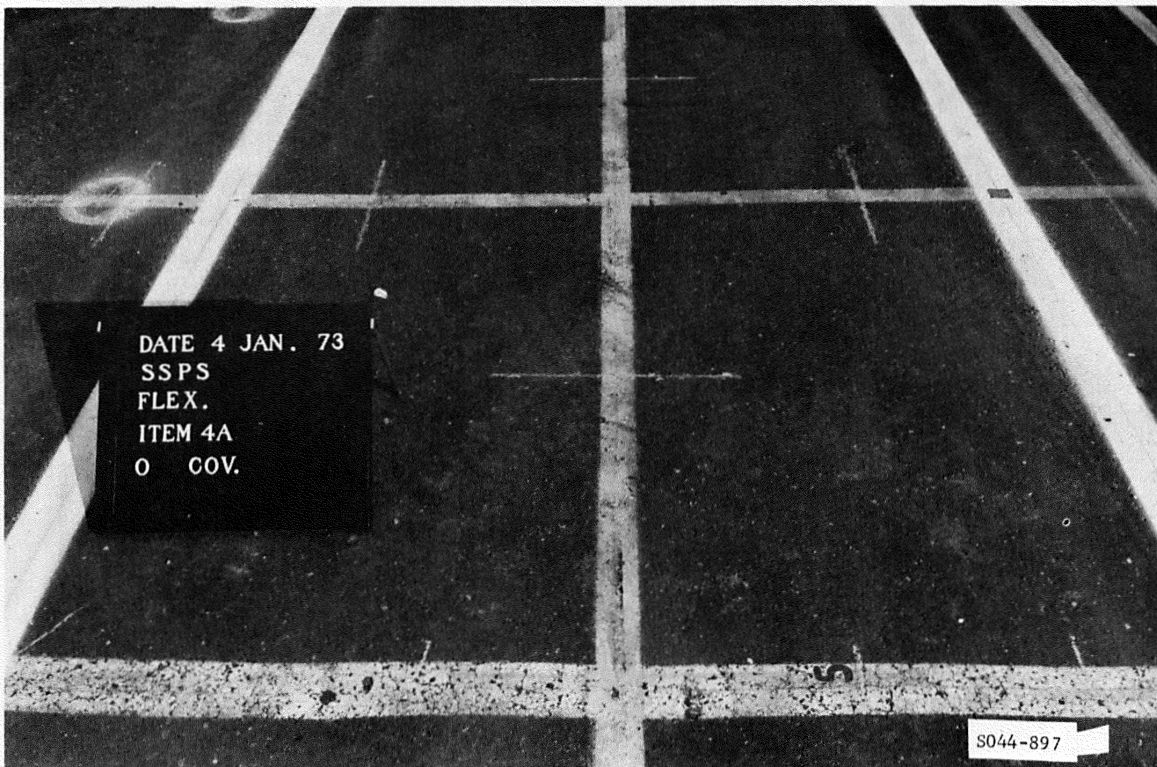
Figure B51. Subitem 4a, lane 3, flexible pavement test section, prior to traffic
