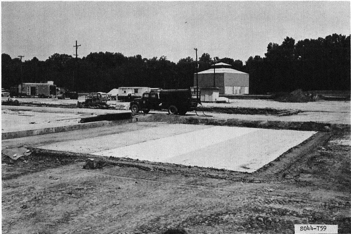
Figure 30. Completed installation of insulating materials on subgrade of subitems 5a-d of the rigid pavement test section
