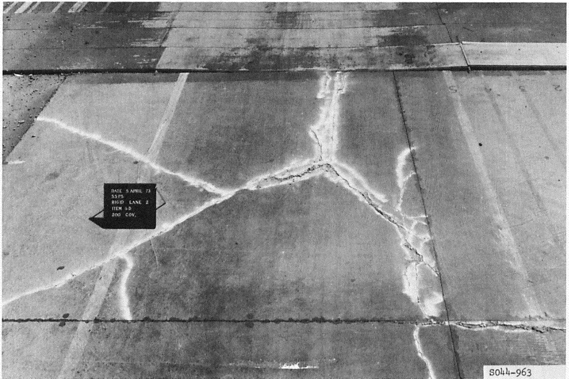
Figure A56. Subitem 5d, lane 2, rigid pavement test section, after 200 coverages by 240-kip twin-tandem assembly
