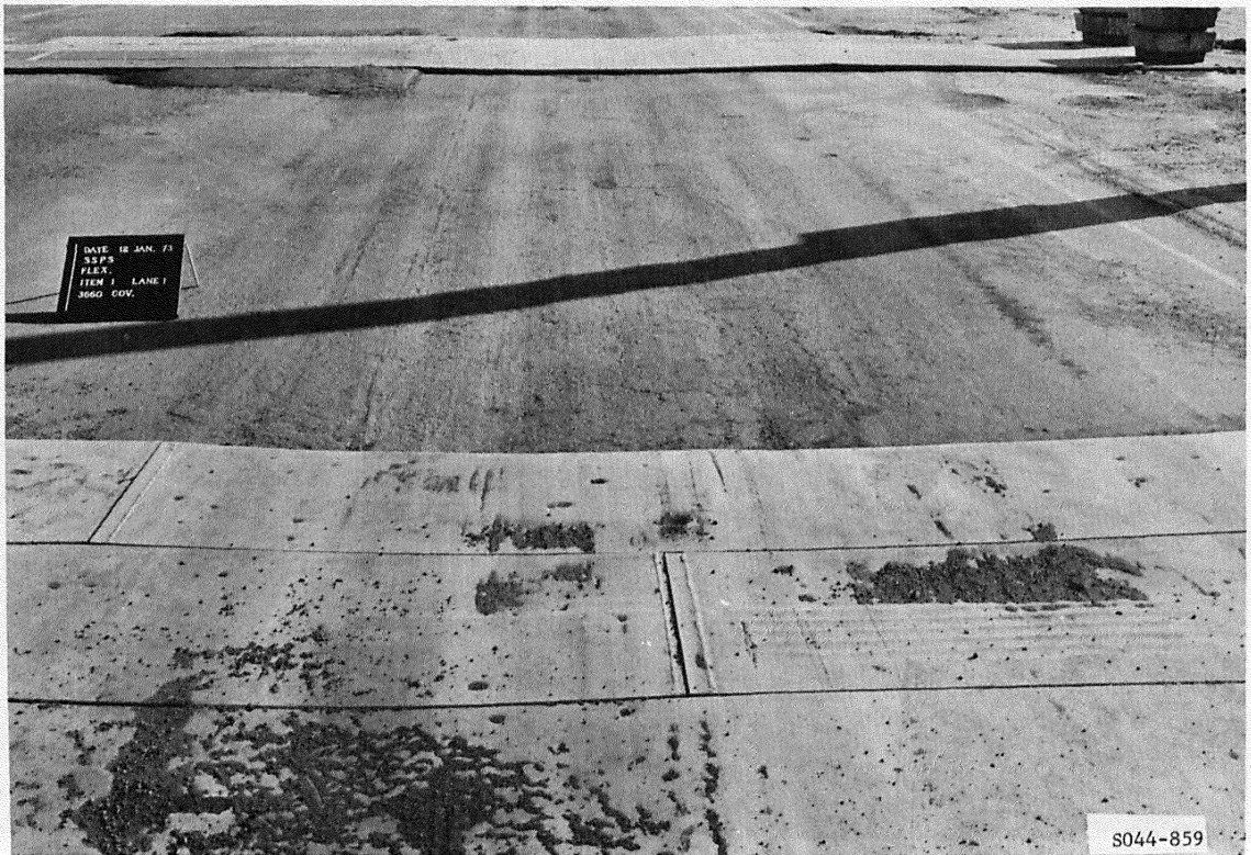
Figure B3. Cracking in eastern three-fourths of item 1, lane 1, flexible pavement test section, at 3660 coverages of 200-kip twin-tandem assembly
