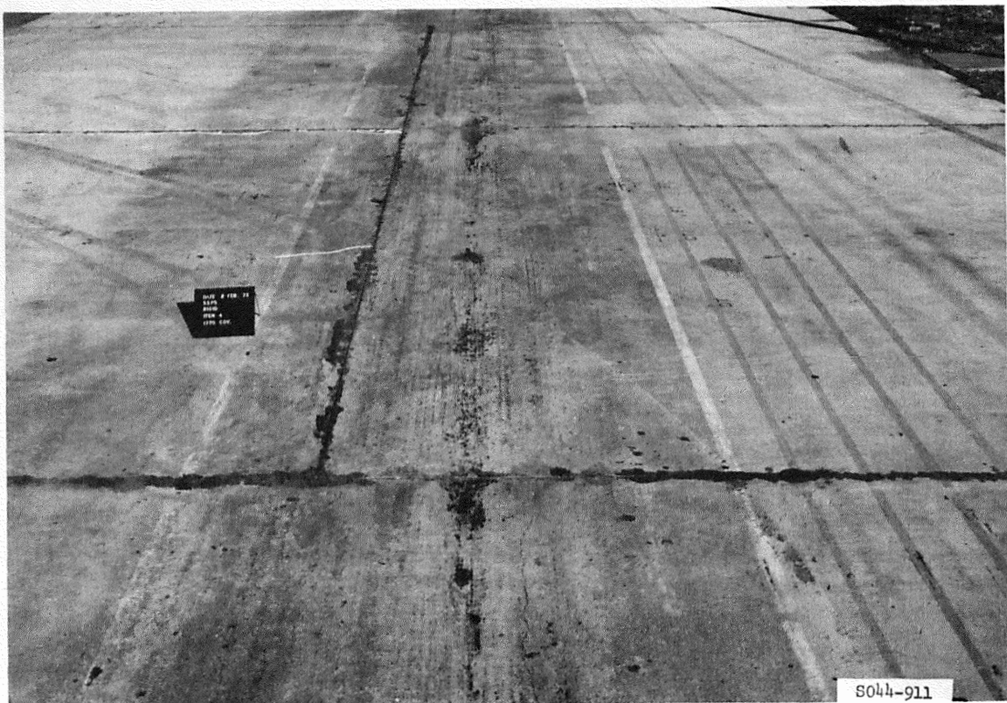
Figure A18. Item 4, lane 1, rigid pavement test section, after 1770 coverages by 200-kip twin-tandem assembly
