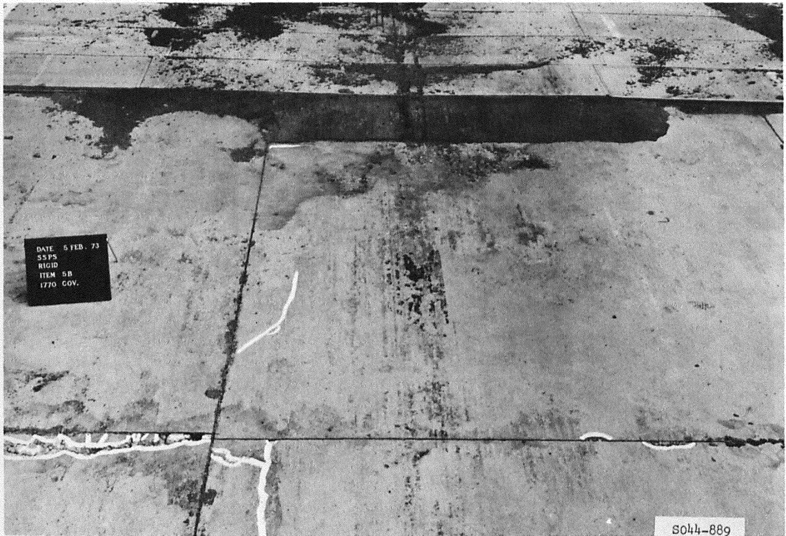
Figure A25. Subitem 5b, lane 1, rigid pavement test section, after 1770 coverages by 200-kip twin-tandem assembly
