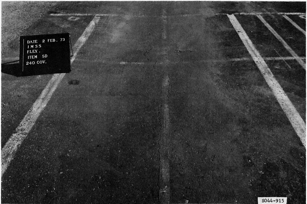
Figure B67. Cracking in subitem 5d, lane 3, flexible pavement test section, at failure after 240 coverages
