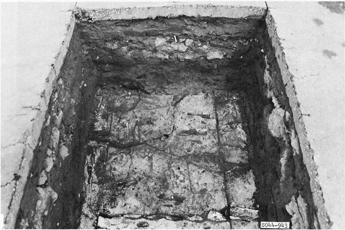
Figure B79. Cracks in polystyrene panels in subitem 4b, lane 3, flexible pavement test section, after traffic
