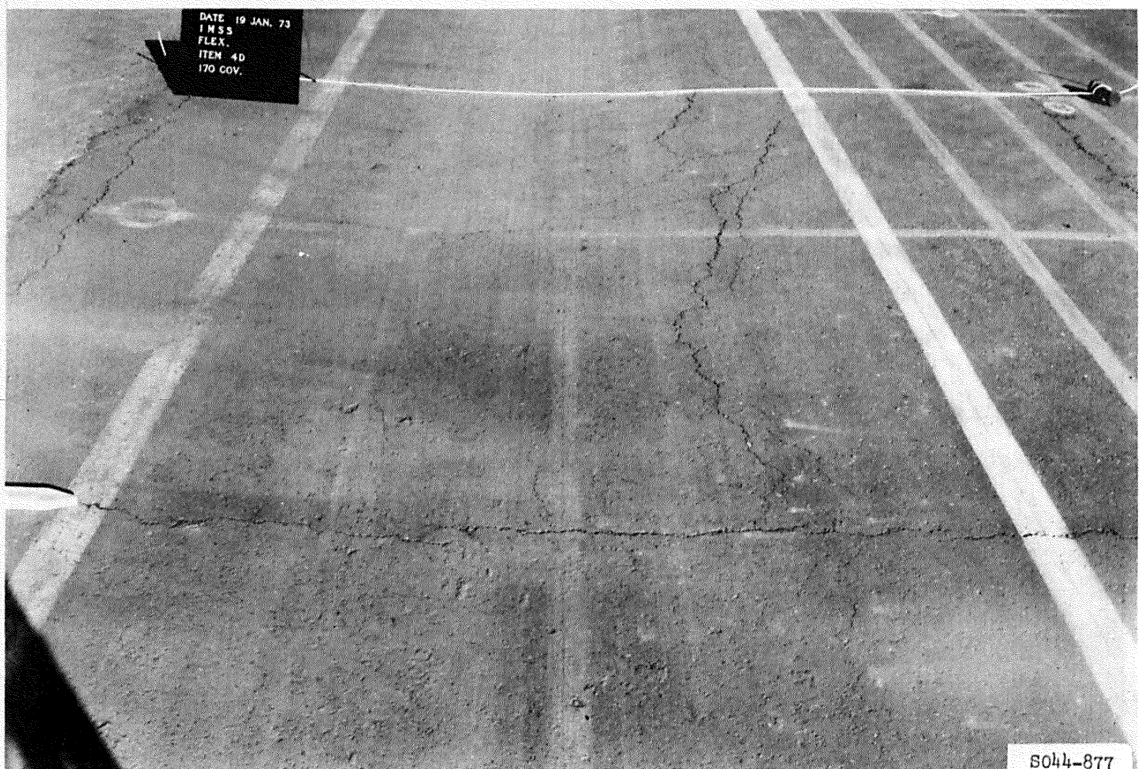
Figure B58. Cracking in subitem 4d, lane 3, flexible pavement test section, at 170 coverages of 50-kip single-wheel assembly
