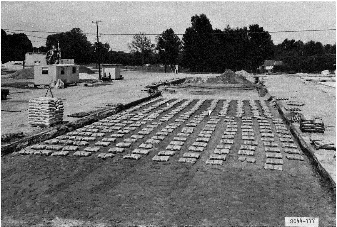
Figure 36. Bags of cement and fly ash distributed over the surface of the subgrade of items 1 and 2 of the flexible pavement test section
