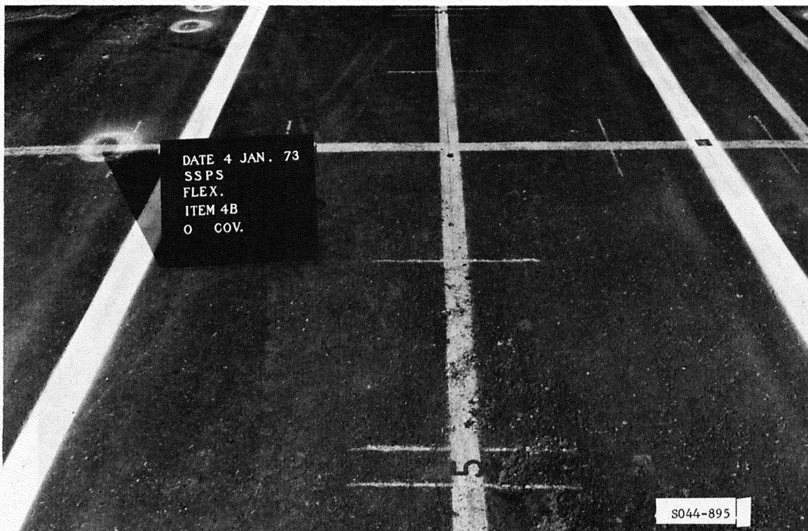
Figure B53. Subitem 4b, lane 3, flexible pavement test section, prior to traffic
