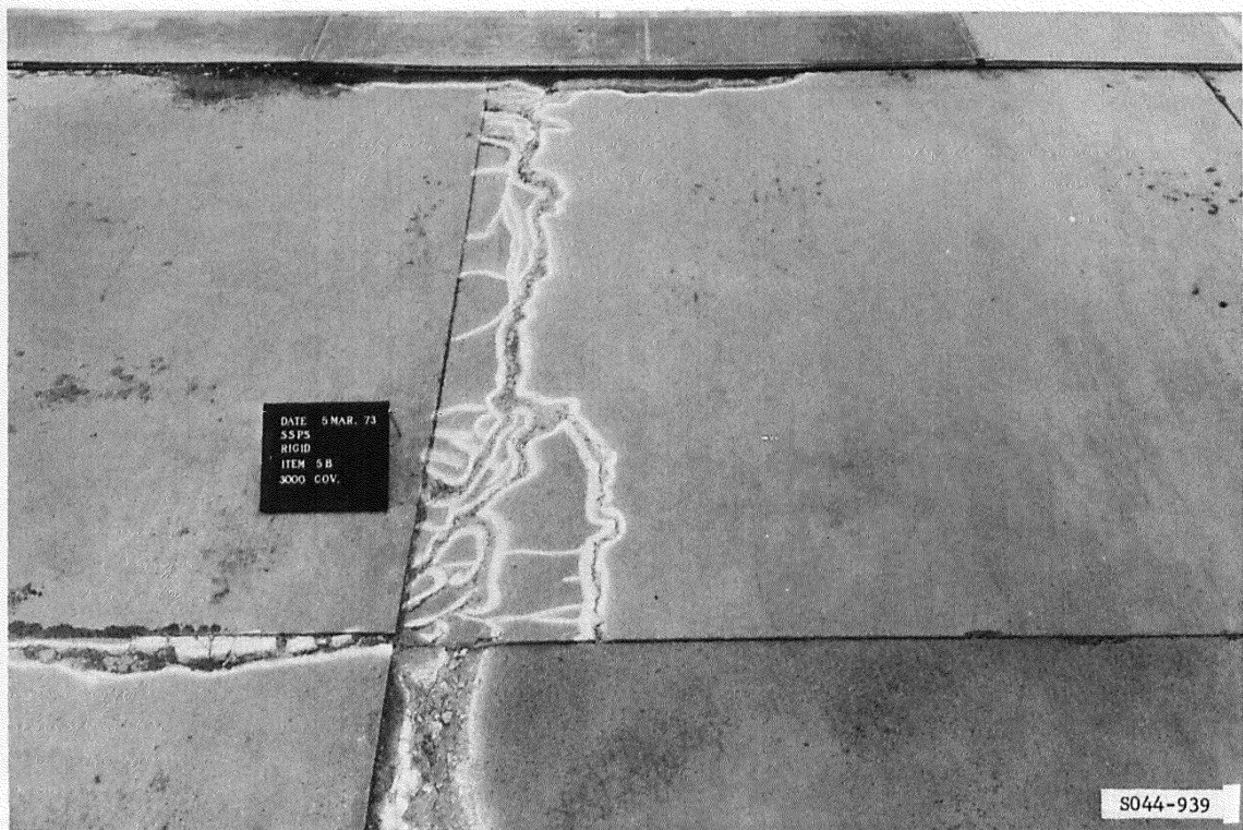
Figure A26. Subitem 5b, lane 1, rigid pavement test section, after 3000 coverages by 200-kip twin-tandem assembly
