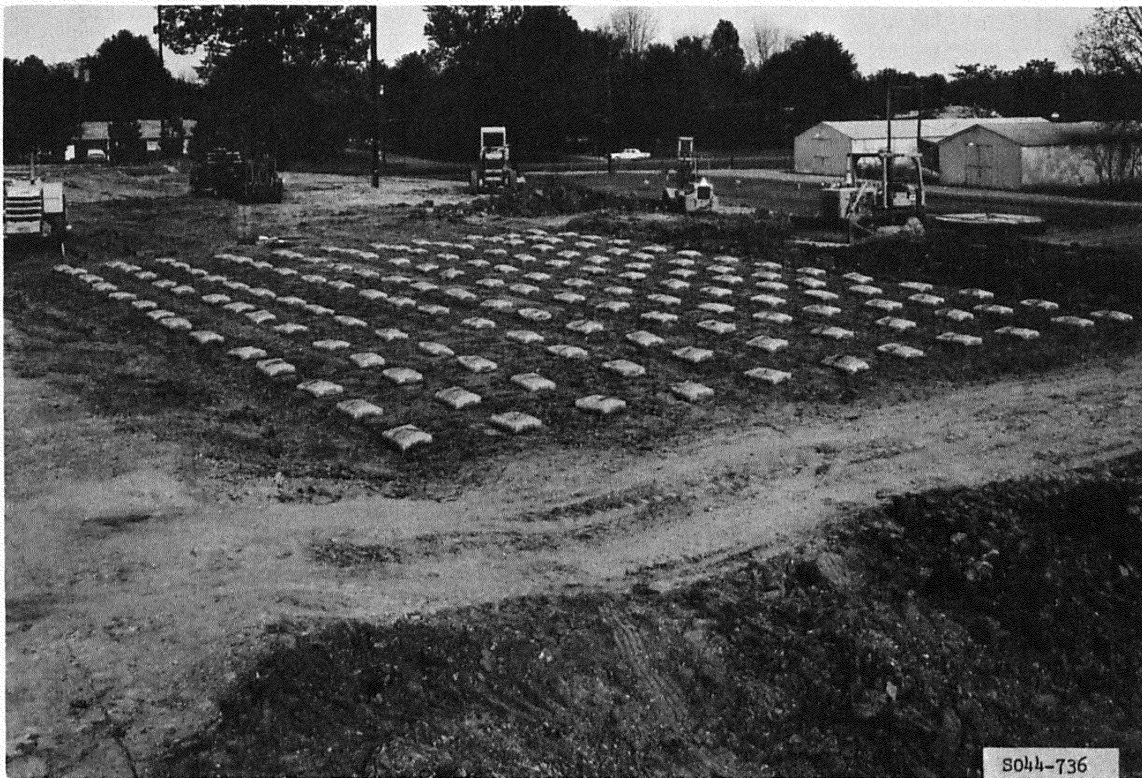
Figure 22. Bags of cement distributed over the surface of the base of item 2 of the rigid pavement test section
