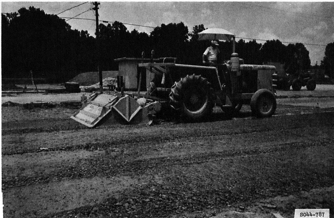
Figure 23. In-place mixing of soil and cement in item 2 of the rigid pavement test section
