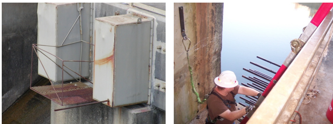
Figure 5. Failed anchor rod penetrating cover, showing one dimple in each cover indicating failed rods that did not penetrate (left); cover removed exposing anchor rods prior to testing (right).
