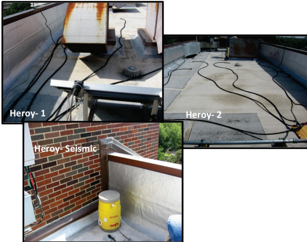
Figure 5. Photograph of the Heroy rooftop array. Highlights include the roof infrastructure, roof vents and raised edges, which could create a complex noise environment for the array. Heroy - 1 is the hose array for the infrasound sensor on channel 1 and solar panel and GPS for the Heroy array. Heroy - 2 is the hose array and manifold for the infrasound sensor on channel 2. Heroy - Seismic is the seismic sensor located under the yellow upside down drink cooler.
