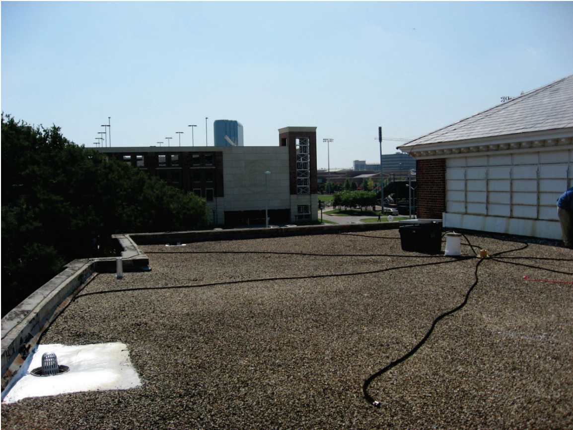
Figure A7. Multi-rooftop array at Perkins Hall.
