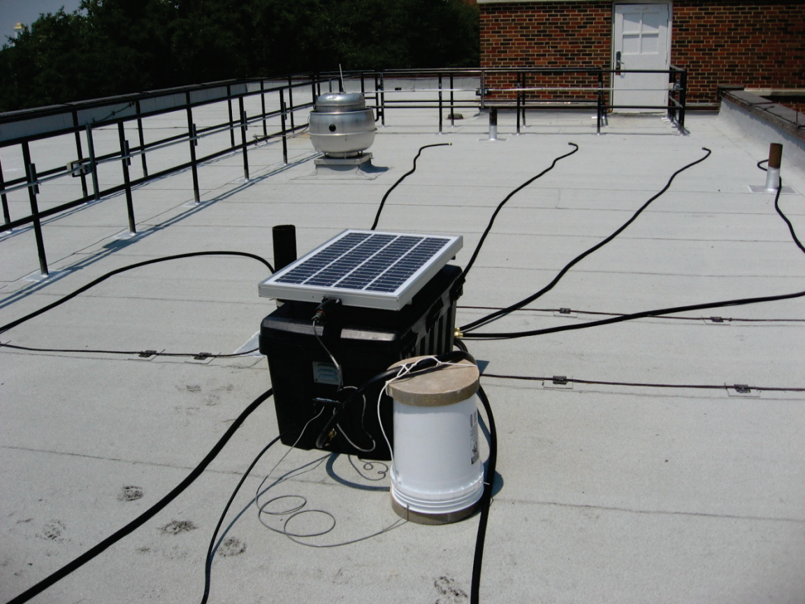
Figure A8. Multi-rooftop array at Boaz Hall.
