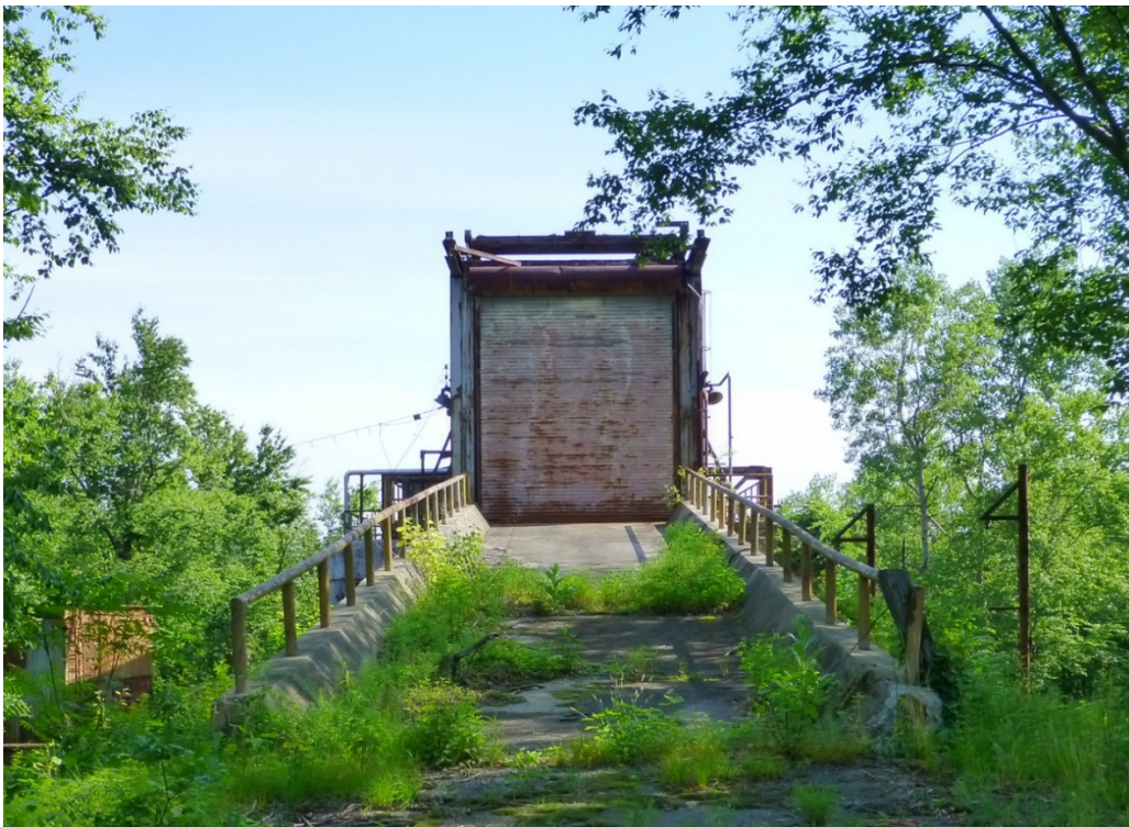
Figure 309. View of rear and southeast side of Static Rocket Test Stand (Building 3618) (ERDC-CERL, 2013).
