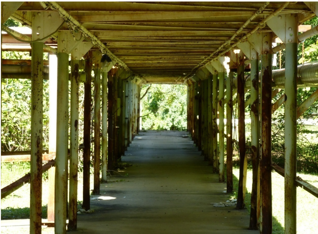
Figure 230. Covered walkways near the test stand area in the Testing Area of the historic district (ERDC-CERL, 2012).
