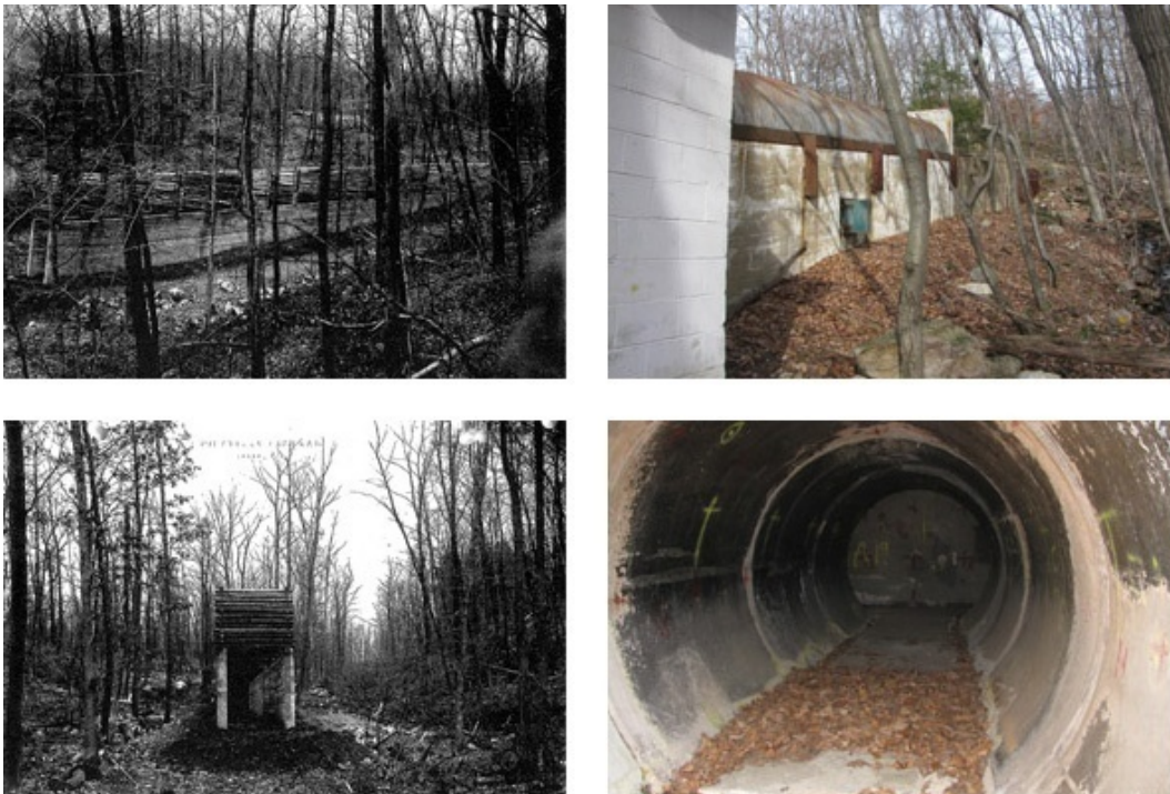
Figure 197. Comparison photographs of the original fuze test tunnel to the altered test tunnel (PICA Cultural Resources Office).
