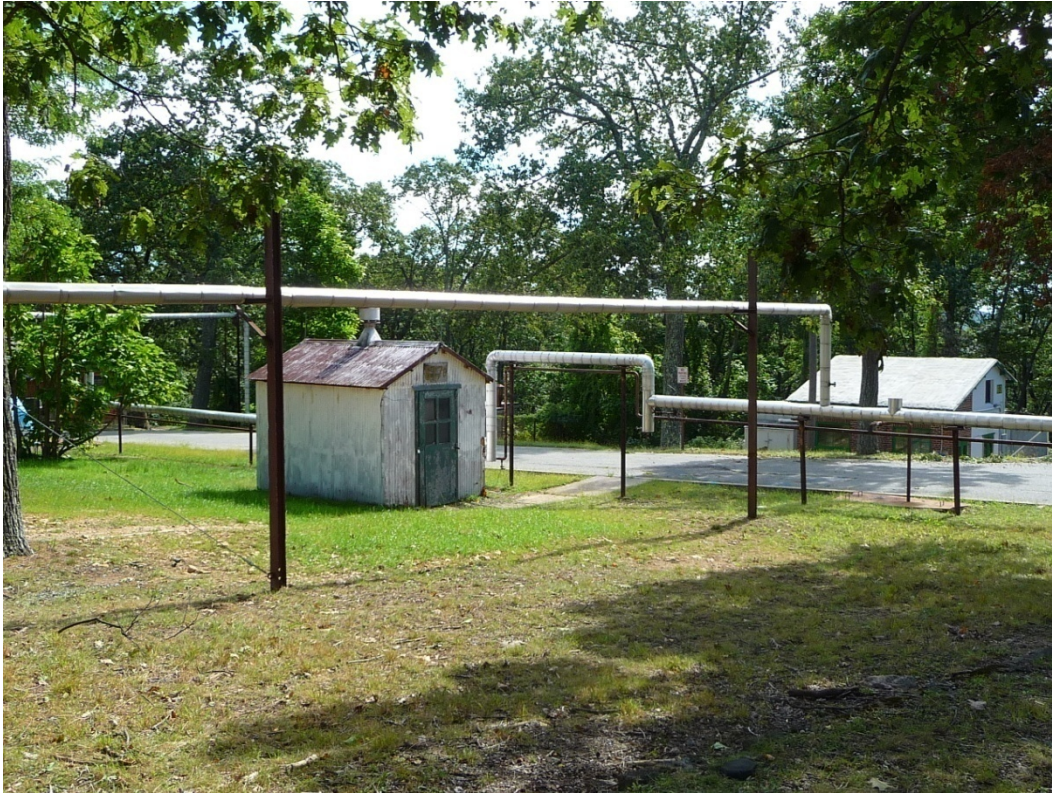
Figure 208. Steam lines located throughout the 600 Test Area (ERDC-CERL, 2012).
