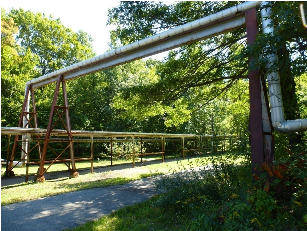
Figure 267. Steam lines supported by metal structure over the paved road (ERD-CERL, 2012).
