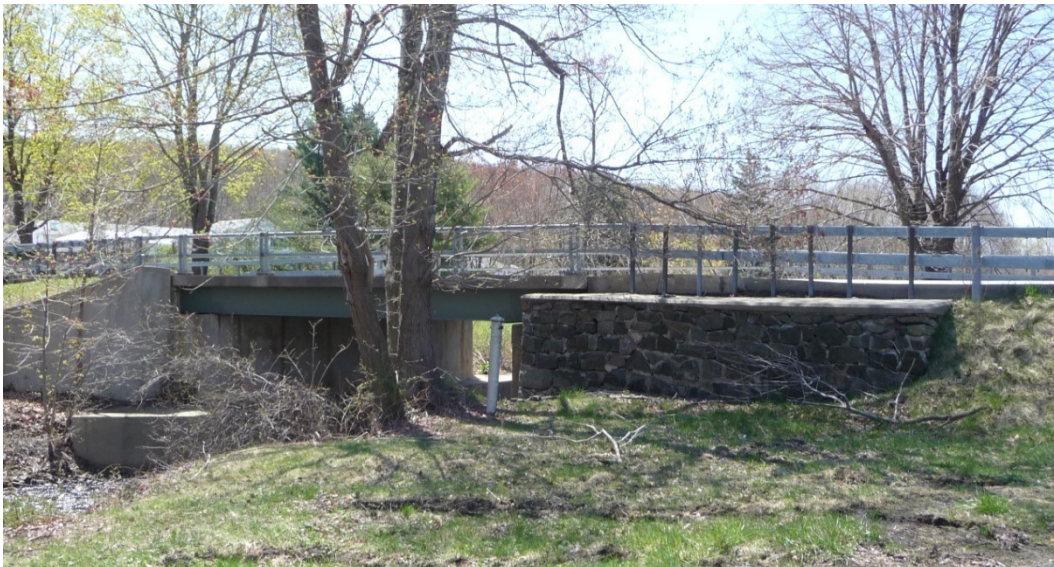
Figure 43. Current stonework for Bridge B-4; note that stonework on one side (left in this photo), has been replaced with concrete (ERDC-CERL, 2013),
