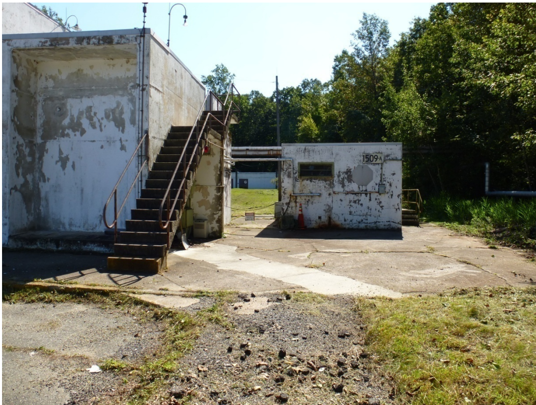
Figure 253. North elevation of Building 1509A (right), with pipes connecting it to Building 1509 (left) (ERDC-CERL, 2012).
