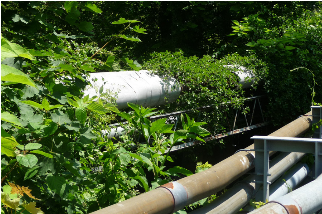
Figure 75. Steam line infrastructure, center, behind Building 151 (ERDC-CERL, 2012).
