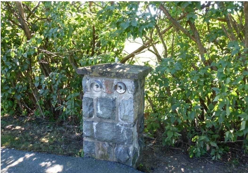
Figure 103. Garage door openers embedded in post located behind Quarters 112 and 113 (ERDC-CERL, 2012).
