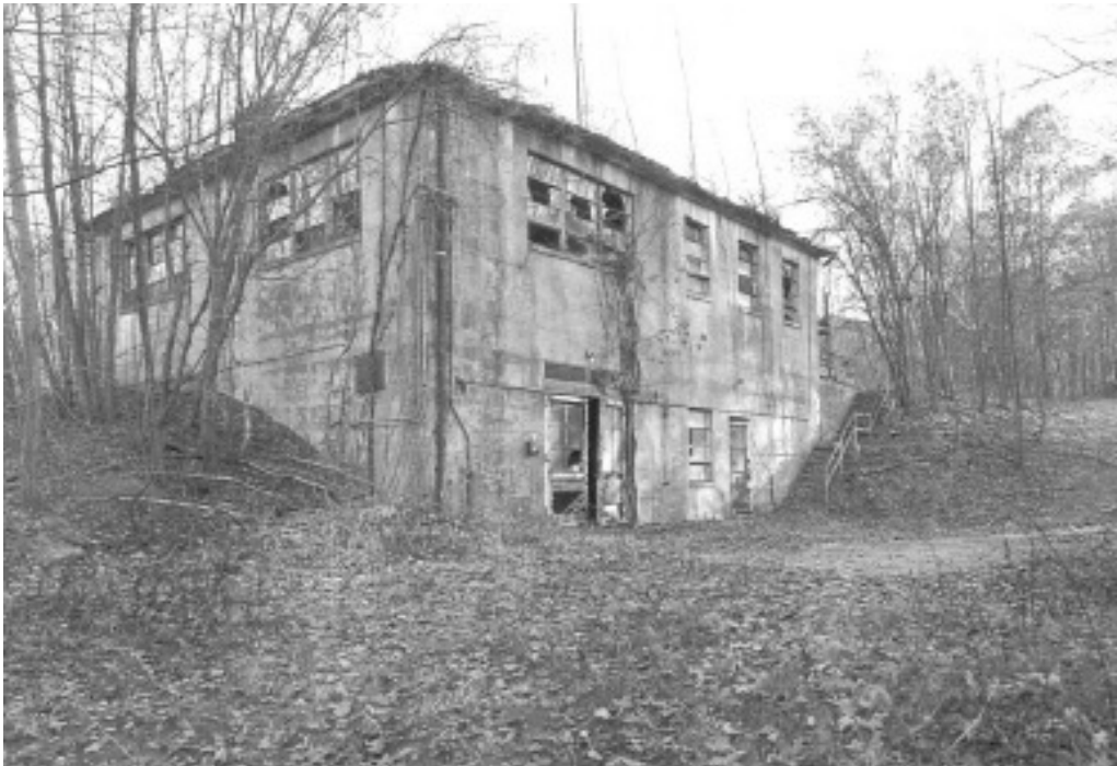
Figure 308. Oblique view of northwest and northeast elevations, Building 3617- Control House (Nolte et al. June 2009).
