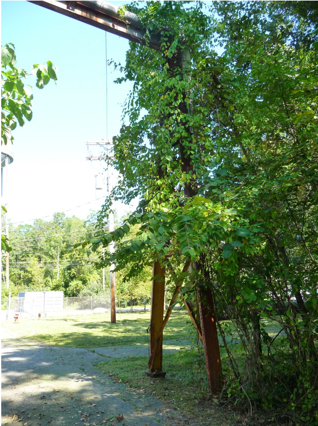
Figure 278. Overgrown vegetation on structure for steam line distribution pipes (ERDC-CERL, 2012).
