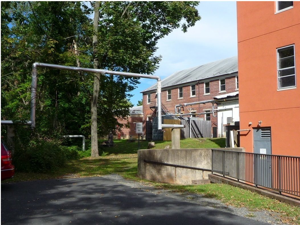
Figure 77. Steam line infrastructure behind Building 1 (ERDC-CERL, 2012).
