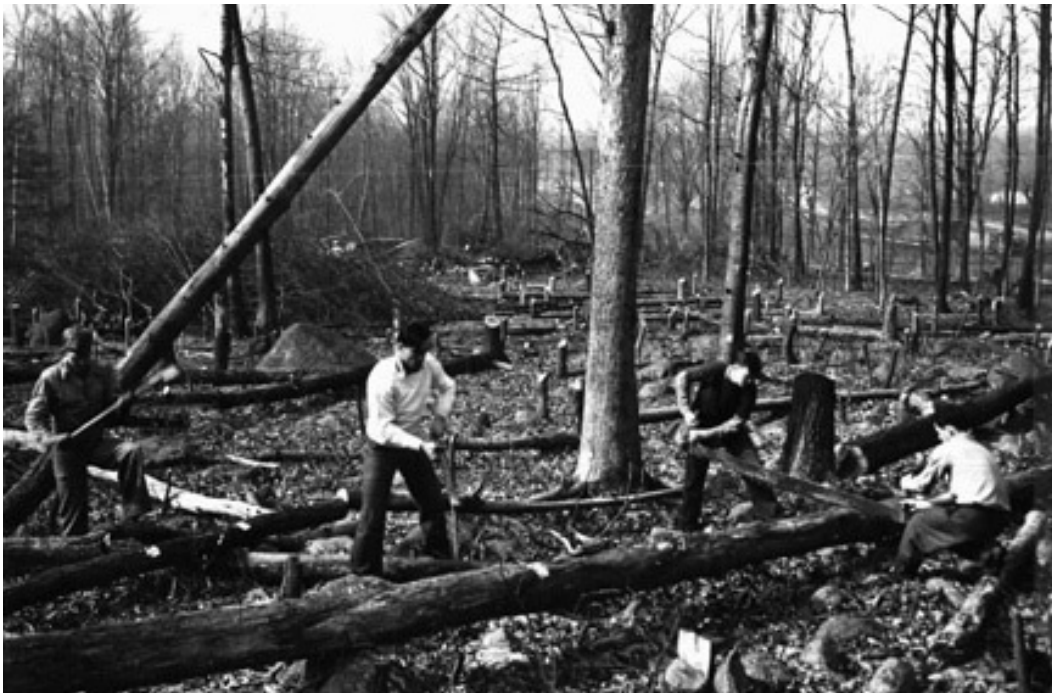
Figure 310. Historic photograph of men working to clear the land in NARTS Test Area D in preparation for building construction, January 1950 (PICA Cultural Resources Office).
