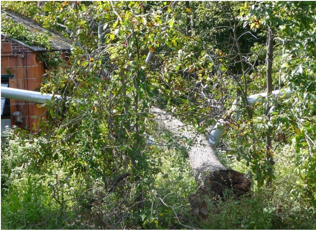
Figure 153. Fallen tree damaging elevated steam line near Building 154 (ERDC-CERL, 2012).
