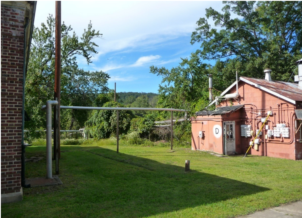
Figure 76. Steam line infrastructure between Buildings 197 and 178, which has been removed since this photo was taken (ERDC-CERL, 2012).
