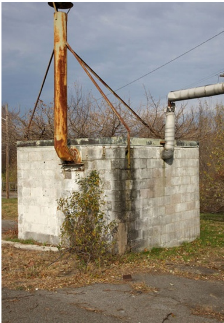
Figure 300. Southeast oblique of Building 3608, NARTS Test Area D Boiler House (PICA Cultural Resources Office, 2010).
