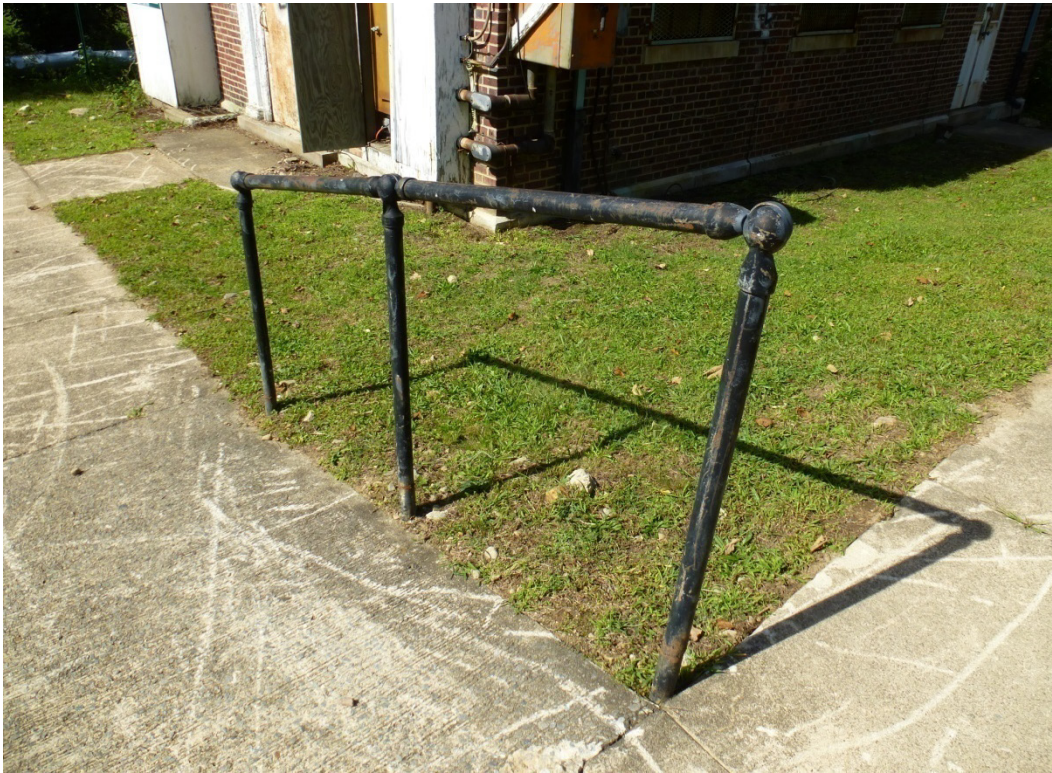
Figure 102. Original cast-iron handrails located in Chemistry Row in the Administrative and Research Historic District (ERDC-CERL, 2012).
