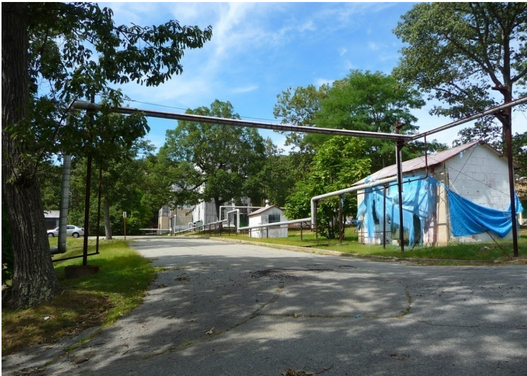
Figure 209. Replacement steam lines placed high above the paved roads in the 600 Test Area (ERDC-CERL, 2012).
