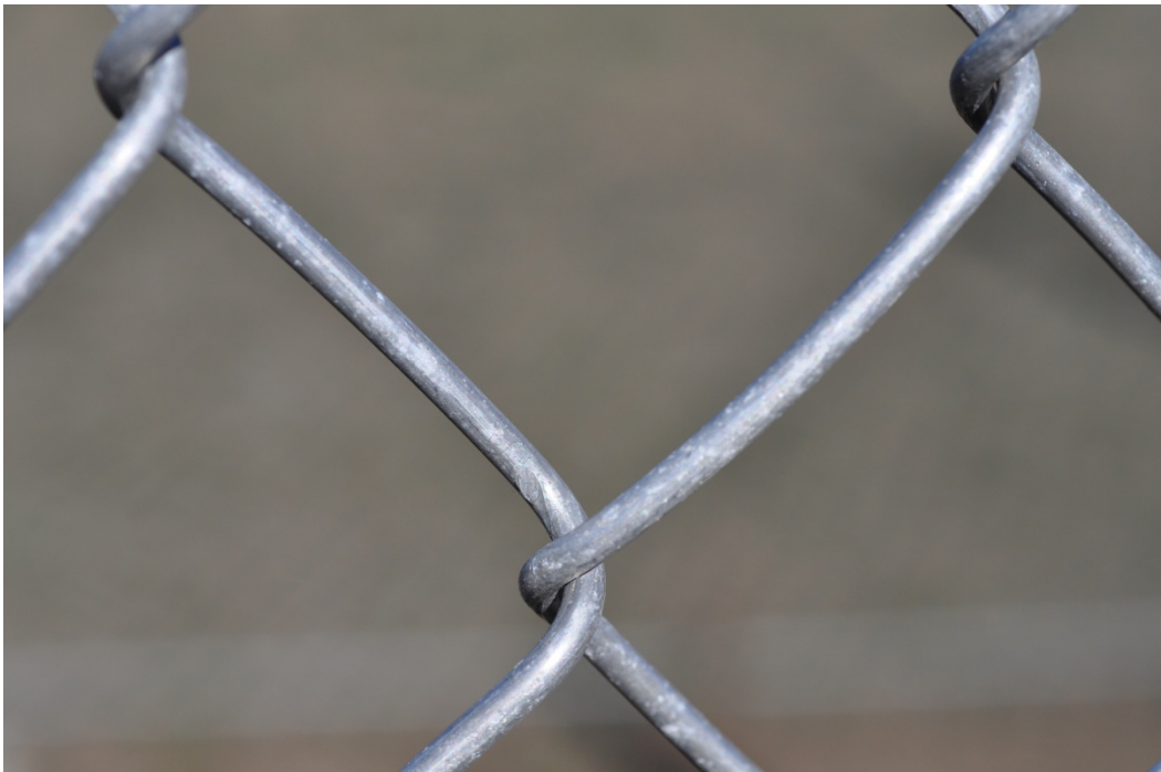
Figure A8. Stainless steel after 6 months exposure.
