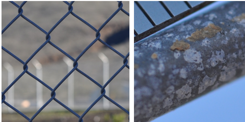
Figure A16. Galvan showing localized corrosion on 10% of its total surface after 12 months exposure.
