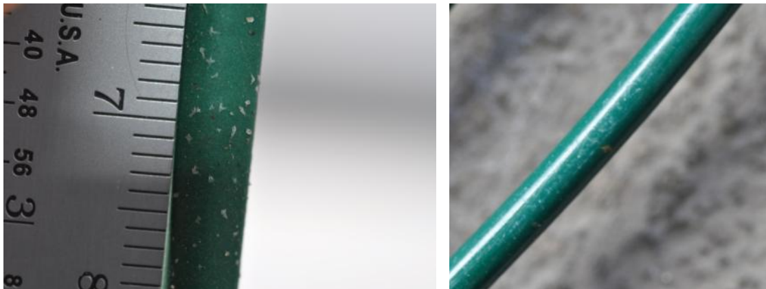
Figure 22. Standard PVC coated galvanized steel wire coupon at FRF (left) and KTA (right) after 12 months of exposure.
