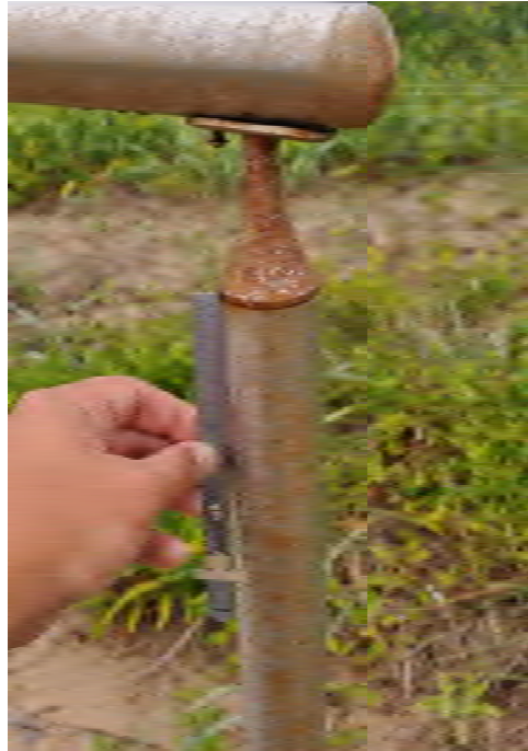
Figure B6. Stainless Steel T-fittings on fabricated railings
