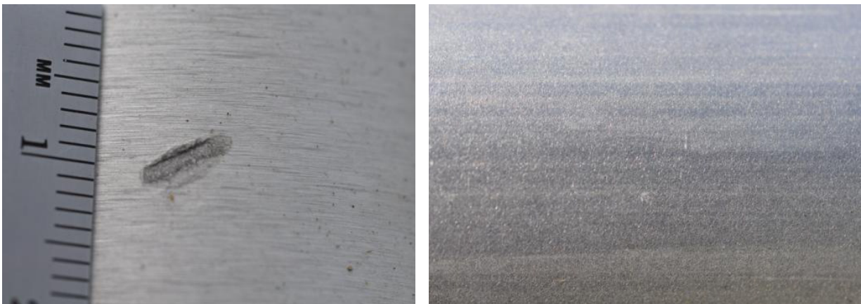
Figure 36. Aluminum railing coupon at FRF (left) and KTA (right) after 12 months of exposure.
