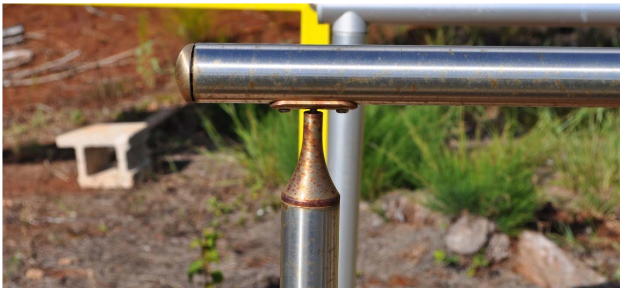
Figure B82. Stainless Steel T-fittings on fabricated railings
