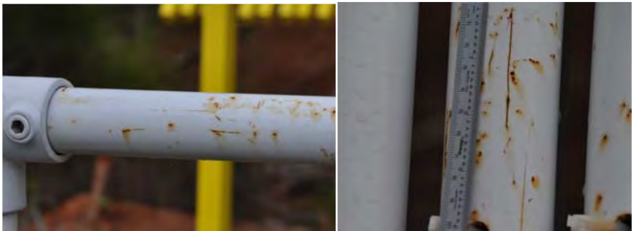
Figure B67. (Left) Painted carbon steel railing coating failure. (Right) Painted carbon steel coupon coating failure.
