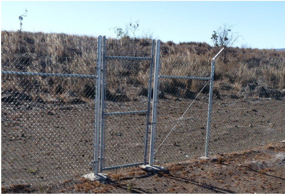
Figure A4. Personnel gate with three rows of barbed wire and locking hardware.
