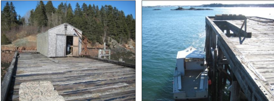
Figure 3. Treat Island weathering station wharf, view toward location of exposure racks and weather station (left) and end of wharf showing access stairway (right).
