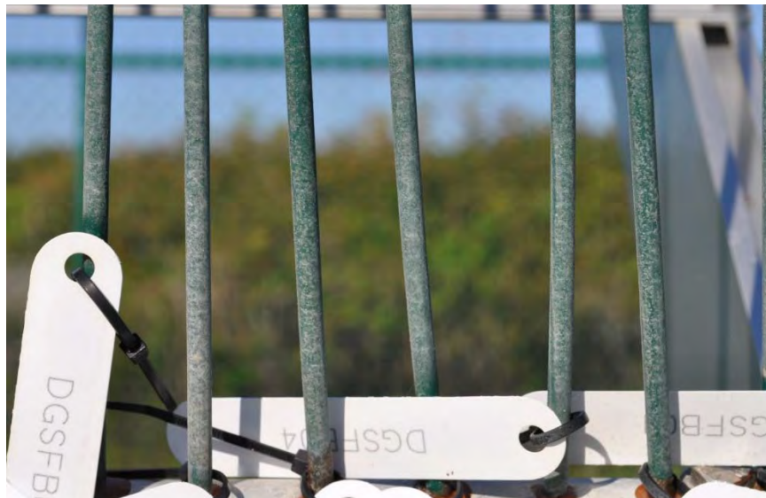
Figure B34. Fuse Bonded PVC Coated Galvanized Wire Coupon
