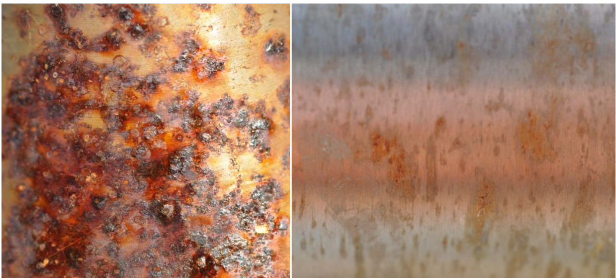
Figure B102. Stainless Steel T-fittings on fabricated railings
