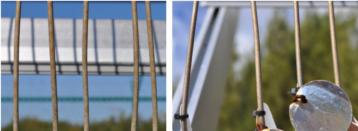
Figure 20. Stainless steel wire coupon at FRF (left) and KTA (right) after 6 months of exposure.
