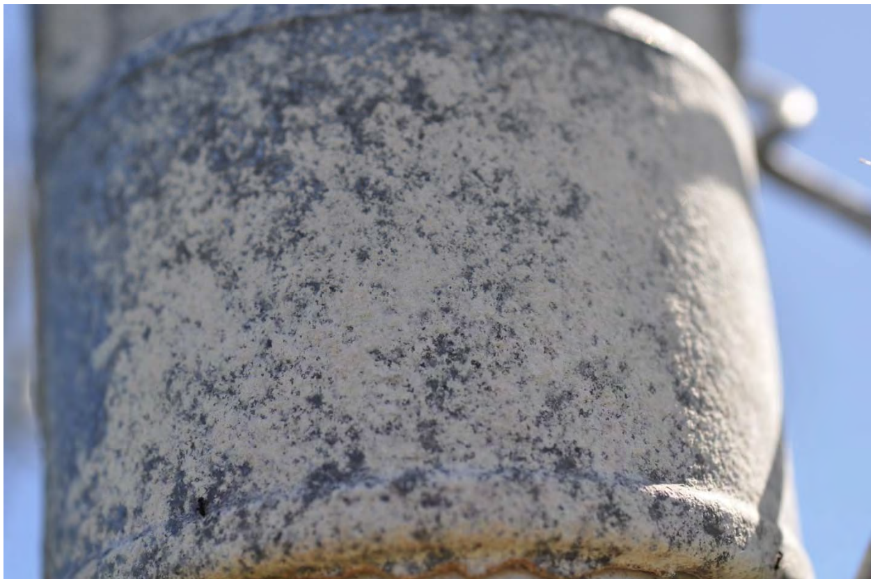
Figure B137. Galvanized Fencing Hardware
