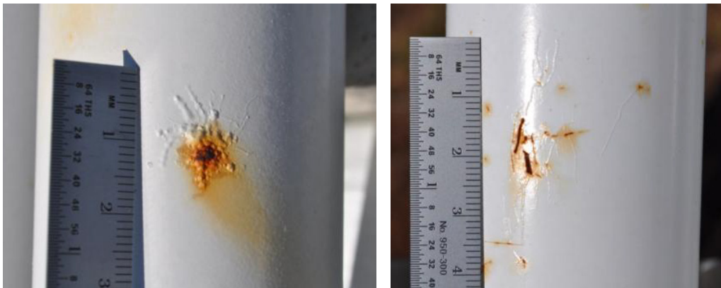
Figure 30. Coated steel railing coupon at FRF (left) and KTA (right) after 6 months of exposure.
