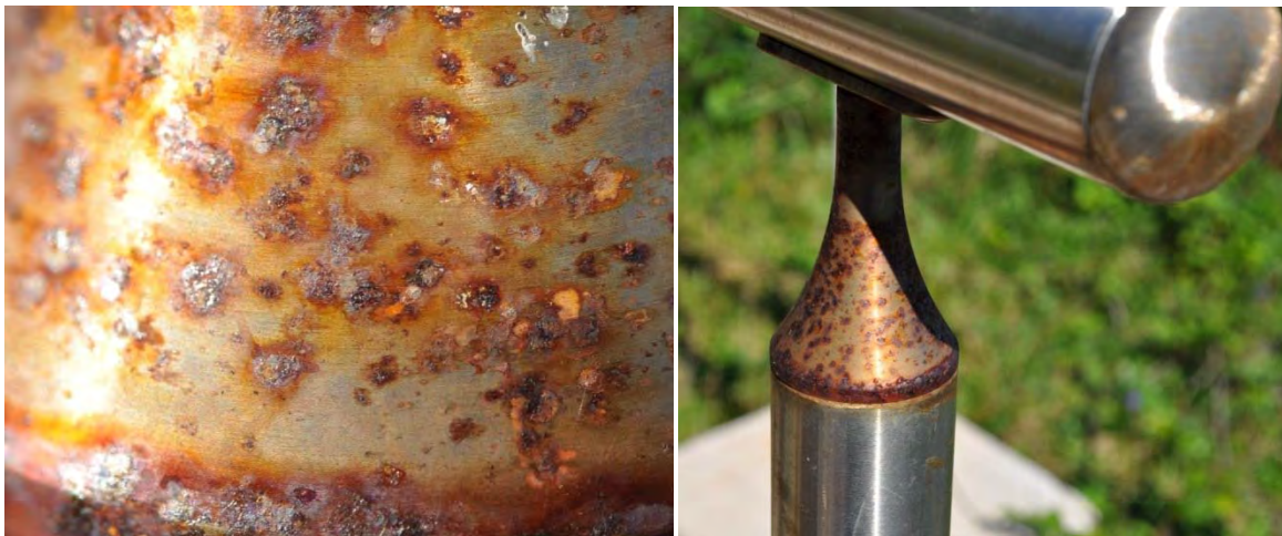
Figure B122. Stainless Steel T-fittings on fabricated railings
