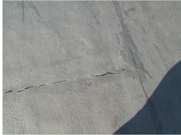
DS-L-1: Seam is open less than 1/2 inch.
