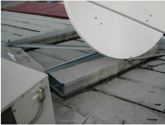
EQ-L-1: All improper equipment supports are rated low severity as a minimum due to the maintenance problems.
