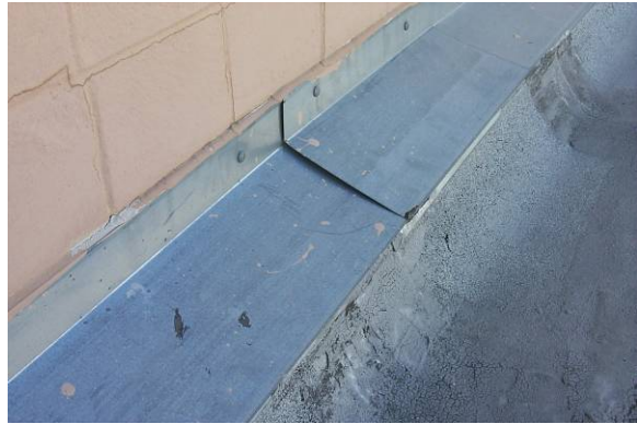
MC-M-2: Metal coping cap has loose fasteners, failure of soldered or sealed joints, open joints, or loss of attachment.
