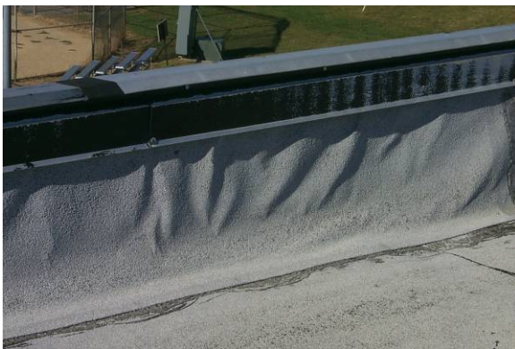
BF-M-1: Slippage, wrinkling, blistering, or pulling of base flashing material.
