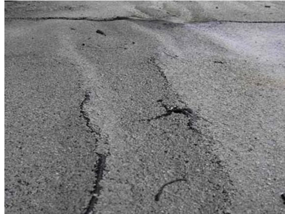
BL-H-1: The blisters are broken; there are holes, splits or tears.
