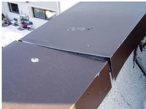
MC-H-3: Metal coping cap has missing joint covers where joint covers were originally installed.
