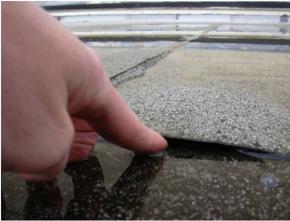
DS-L-1: Seam is open less than 1/2 inch.
