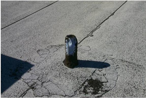
FP-L-1: Flashing sleeve is deformed.
