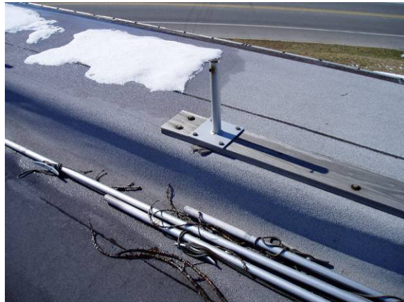
EQ-H-2: The equipment is bolted through the membrane and the bolts appear not to be sealed.
