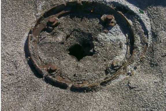
DR-L-1: Bitumen has flowed into the drain leader but the drain is not clogged. (Strainer was removed for photograph.)
