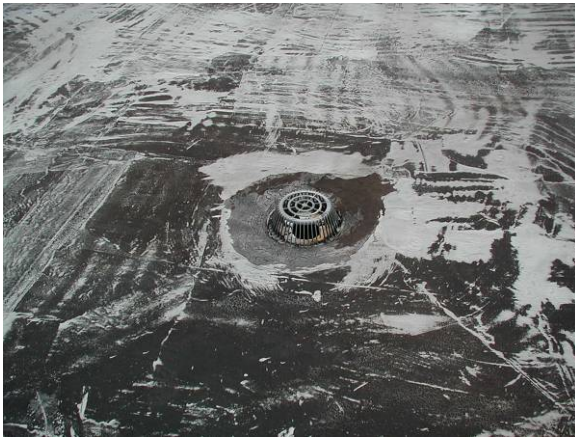
SR-L-2: On smooth liquid applied surfacing, there is loss of coating but no visible deterioration of surfacing ply.
