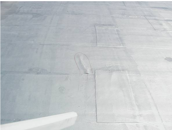
DS-H-2: Fishmouths, wrinkling, blistering or ridging at the seams that allow water to penetrate.
