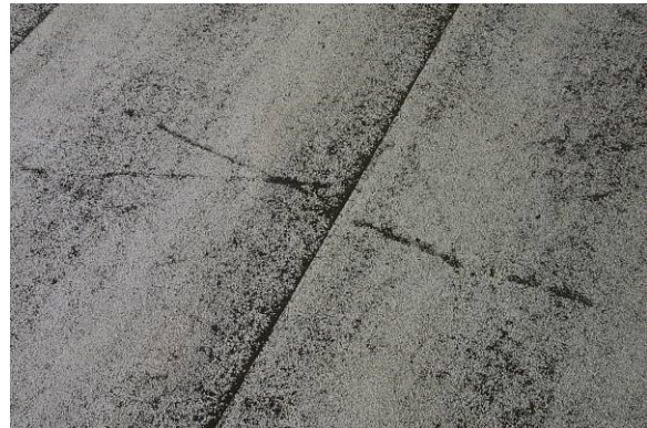
SR-M-2: On mineral surfaced capsheet surfacing, there is loss of granules, exposing the surfacing ply.
