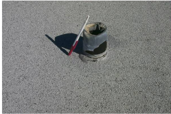
FP-L-2: Opening in the penetration or flashing is less than 6 in. above the roof surface.
