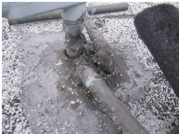
FP-H-3: No flashing sleeve is present.
