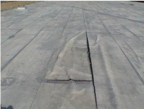
BL-M-2: Blister is beneath a seam, which has exposed unsurfaced membrane along the seam.
