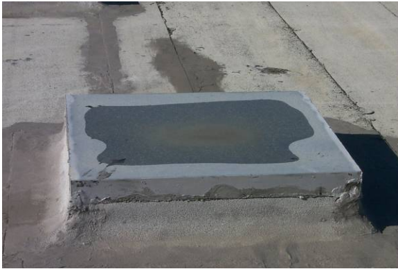
MC-L-2: Metal coping cap is deformed and allows water to pond on the top.
