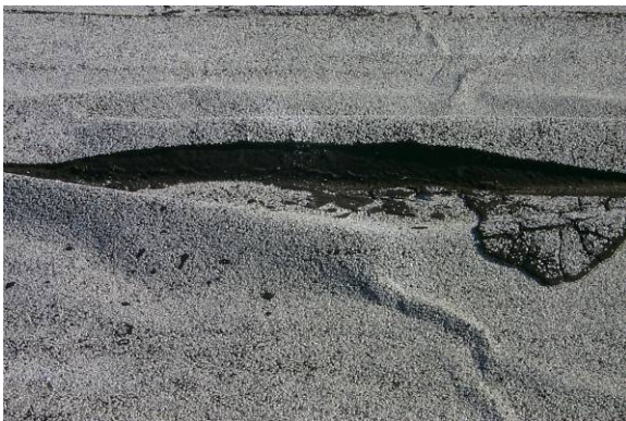
BL-H-1: The blisters are broken; there are holes, splits or tears.
