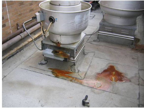
DV-M-2: Grease, solvent, or oil drippings on the roof which show no degradation of the roof membrane.
