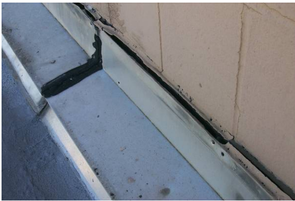
MC-M-3: Sealant at reglet or top of counterflashing is missing or no longer functioning, allowing water to channel behind.
