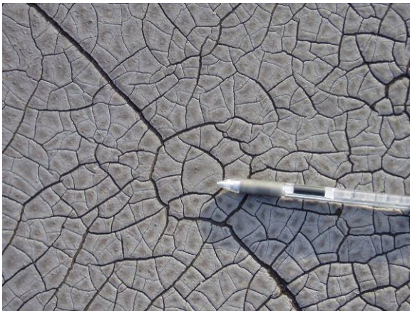
SR-M-4: On smooth liquid-applied surfacing, alligator cracks extend down through coating to the surfacing ply.
