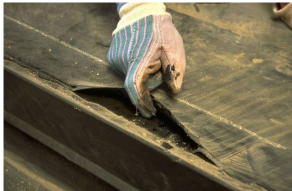
EM-H-1: Surfacing plies are missing or loose.
