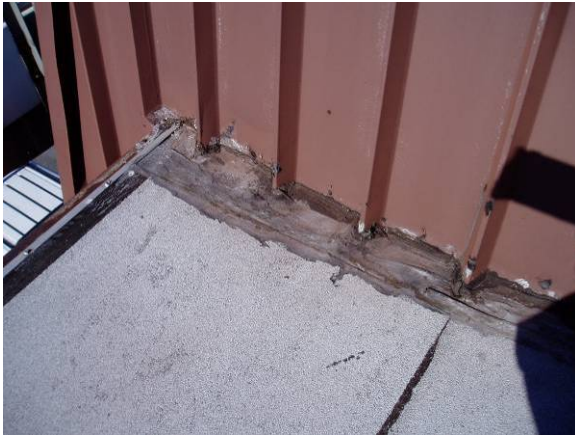
BF-H-4: No base flashing is present.
