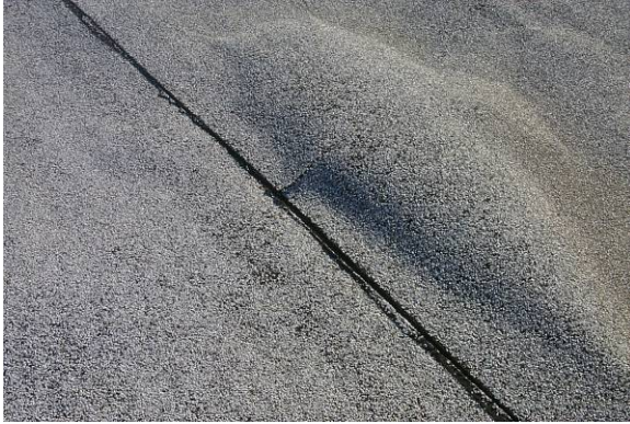
BL-L-1: The raised areas are noticeable by vision or touch. The surfacing is still in place and there is no membrane deterioration.
