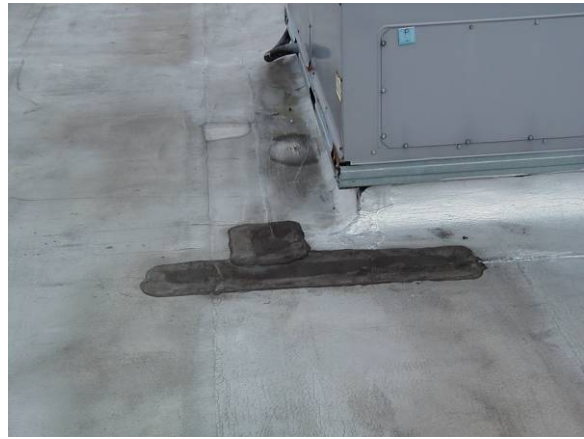
PA-M-1: The materials and workmanship of the patch are not equal to or better than the existing membrane.
