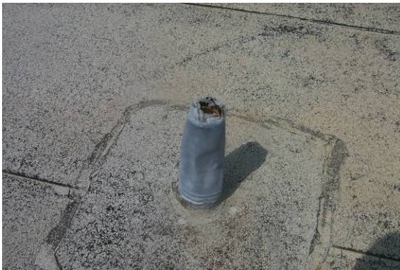
FP-M-2: Top of flashing sleeve is not sealed or has not been rolled down into an existing plumbing vent stack.
