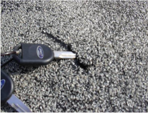
HL-H-1: All holes are considered high severity due to their high leak potential.
