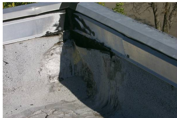
BF-H-2: Exposed gaps at the top of the base flashing that are not covered by counterflashing or open side laps in the flashing.
