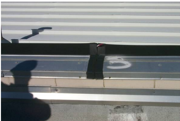
MC-H-2: Corrosion holes penetrating metal on horizontal surface or rubber bellows of an expansion joint cover.
