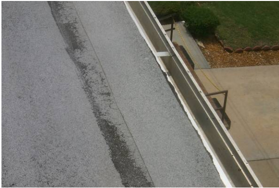
EM-L-1: The entire length of embedded edge metal flashings is rated low severity at minimum due to the maintenance problems.
