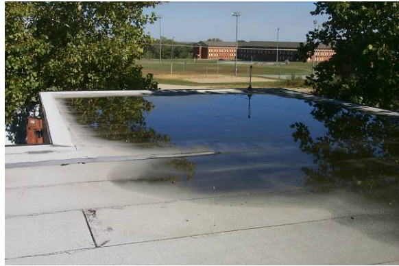
PD-L-1: Ponding is rated low severity due to the maintenance problems associated with it.
