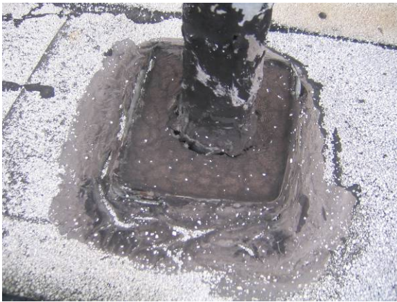
PP-H-4 : Sealing material has cracked or separated from pan or penetration.
