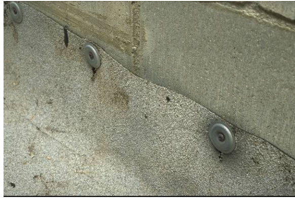
MC-H-1 : Metal coping cap or counterflashing is missing or displaced from its original position.
