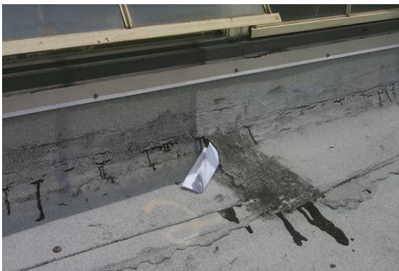
BF-H-1: Holes, splits, or tears in flashing caused by deterioration or physical damage.
