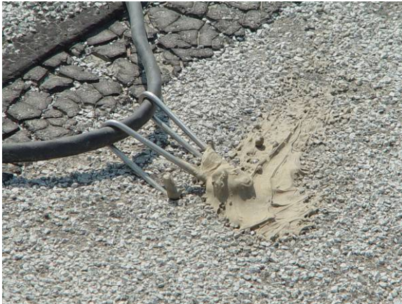
EQ-M-2: The equipment is bolted through the membrane but the bolts appear to be sealed.
