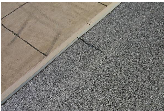
EM-H-2: Splits in the surfacing plies above the metal joints.
