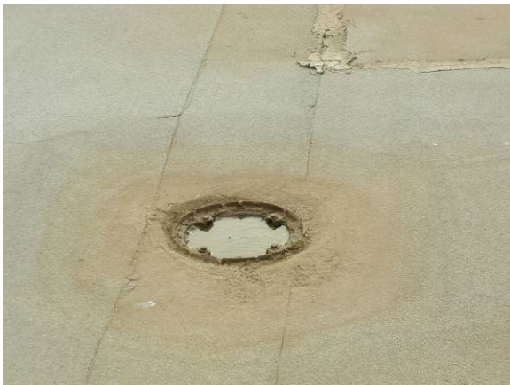
DR-H-3: Drain is clogged.
