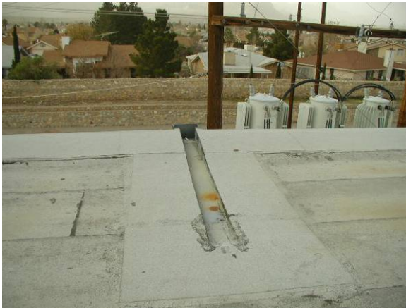
EM-M-6: Entire length of interior gutter is rated medium severity at minimum due to the maintenance problems.
