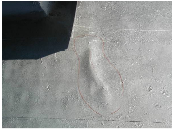
BL-L-1: The raised areas are noticeable by vision or feel. The surfacing is still in place and there is no membrane deterioration.
