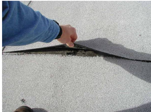
DS-H-1: Seam is open through its entire depth, allowing water to penetrate.
