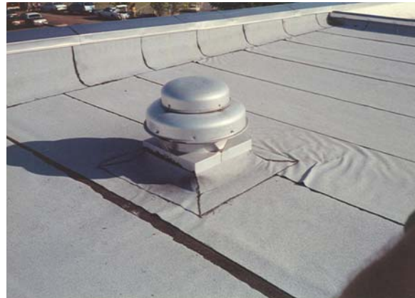
SL-H-1: More than 2 in. of slippage has occurred or the exposed bitumen has shown deterioration. There may be evidence of humping and wrinkling.
