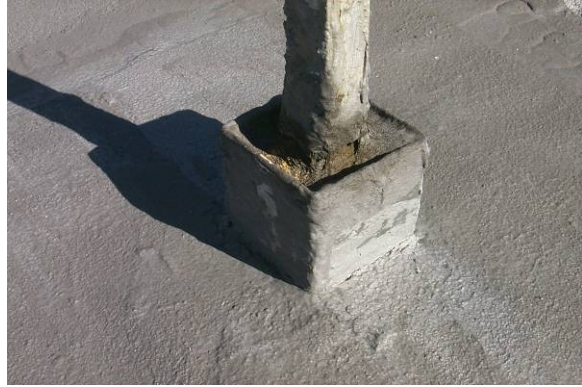
PP-H-2: Sealing material does not fill pitch pan to top of metal rim.
