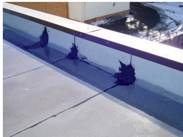
BF-M-4: Flashing has temporary repairs.
