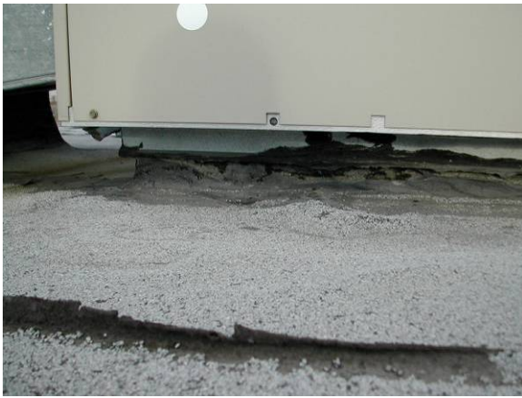
BF-L-2: Top of base flashing is less than 6 in. above the roof surface.
