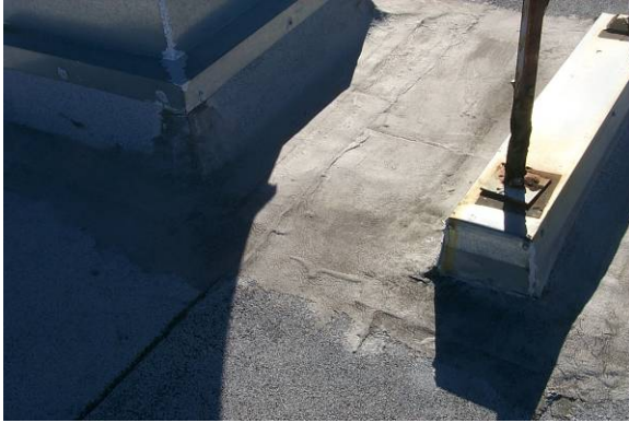
PA-M-1: The materials and workmanship of the patch are not equal to or better than the existing membrane.
