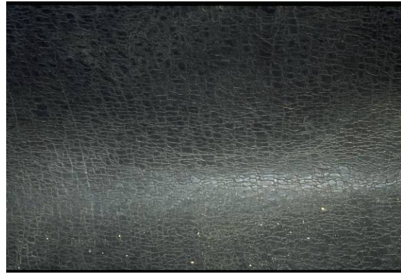
SR-L-3: On smooth liquid applied surfacing, there is evidence of crazing of top surface with hairline cracks (alligatoring).
