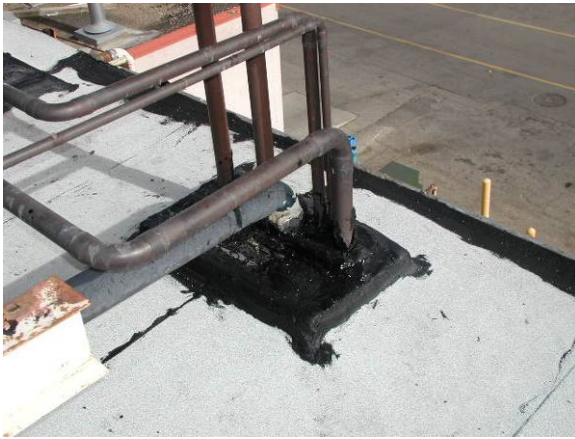
PP-L-1: Pitch pans are rated low severity as a minimum due to the maintenance problems associated with them.
