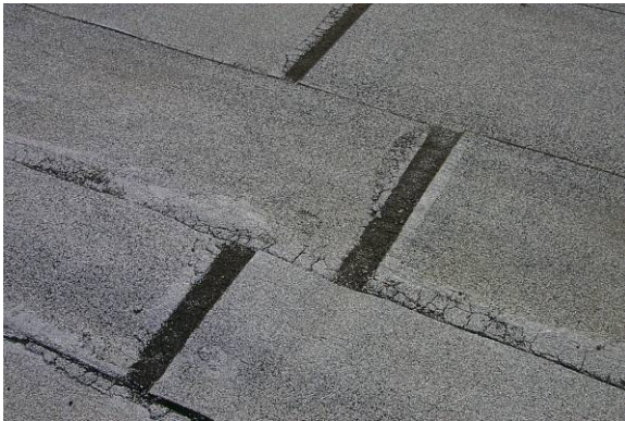
SR-M-2: On mineral surfaced capsheet surfacing, there is loss of granules, exposing the surfacing ply.
