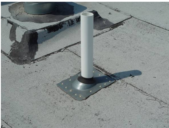
FP-H-1: Flashing sleeve or metal curb has been installed with no stripping plies.
