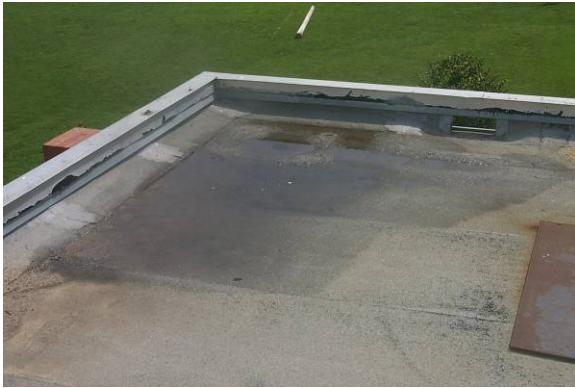
PD-L-1: Ponding is rated low severity due to the maintenance problems associated with it.
