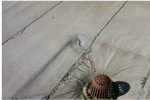
DR-H-1: Holes, splits, or tears in stripping ply caused by deterioration or physical damage.
