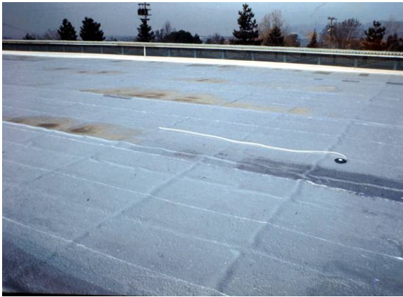
RG-L-1: The ridges are noticeable but the surfacing is still in place and there is no membrane deterioration.
