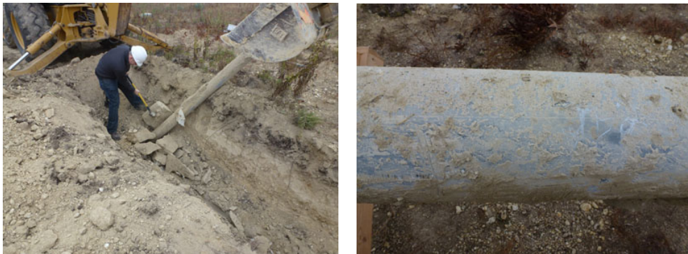
Figure 14. Overall view (left) and close-up view (right) of pipe section JB2 after extraction from soil cement with CP.
