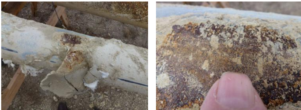
Figure 15. Views of JB2 pipe sections at location of support pads near pipe ends.
