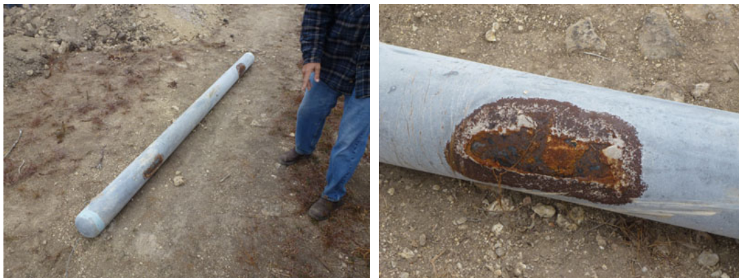
Figure 25. Overall view (left) and close-up view (right) of JB4 after extraction from flowable fill without CP.
