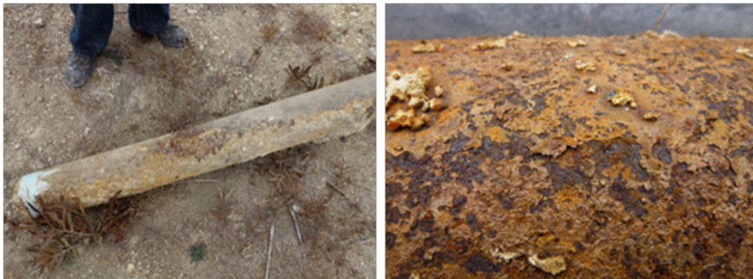
Figure 35. Overall view (left) and close-up view (right) of specimen JB6 after extraction from native soil without CP.
