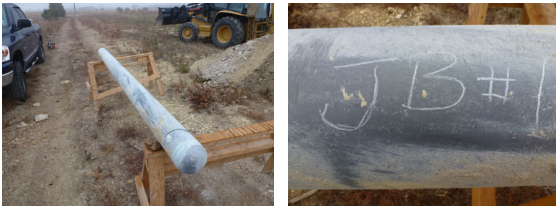
Figure 9. JB1 pipe section after extraction from flowable fill with CP.
