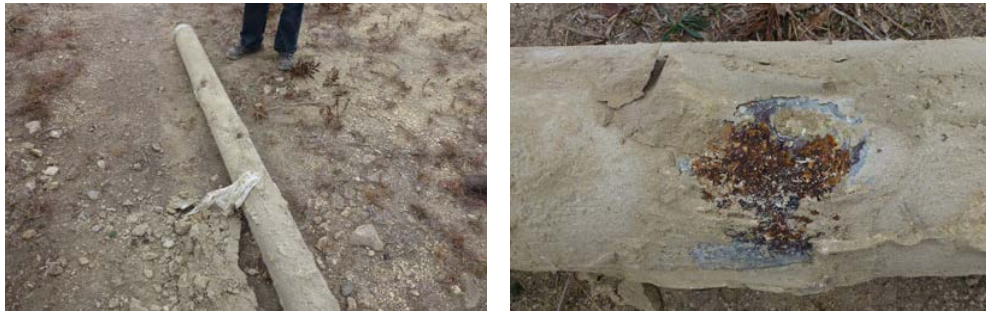
Figure 30. Overall view (left) of JB5 pipe section JB5 after extraction from soil cement without CP..
