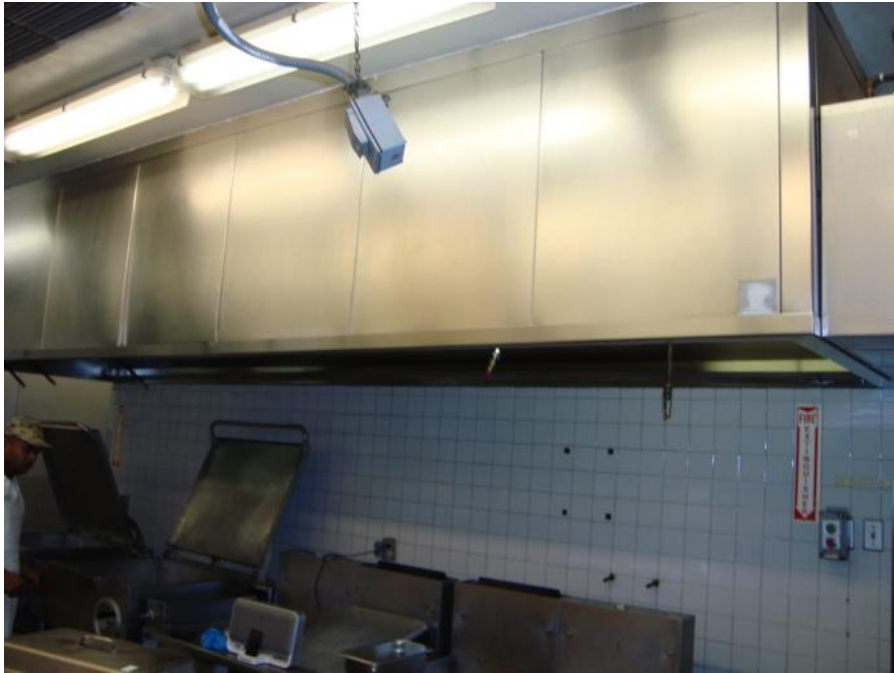
Figure B-2. Kitchen hood that is good candidate for variable air flow.
