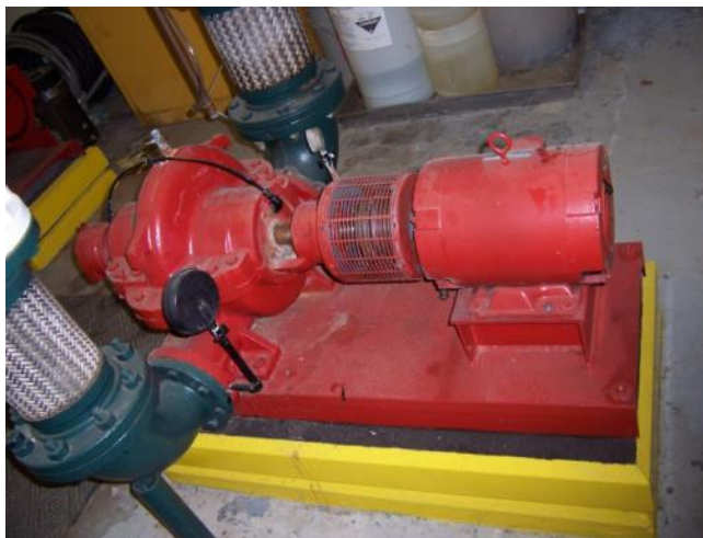
Figure B-3. Typical pump motor.
