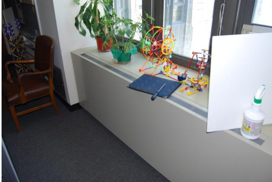
Figure B-1. HW radiator within office of Mahan Hall.
