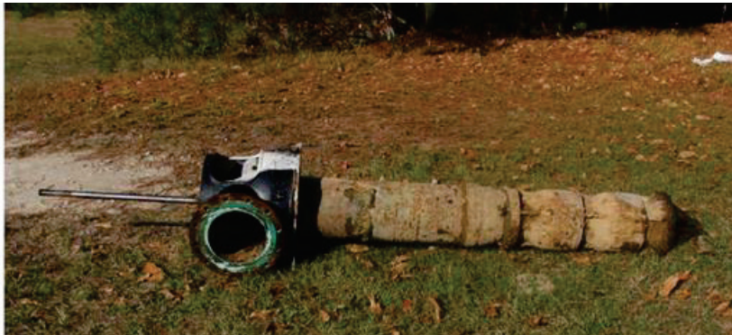
Figure 6. Condition of pump housing 3, after removal from sump.
