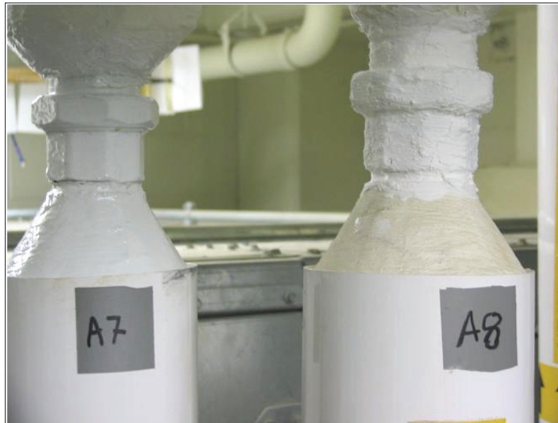
Figure 3. Union joints in Mechanical Room A, coated with Sherwin-Williams Corothane System (A7, on left) and TC Ceramic (A8, on right).
