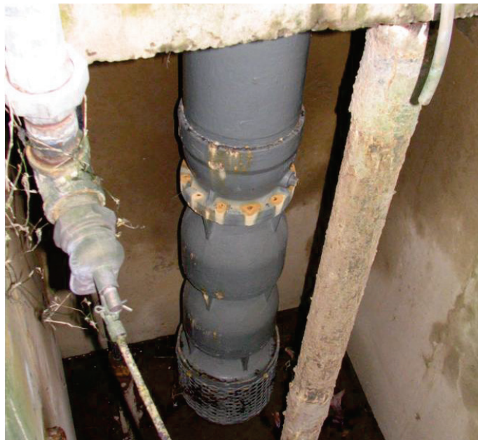
Figure 26. Pump 3 (Macropoxy primer-topcoat), 12 months.
