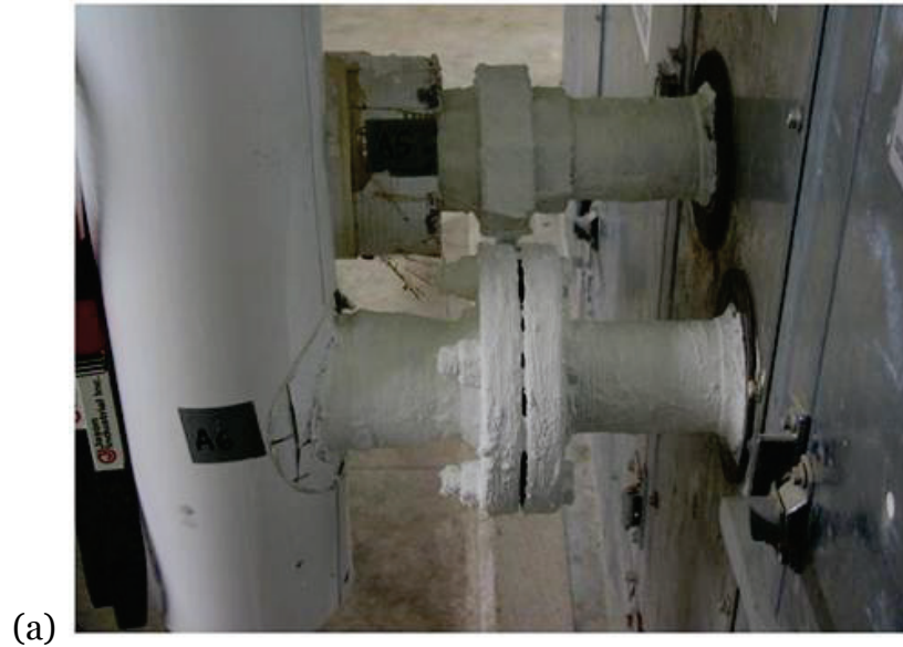
Figure 17. Two cold water line fittings coated with TC Ceramic in Mechanical Room A exposures at 3 months (a), 6 months (b), 9 months (c), 12 months (d), and 30 months (e).
