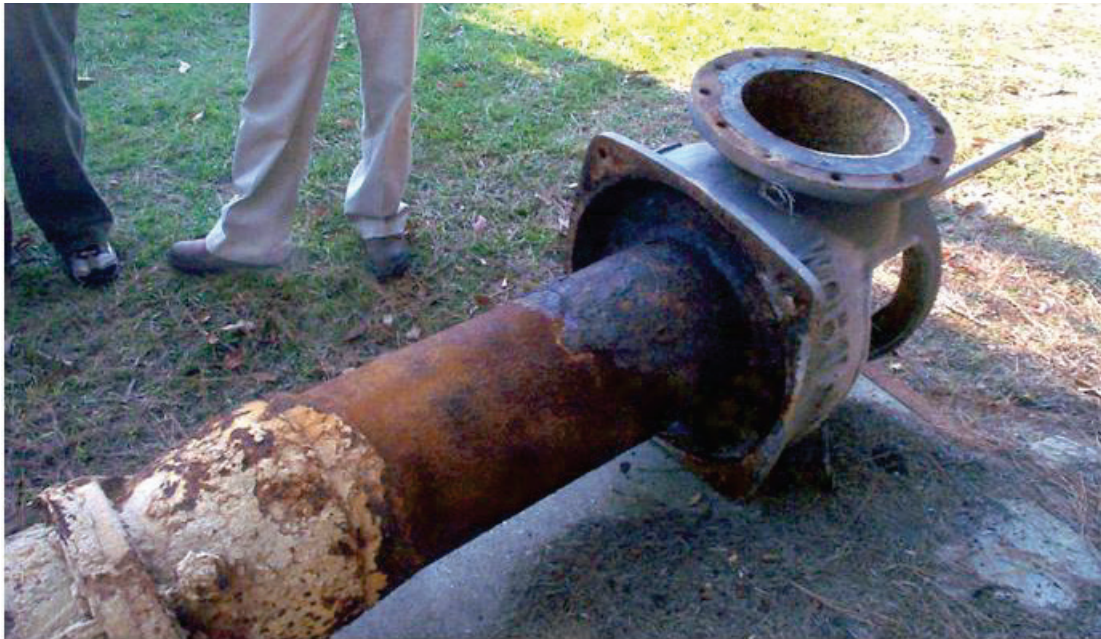
Figure A2. Corroding pumps bodies at central heating plant at Fort Bragg.
