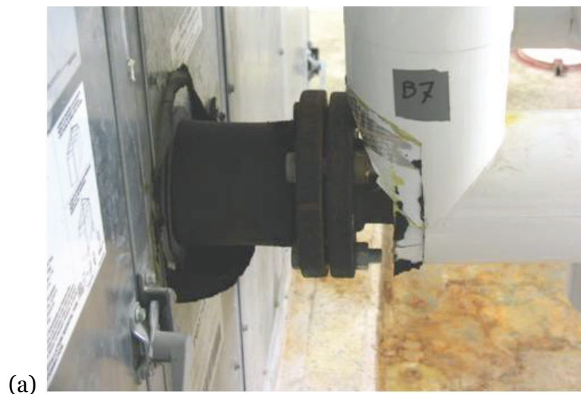
Figure 21. Cold water line fitting in Mechanical Room B exposures at 3 months (a), 6 months (b), 9 months (c), 12 months (d), and 30 months (e).
