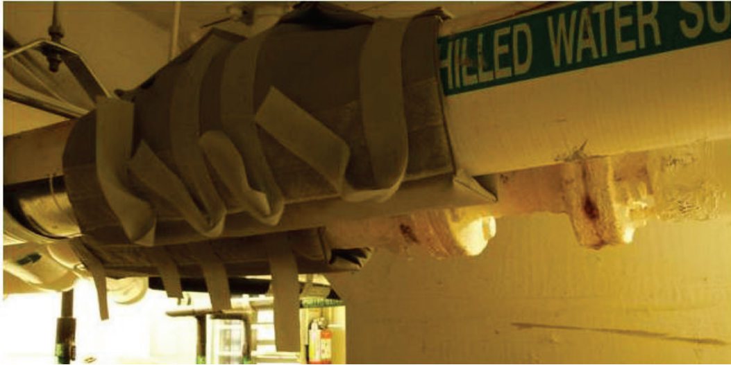
Figure 22. SpeedWrap on fittings, Mechanical Room A, 9 months exposure.
