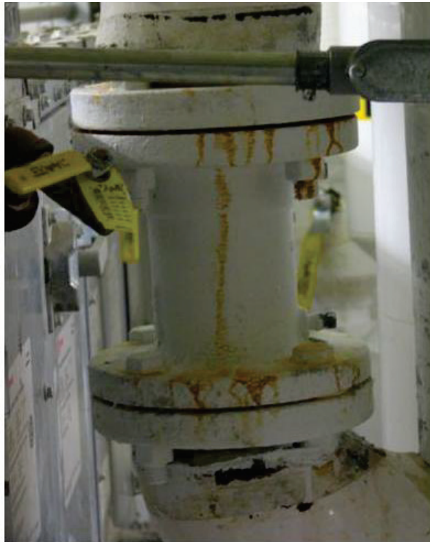
Figure 23. Condition of fitting after removal of SpeedWrap, Mechanical Room A, 12 months exposure.
