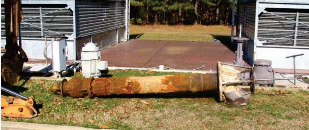
Figure 8. Condition of pump housing 5 after removal from sump.
