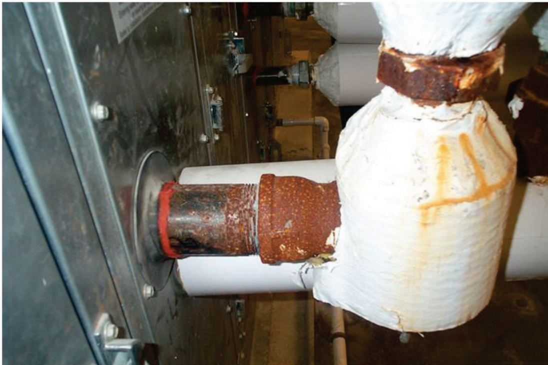
Figure A1. Corroding steel utility piping in high-humidity mechanical room at Fort Bragg.
