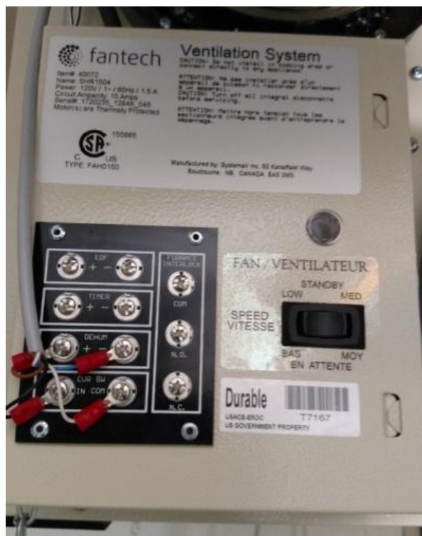
Figure 5-6. Fantech SHR 1504 HRV electrical panel.
