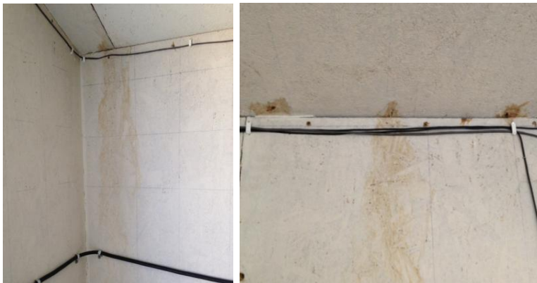
Figure 6-5. Staining on walls from water infiltration.
