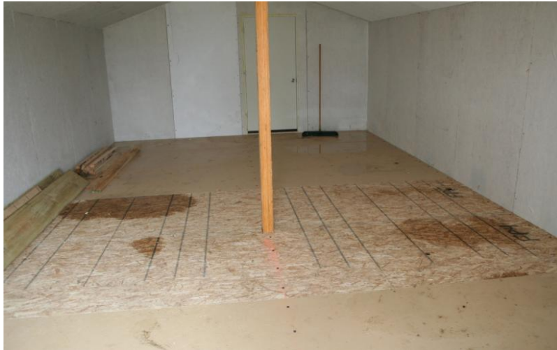
Figure 6-1. Standing water in SIP hut (14 March 2014).
