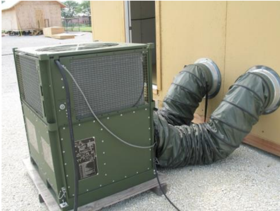
Figure 4-22. IECU serving the SIP hut and the flexible ducts used as supply and return ducts.
