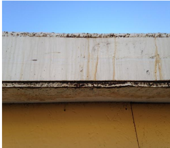
Figure 6-7. Deterioration of the edges of the SIP OSB panels on roof eave fascia.
